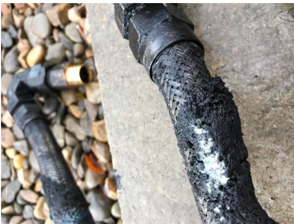
Close up of gas connector, source of fire.
