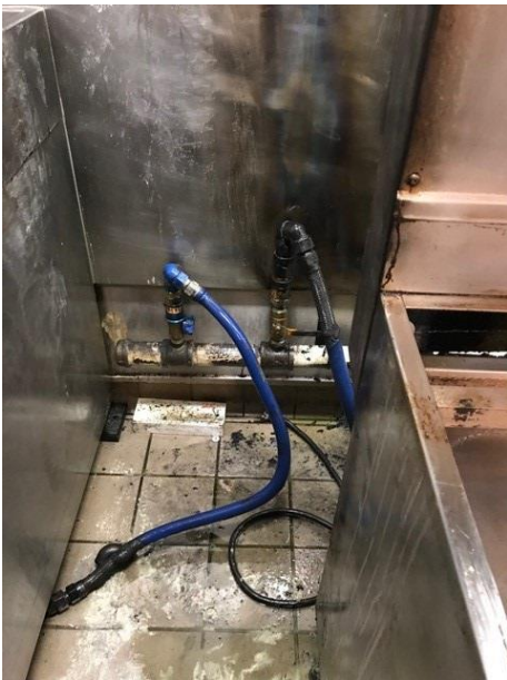
Fire damaged area with gas connectors to appliances.
