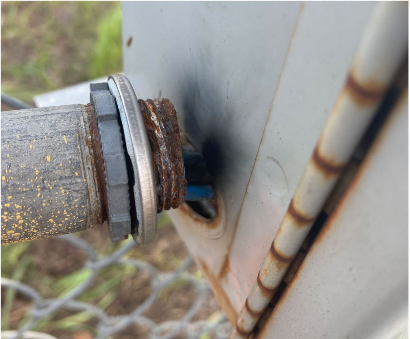
Photo 1 - Conductors in contact with enclosure
