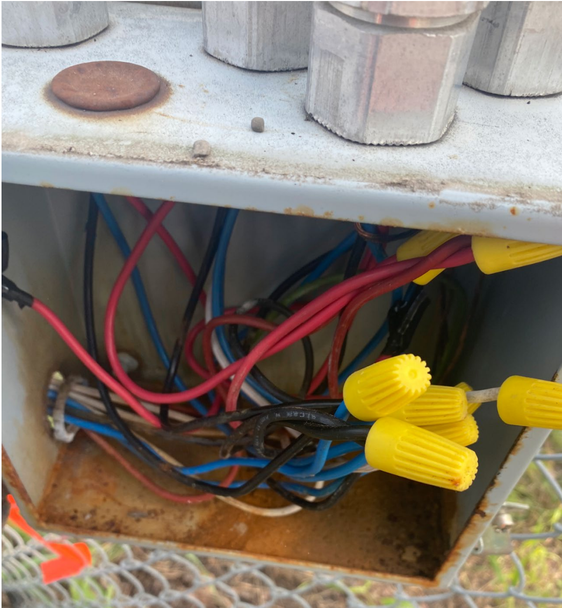
Photo 3 - Conductors in splice box
