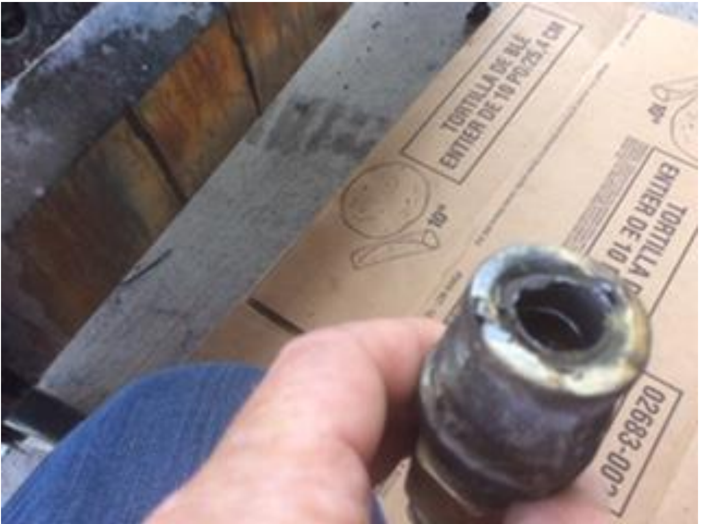
Broken Connection Point
