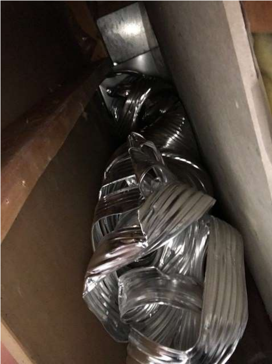
Figure 3 View of fireplace venting above fireplace extending through 2nd floor to roof termination
