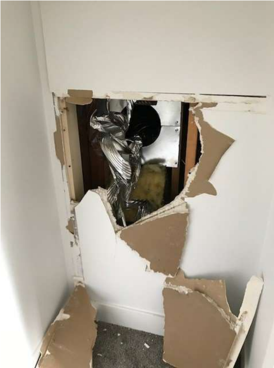
Figure 2 - View of gas fireplace venting above fireplace 10-15' away
