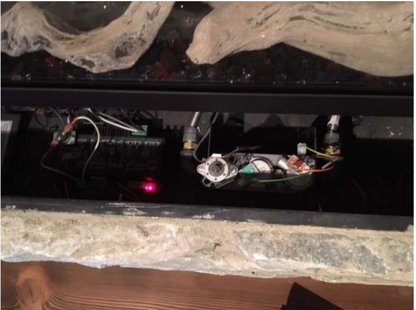
This is a picture of the gas safety valve that failed
