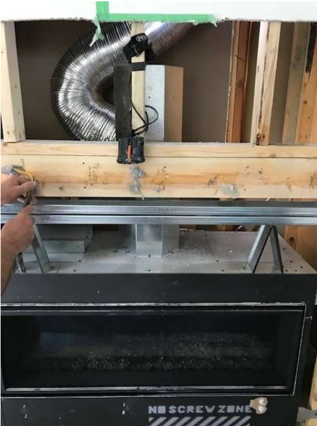
Figure 1 - Front view of fireplace with drywall removed
