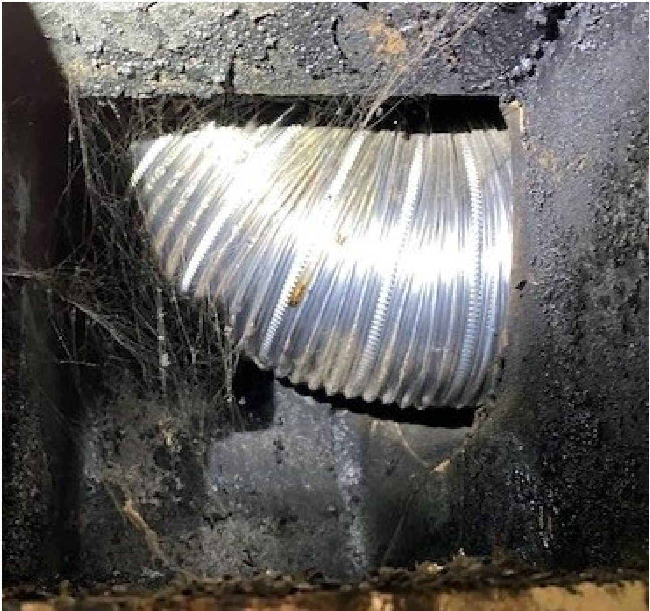
Photo 9 - Stainless steel chimney liner connected to the fireplace pulled through the existing masonry chimney. The installation manual does not describe using a chimney liner as part of the installation.
