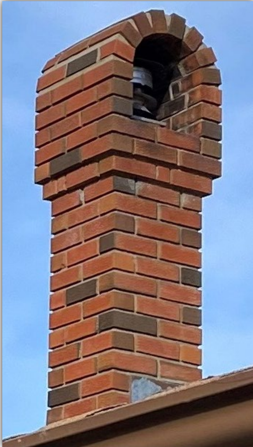
Photo 10 - The top arch of the existing masonry chimney is a restriction to the vent cap for the fireplace venting.
