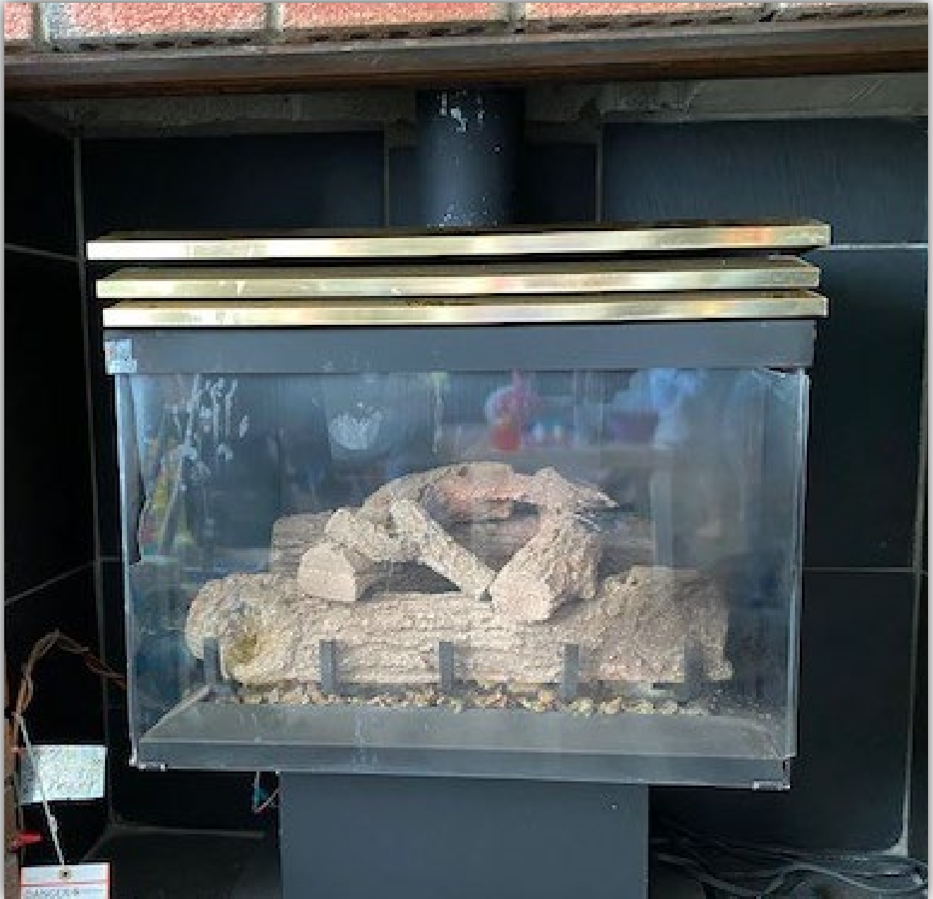
Photo 2 - The fireplace after the incident. A gas utility technician had removed the aluminum trim on the corners of the glass exposing the holes in the glass on the sides.
