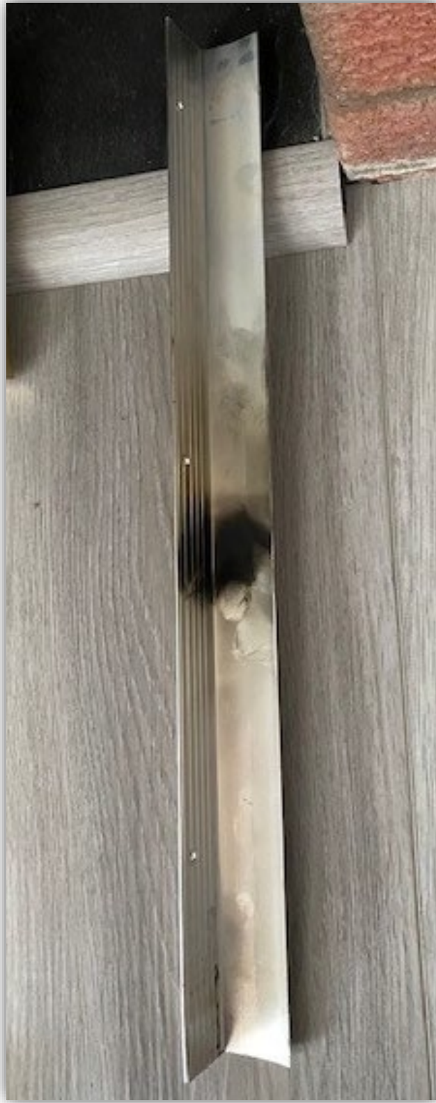
Photo 8 - The back of the right-side aluminum trim piece showing discoloration from products of combustion from the damaged glass.
