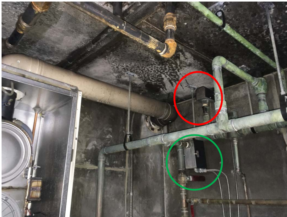
Room upper right corner near boiler #2, low water cut off (green), and above it the flow switch (red)
