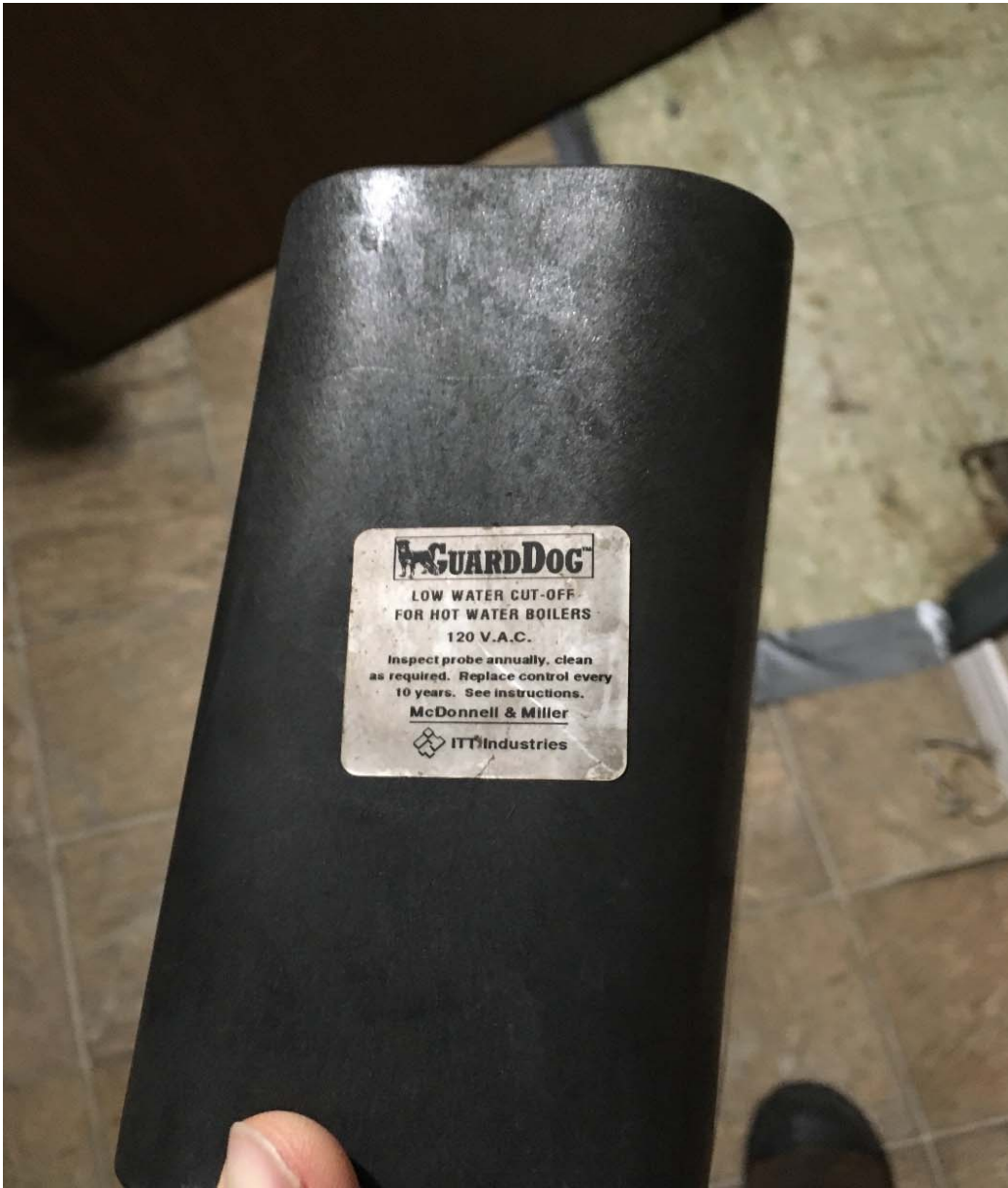
Low water cut-out cover (removed by contractor)
