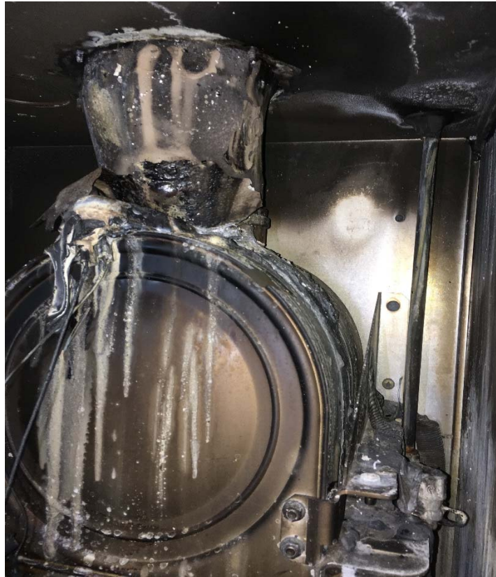
Above – Boiler #1 exhaust fan housing and melted vent
