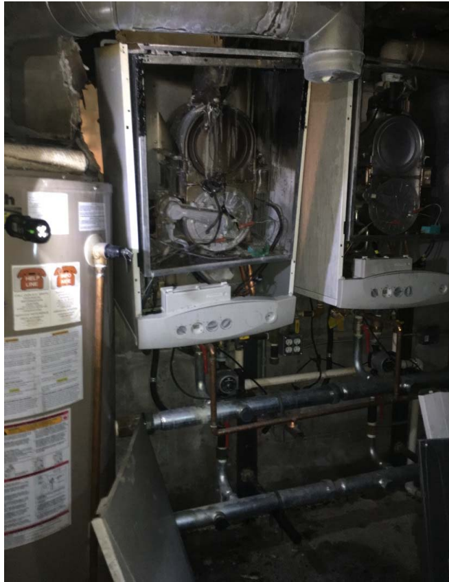
Boiler #1 on left (prior to removal by contractor)
