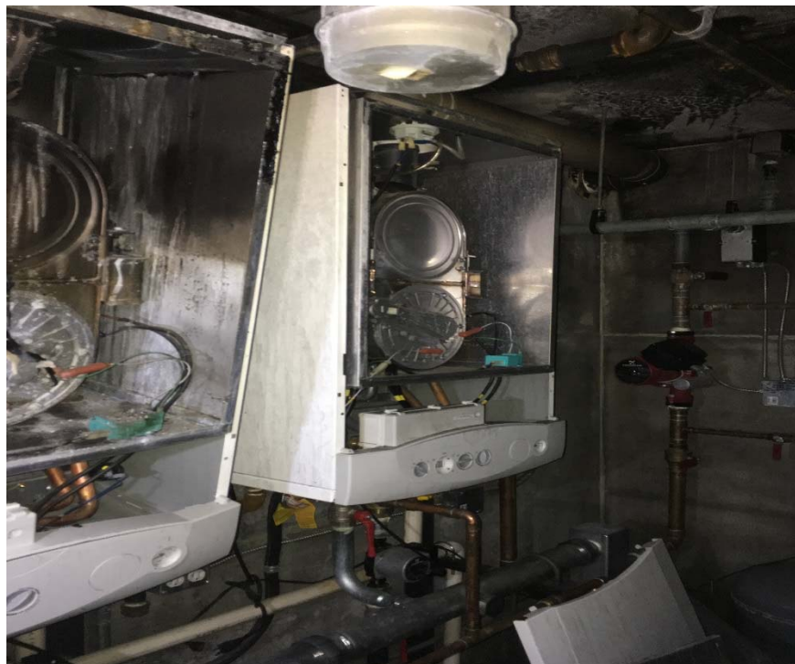
Boiler overview - Boiler #1 on left
