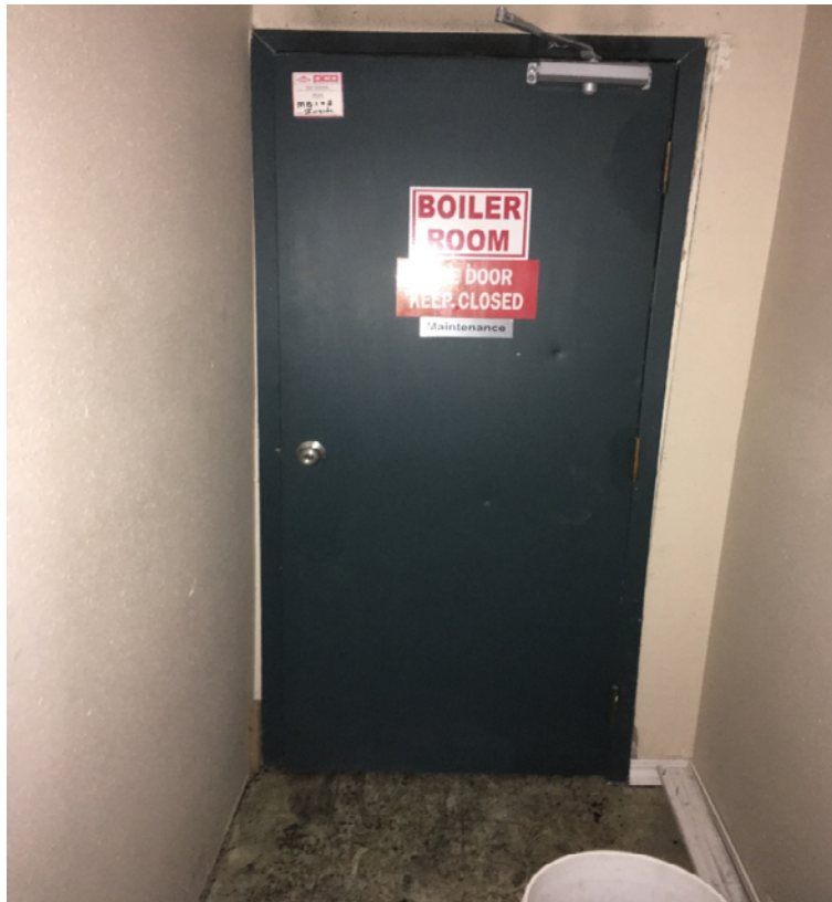
Boiler room door closed – notice soot above door frame
