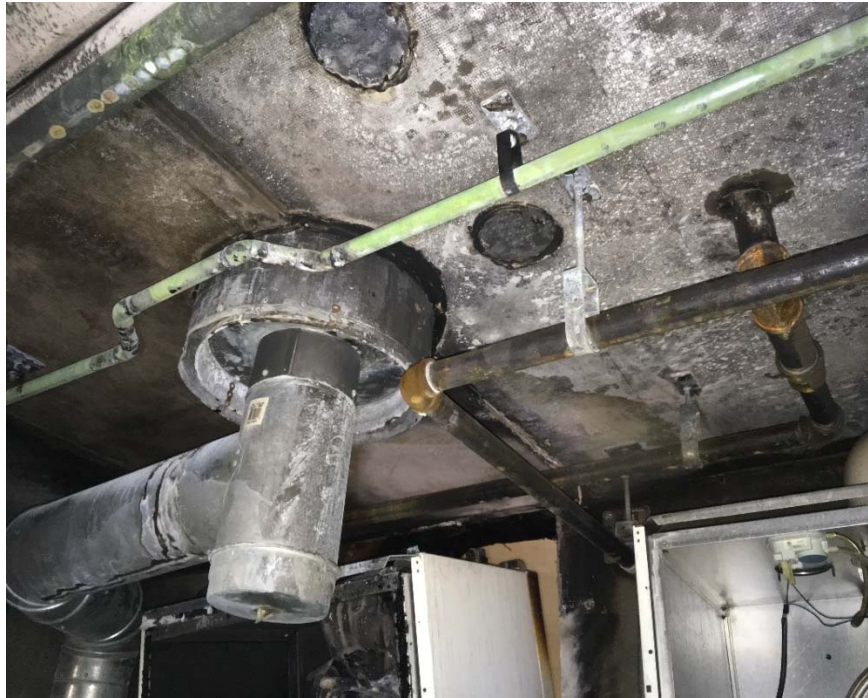
Photo above shows boiler room ceiling damaged by fire
