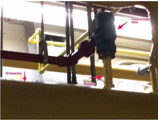
Photo 1: View of pressure relief valve and nipple assembly.
