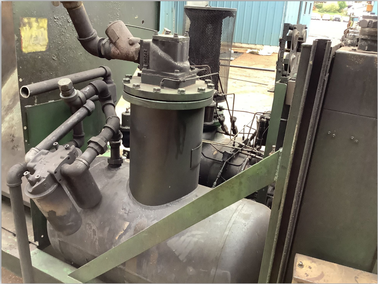
Image 5 - Air tank and cooling oil, heat exchange piping.
