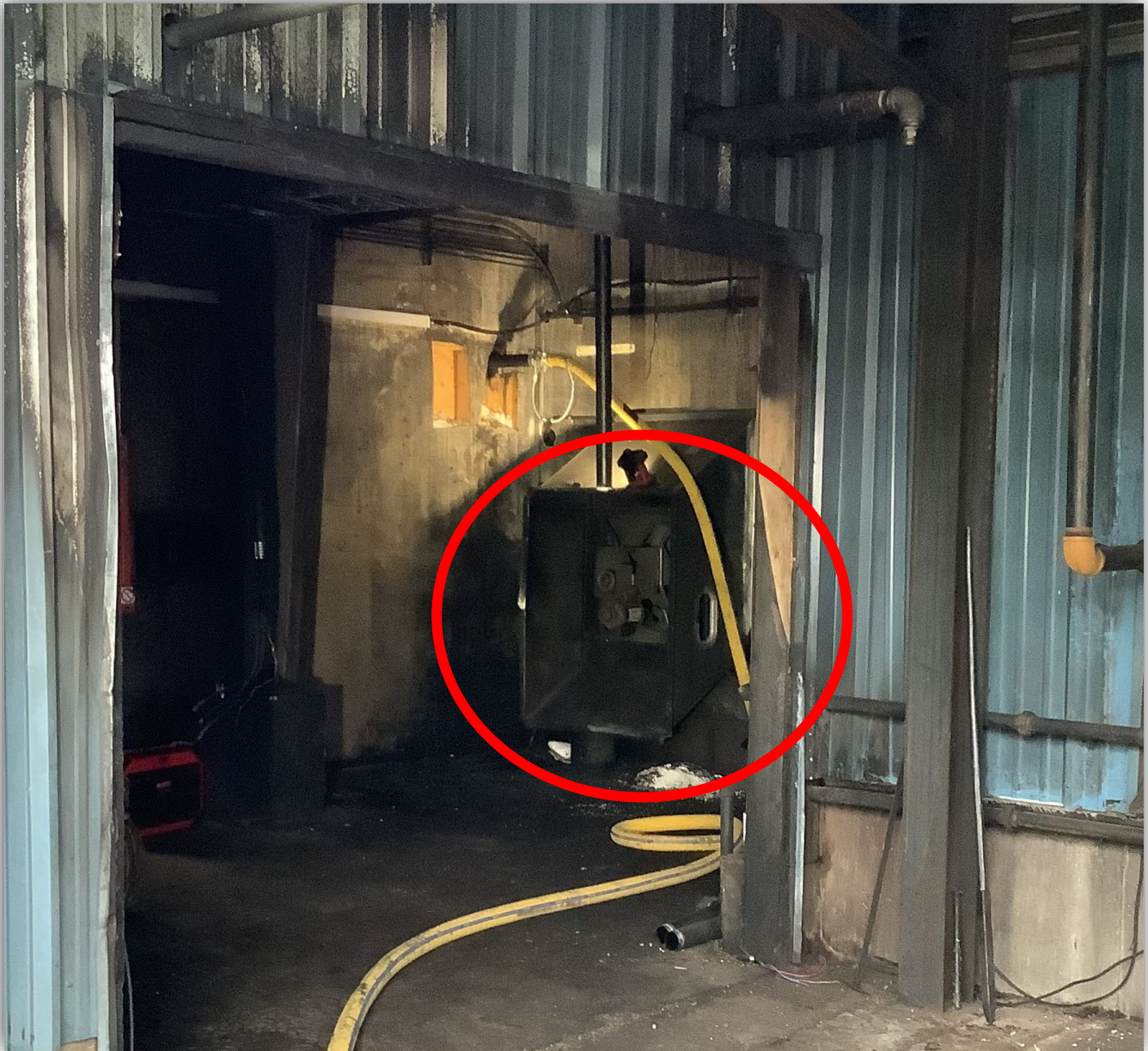
Image 1 - Air compressor location.
