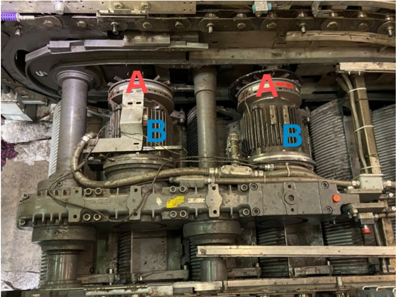
Image 4 - Escalator #3 dual motor drive assembly installed at top of escalator.
