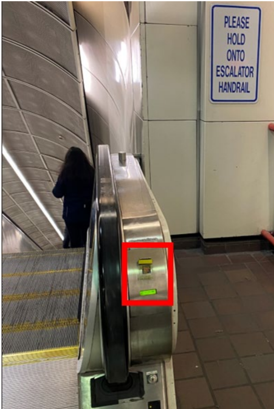
Image 2 – Top of escalator #3. [RED] Emergency stop button.
