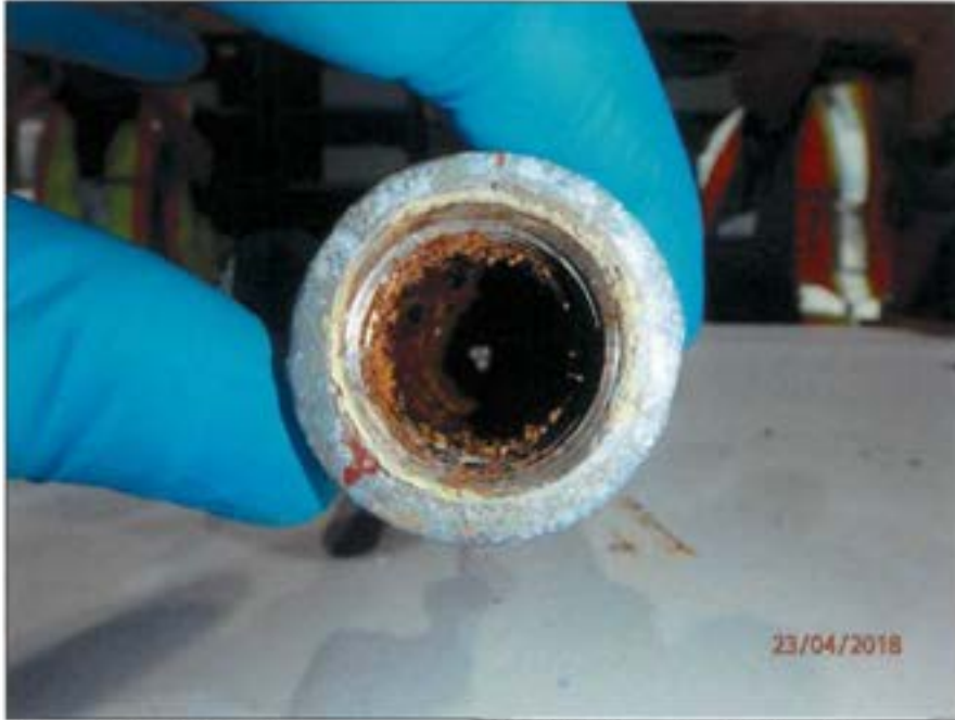
Figure 14 Relatively minor corrosion debris in Tee end of Valve A-2.
