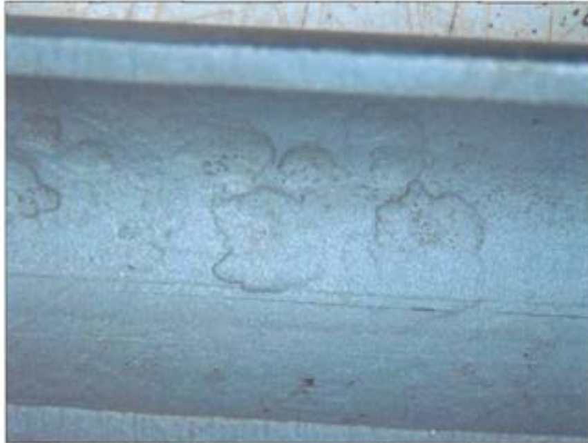
Figure 154 Corrosion damage on row 14 - tube 2 (bottom) after aluminum oxide blasting.
