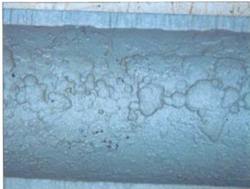
Figure 135 Corrosion damage on row 4 - tube 10 (top) after aluminum oxide blasting.
