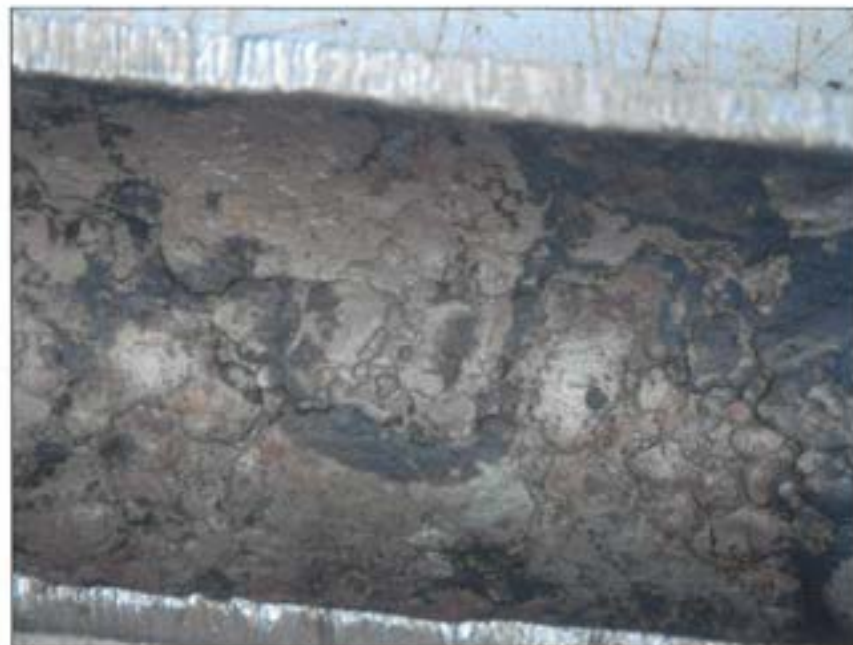
Figure 147 Corrosion damage on row 11 - tube 1 (top) after plastic bead blasting.
