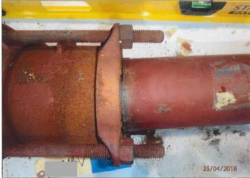
Figure 87 Misalignment with coupling after event. Bolt extensions are roughly equal.
