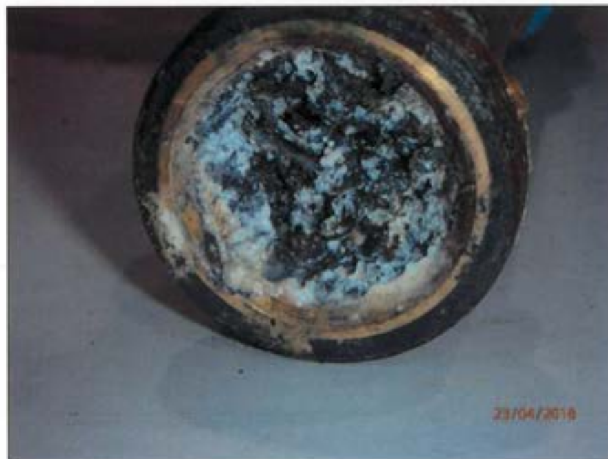
Figure 2 Plugged end fitting on top end of Valve X.
