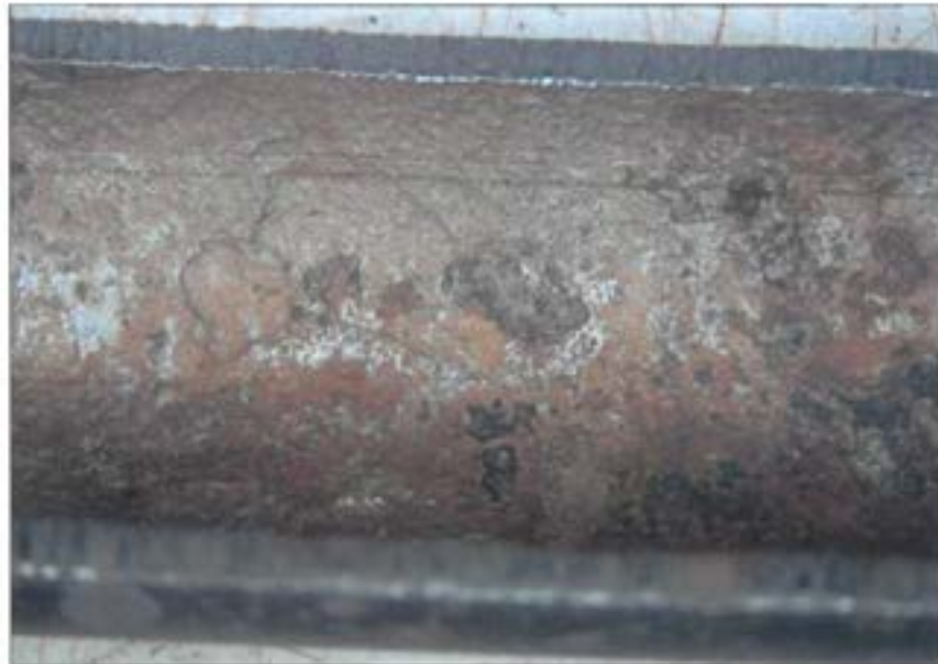
Figure 149 Corrosion damage on row 11 - tube 10 (bottom) after plastic bead blasting.
