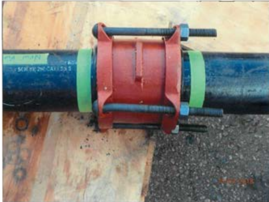
Figure 69 Slipped exemplar [redacted] coupling at 24 psi.
