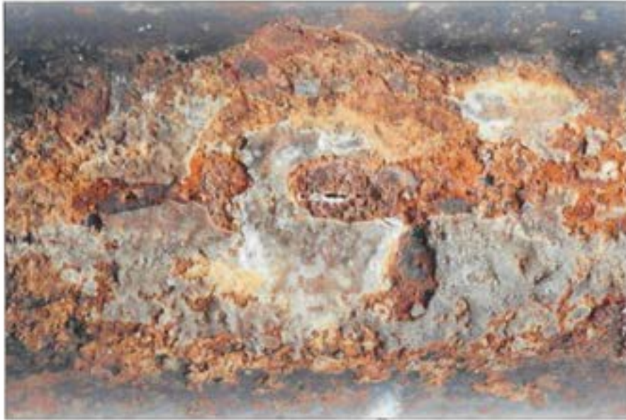
Figure 115 Close-up view of leaking defect on row 2 – tube 3 showing white deposits.
