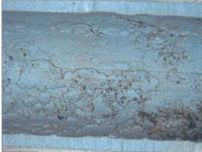
Figure 144. Corrosion damage on row 7 - tube 13 (top) after aluminum oxide blasting.
