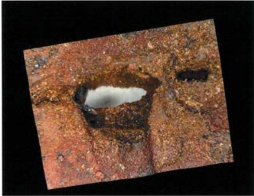
Figure 125 Oblique view of leaking pit showing corrosion attack through cross section.
