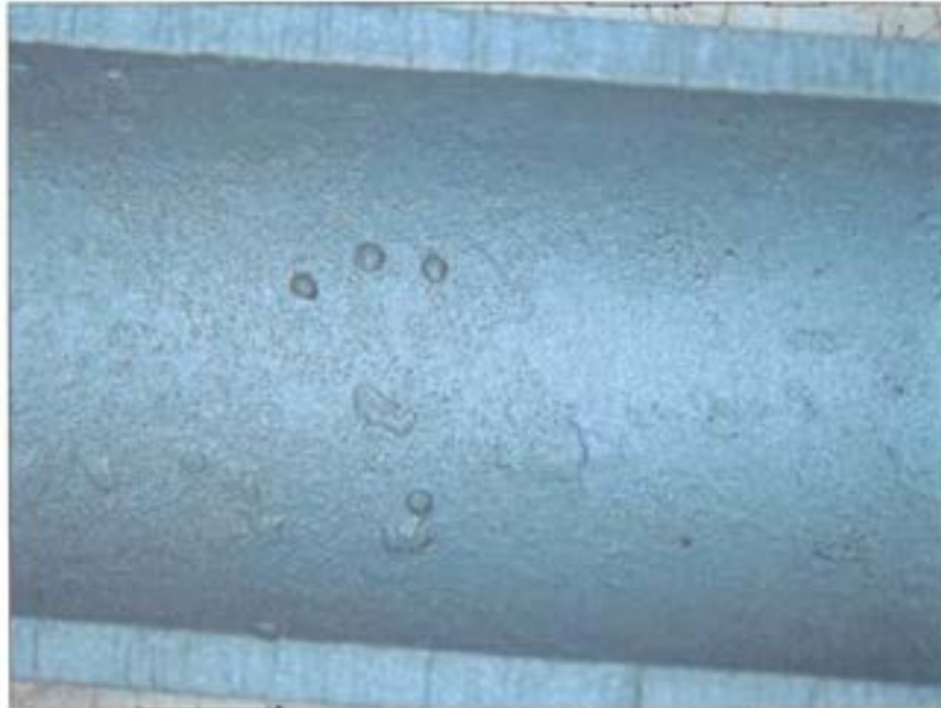
Figure 152 Corrosion damage on row 11 - tube 10 (top) after aluminum oxide blasting.
