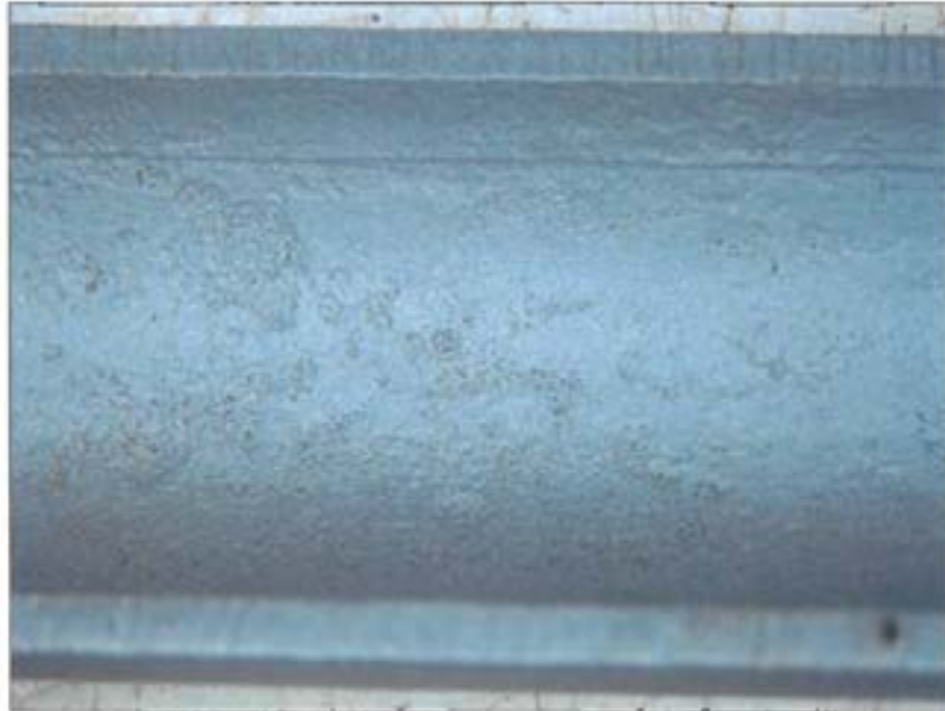
Figure 150 Corrosion damage on row 11 - tube 10 (bottom) after aluminum oxide blasting.
