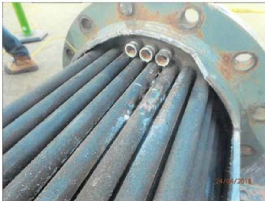
Figure 104 Row 1 tubes removed for access to leak area. Note white material has begun to be dissolved by a process of deliquescence.
