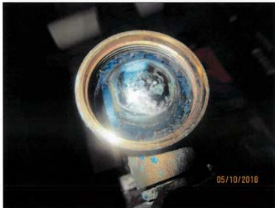
Figure 23 Corrosion debris surrounding ball in partially cocked valve Z.
