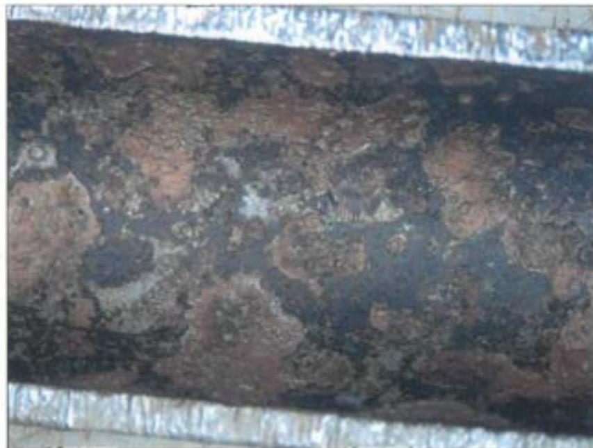
Figure 151 Corrosion damage on row 11 - tube 10 (top) after plastic bead blasting.
