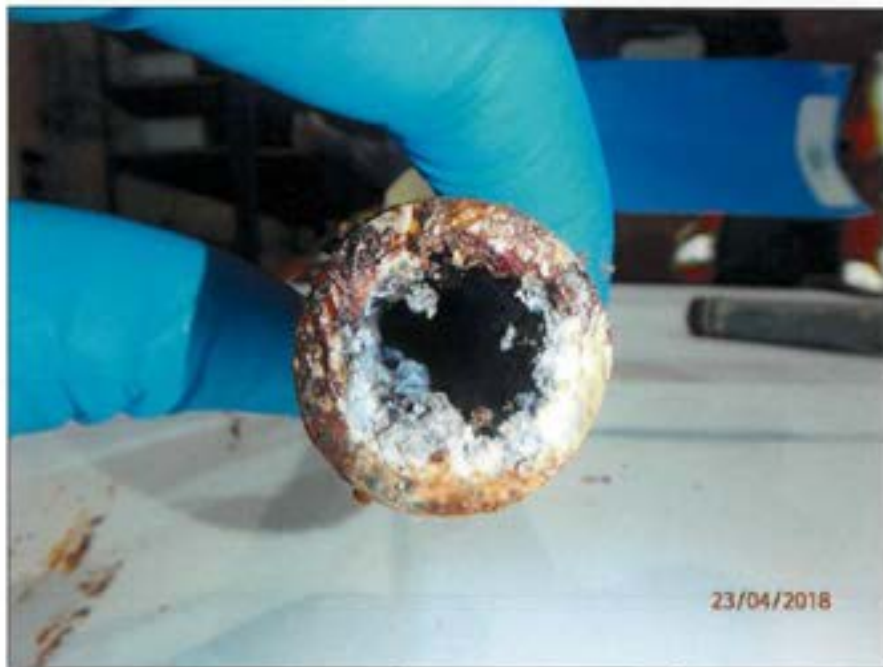
Figure 19 White deposit partially plugging Valve Z. White material is calcium chloride.
