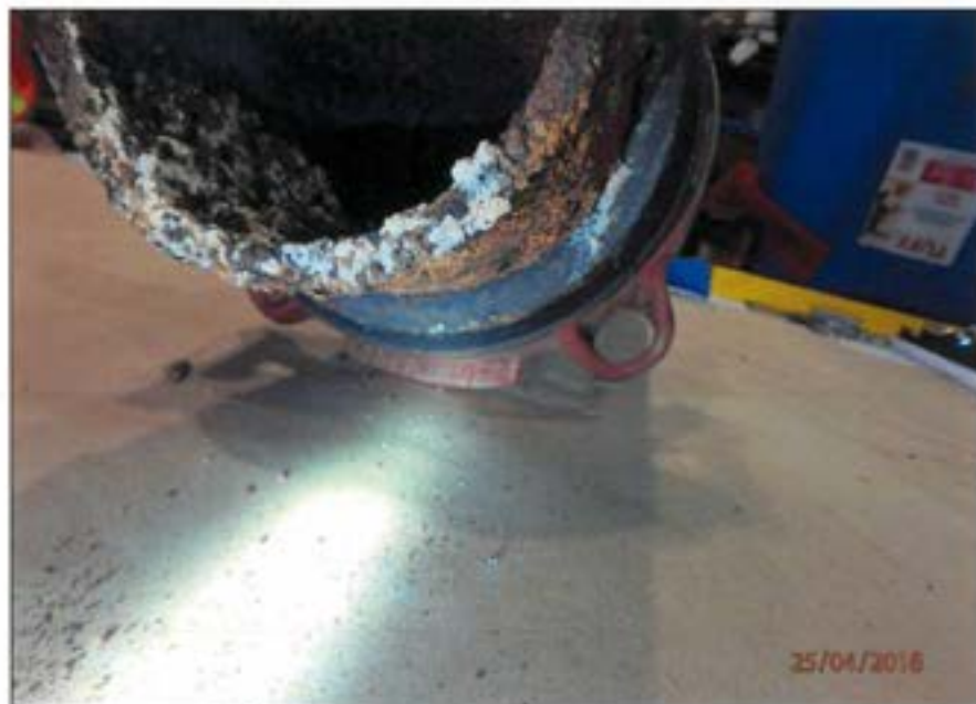
Figure 74 Typical white salts found within the pipe attached to horizontal [redacted] coupling.
