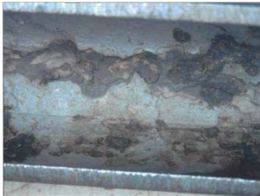
Figure 153 Corrosion damage on row 14 - tube 2 (bottom) after plastic bead blasting.
