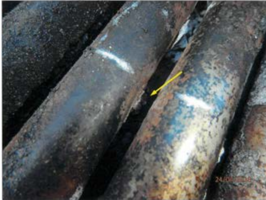
Figure 105 Location of leaking defect on Row 2 – Tube 3.
