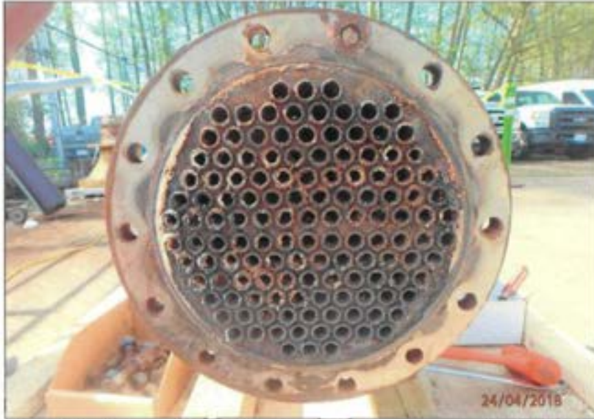
Figure 97 Return tubesheet side of chiller. Tubes are corroded and partially filled with debris.
