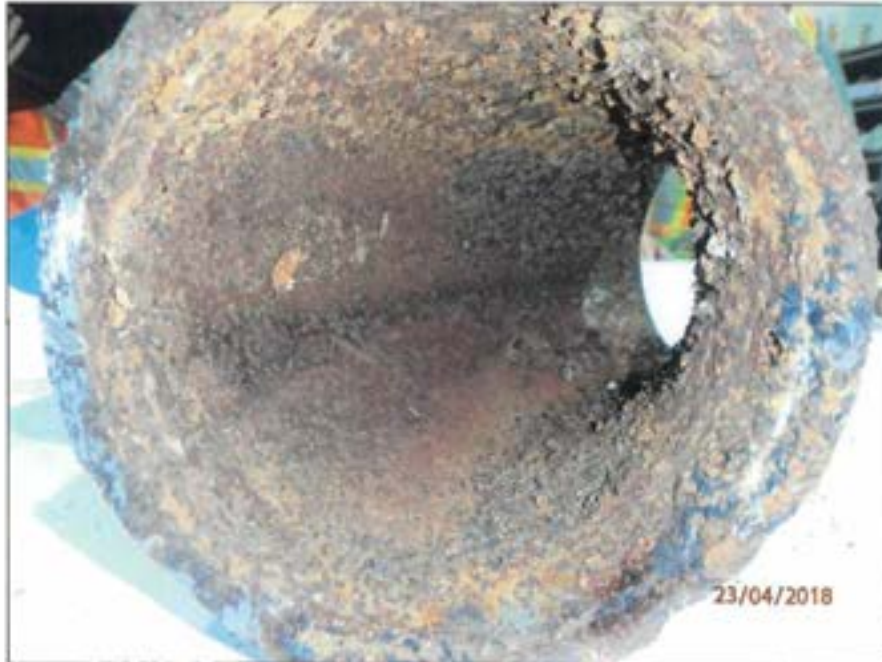
Figure 24 Inside of Elbow A-10 showing severe corrosion damage.
