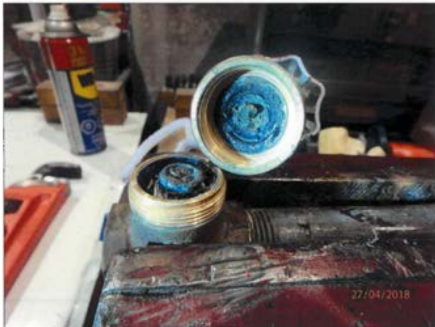
Figure 33 Gate Valve Y internal components. Stem would not engage and appeared fractured.
