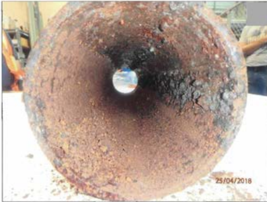
Figure 79 Severe corrosion in horizontal brine pipe that detached from coupling.
