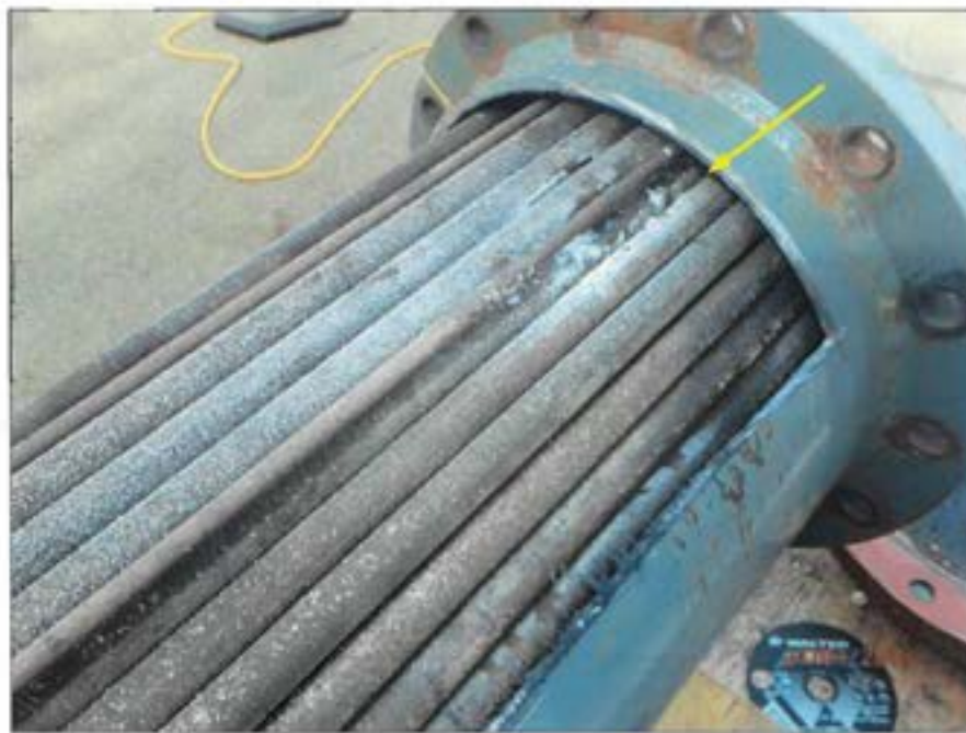
Figure 100 General area of leak found by pressurized argon testing.
