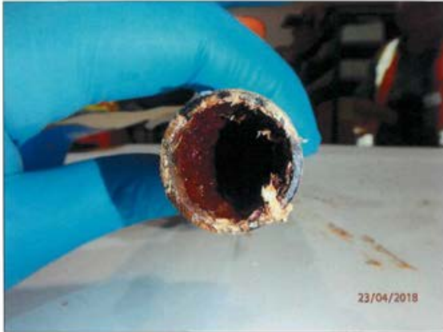
Figure 10 Nipple end of Valve A-6 piping showing internal deposits.
