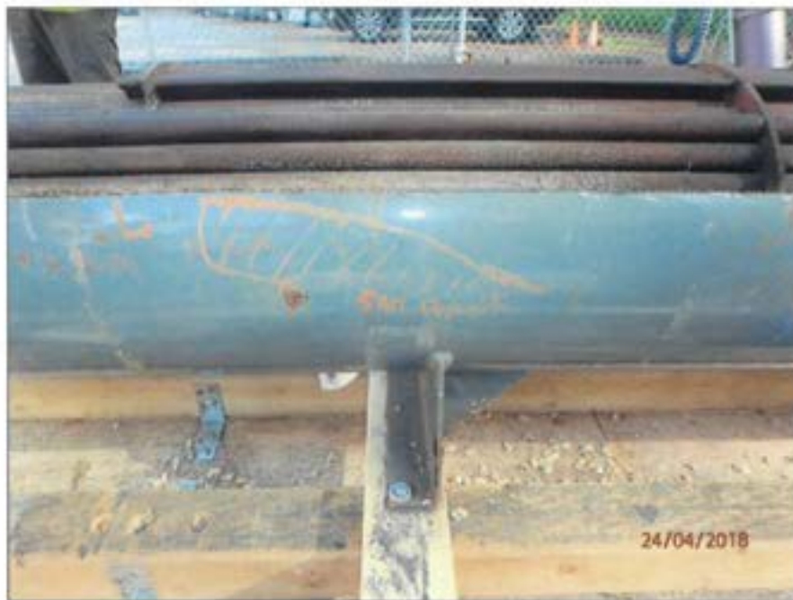
Figure 106 Area where white material was sprayed onto the tank wall and tubes (orange paint).
