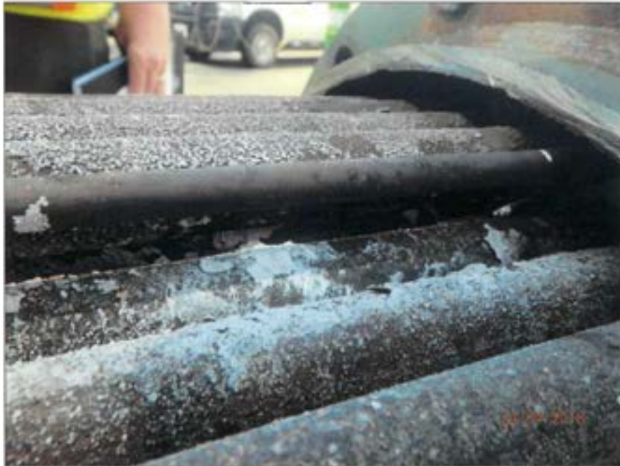
Figure 101 Closer view of leak area on row 2 – tube 3. Note relatively large amounts of white material deposited on surfaces.
