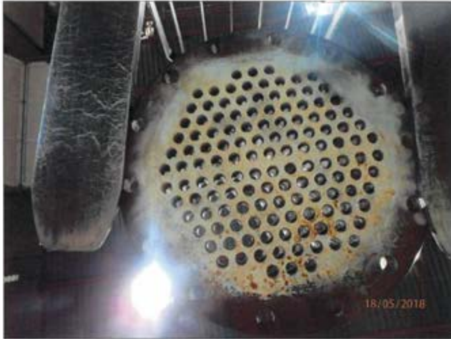
Figure 109 No sign of leaks after 18 hours of dwell time.
