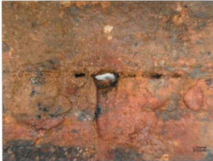
Figure 123 Closer view of pit line in row 2 – tube 3 at leak.
