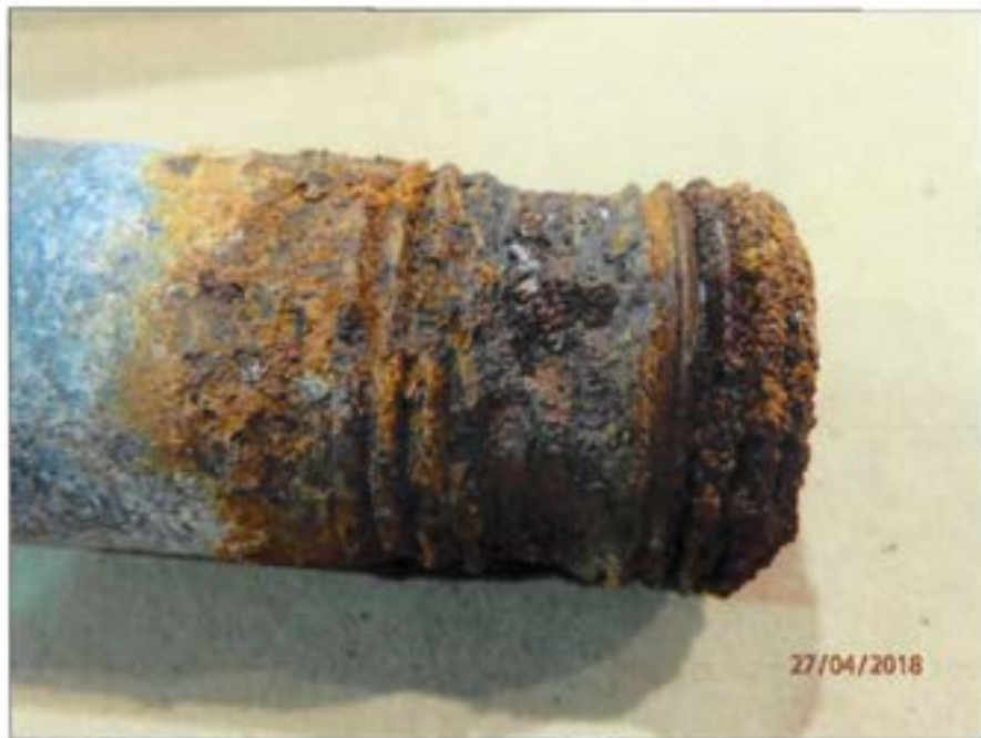
Figure 31 Corroded nipple threads on Valve Y nipple.
