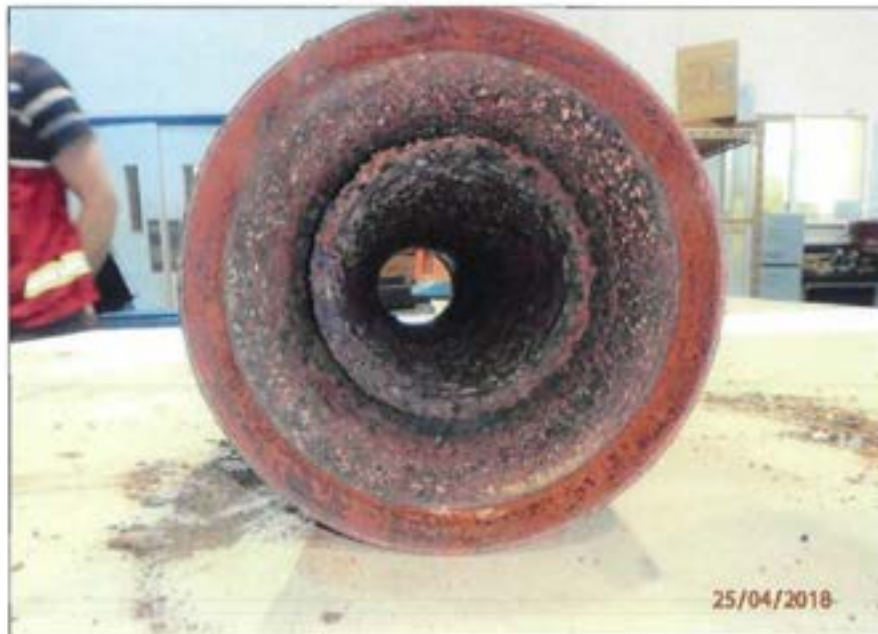
Figure 88 Severe corrosion damage on interior surface of vertical coupling.
