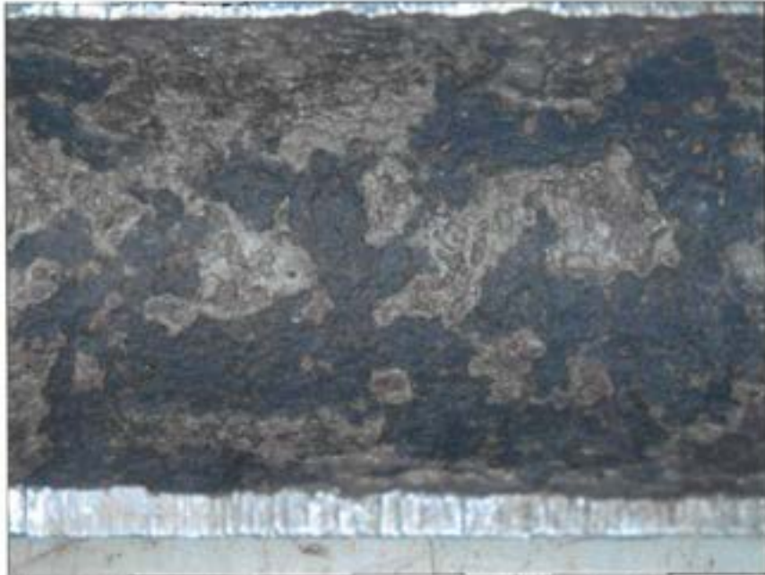
Figure 134 Corrosion damage on row 4 - tube 10 (top) after plastic bead blasting.
