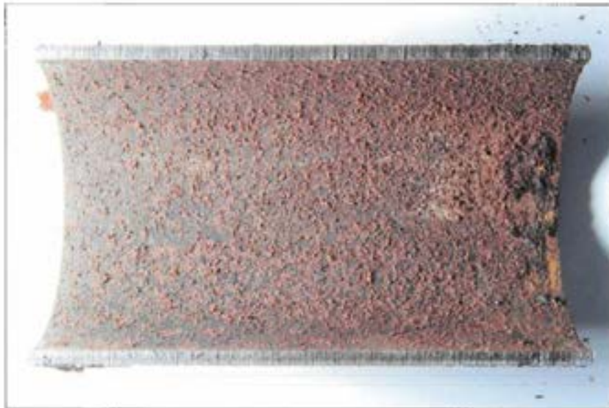
Figure 80 Corrosion found in horizontal brine pipe separated from coupling.
