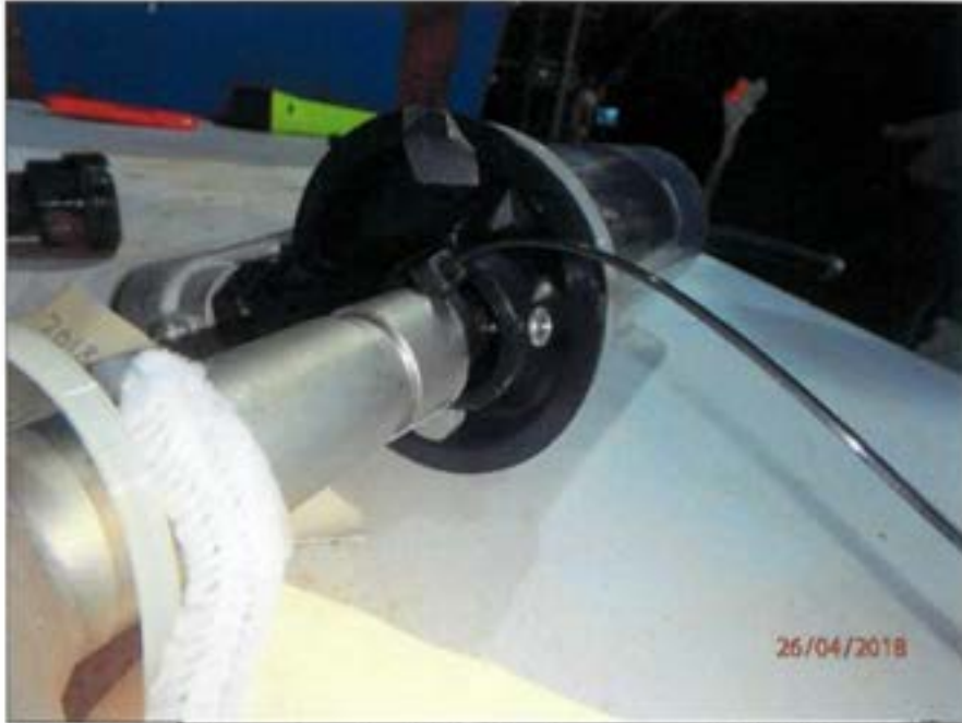
Figure 62 Zap strap found on LC2. Operation was restricted by this strap.
