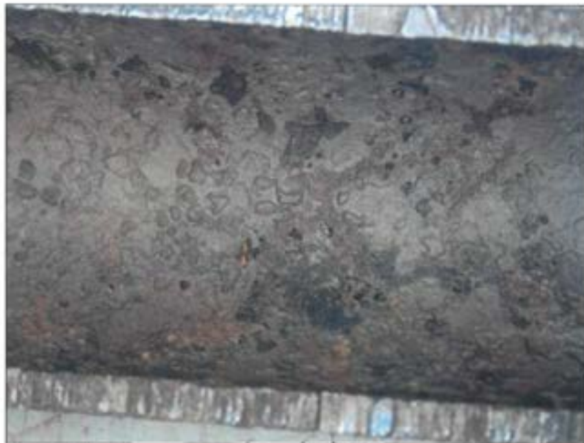
Figure 145. Corrosion damage on row 11 - tube 1 (bottom) after plastic bead blasting.
