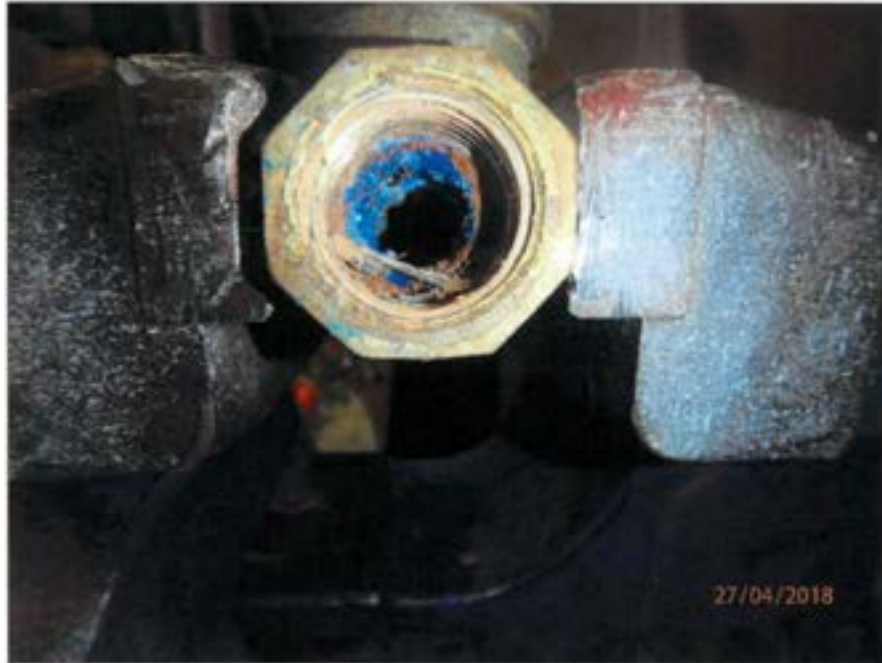
Figure 34 Blue corrosion product in Valve Y body. Body is partially plugged.
