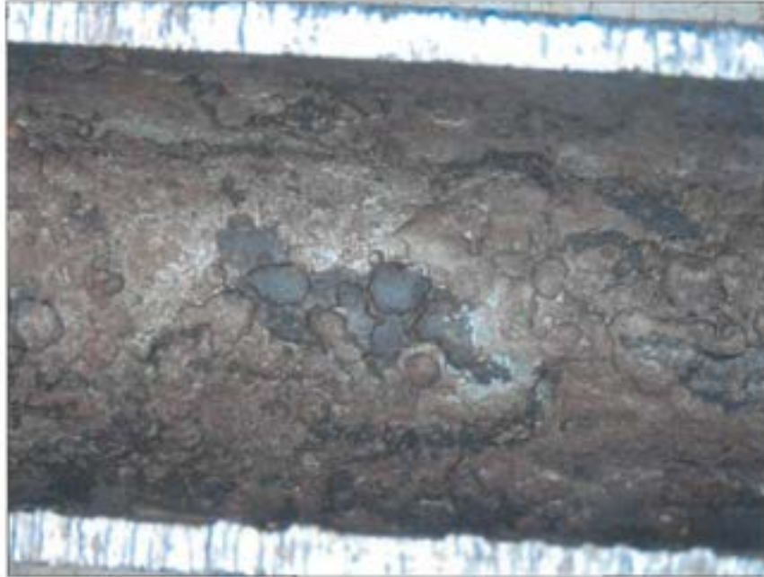
Figure 140 Corrosion damage on row 7 - tube 13 (bottom) after plastic bead blasting.
