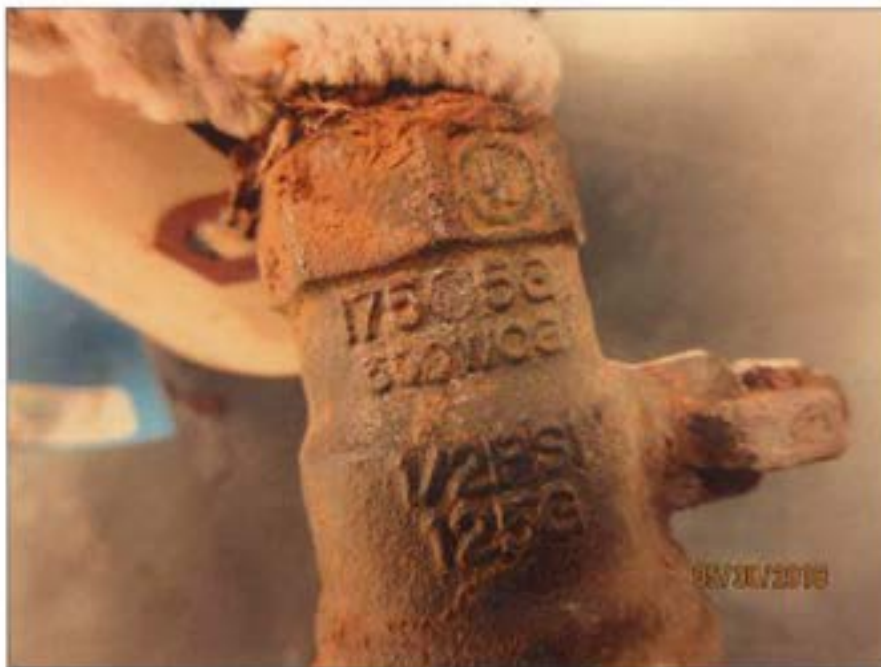
Figure 27 Markings on Valve A-10.
