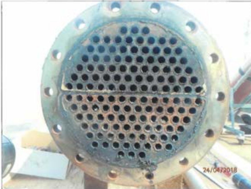
Figure 95 Inlet/outlet tubesheet on return side of chiller.
