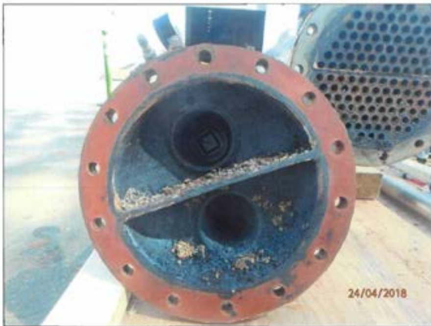
Figure 96 Inlet/outlet head removed from chiller.
