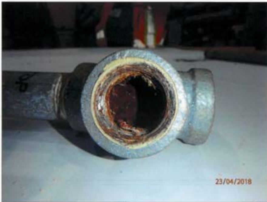
Figure 15 Relatively minor corrosion debris in second Tee end of Valve A-2.
