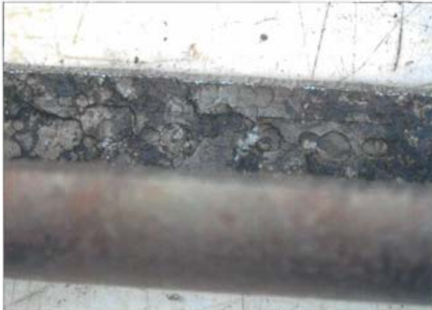
Figure 132 Corrosion damage on row 4 - tube 10 (bottom) after plastic bead blasting.
