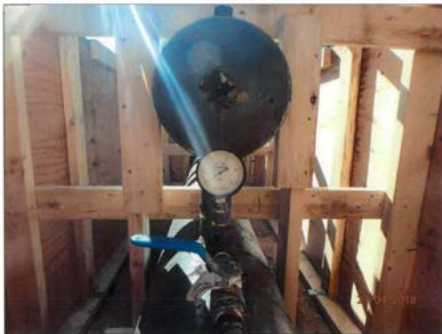
Figure 94 Positive pressure on brine side of chiller.
