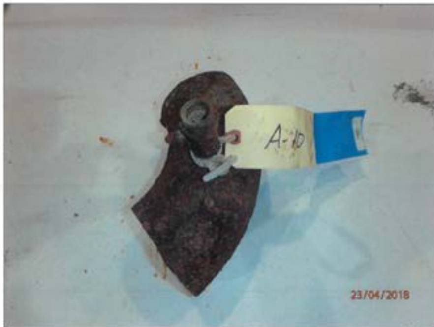
Figure 25 Valve A-10 on rusty elbow. Ball appears corroded and slightly worn.
