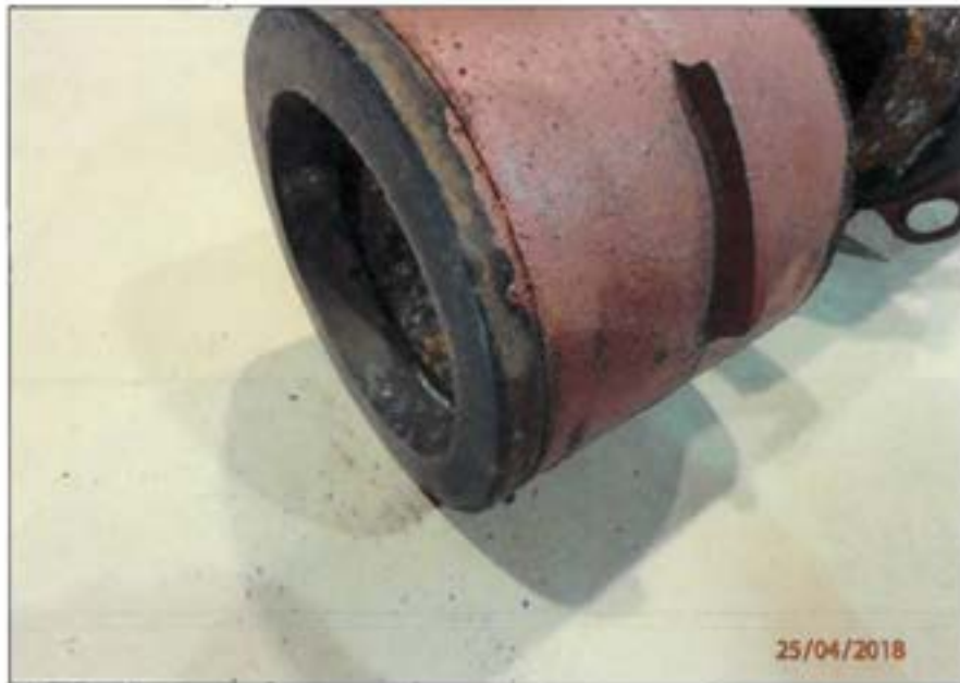
Figure 76 Rubber gasket on sleeve end where horizontal pipe separated.
