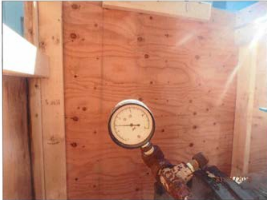
Figure 93 Positive pressure on ammonia side of chiller.
