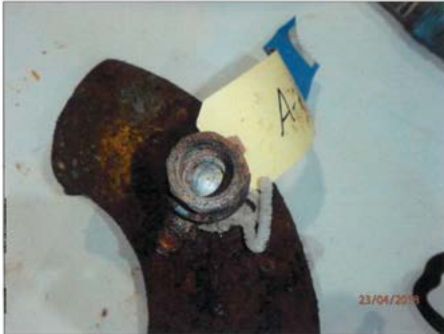
Figure 26 Closer view of ball on Valve A-10 showing light corrosion.
