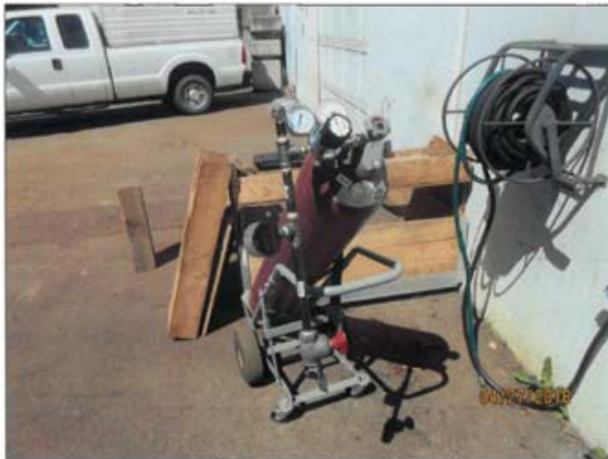
Figure 54 PRV test set-up. Argon was used to operate PRV Valve "2".
