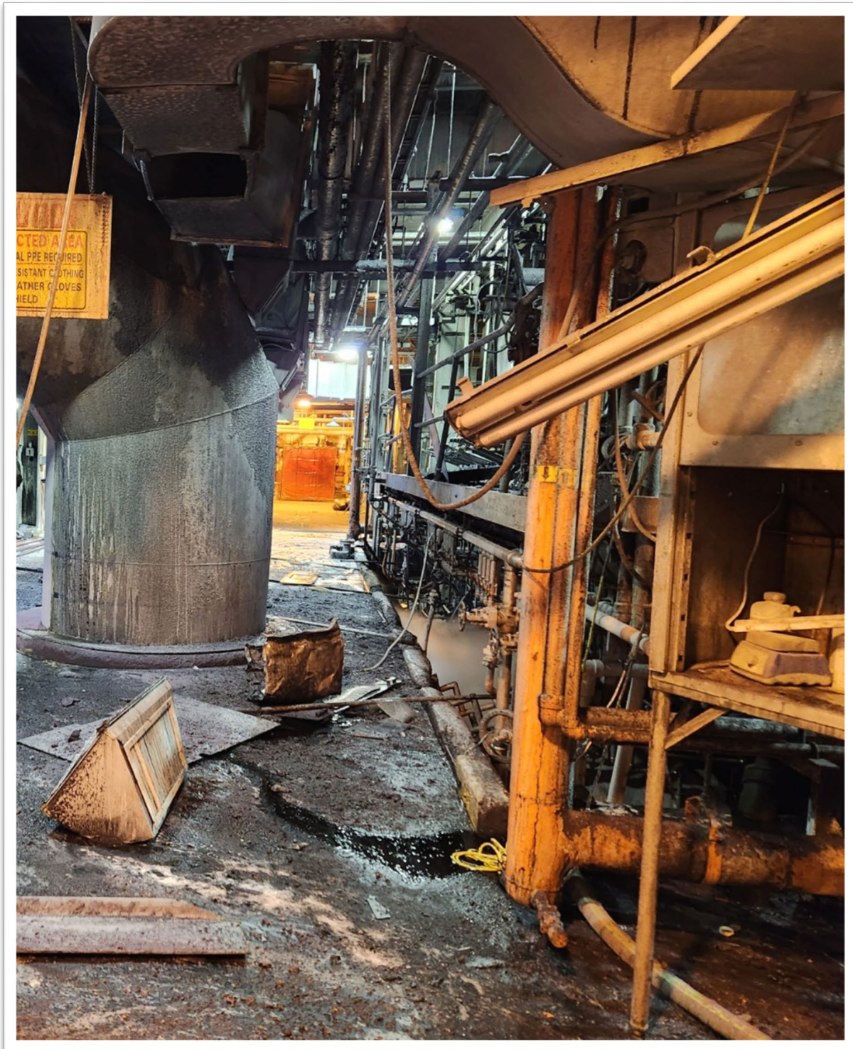
Photo 1 – Location of recovery boiler smelt spouts and dissolving tank.
