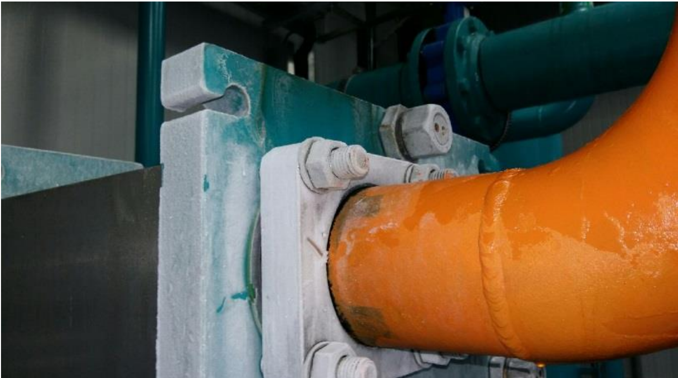
Image 1 NH3 Leak – no lock washer on bolts
