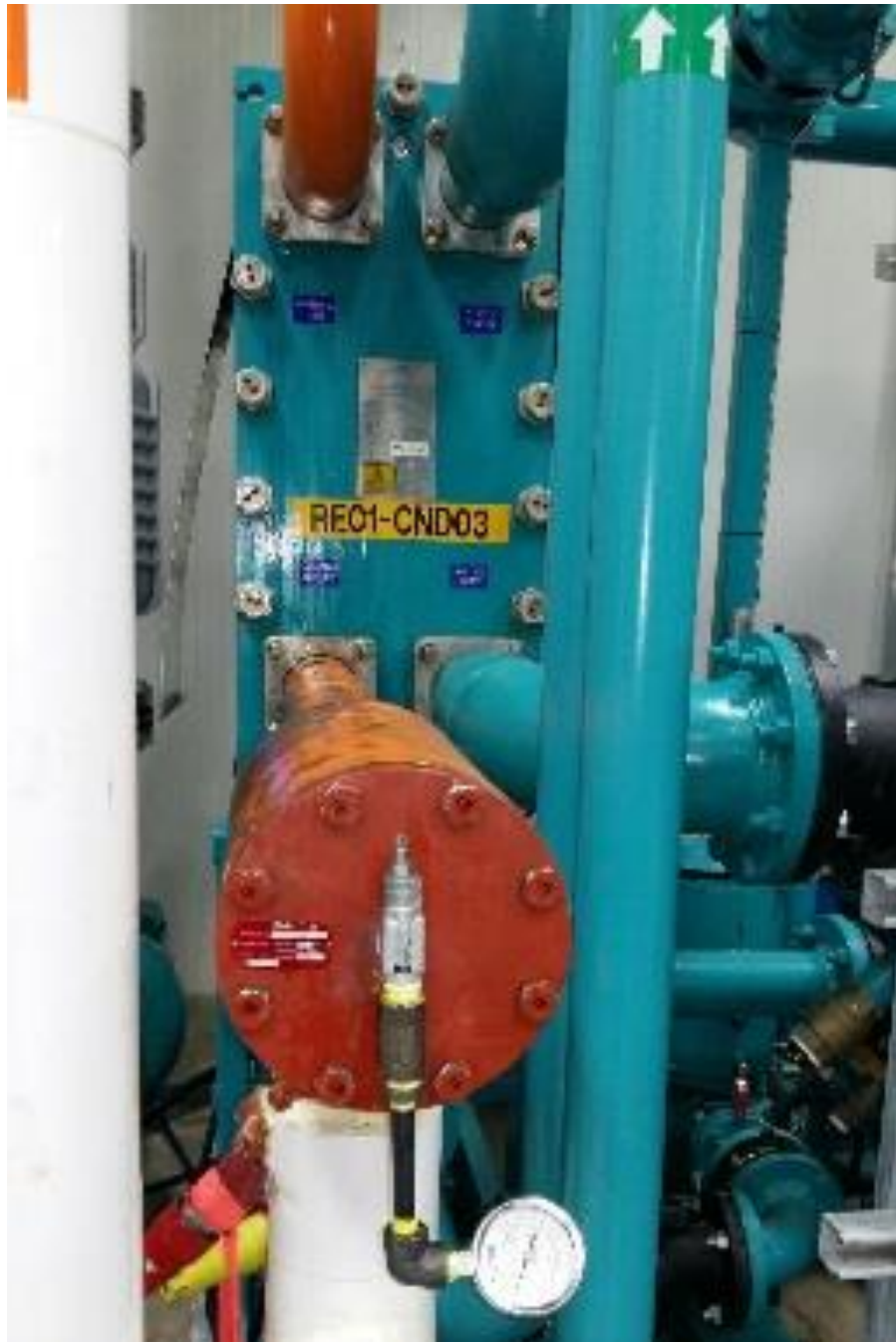
Image 5 Plate Heat Exchanger – NH3 & glycol
