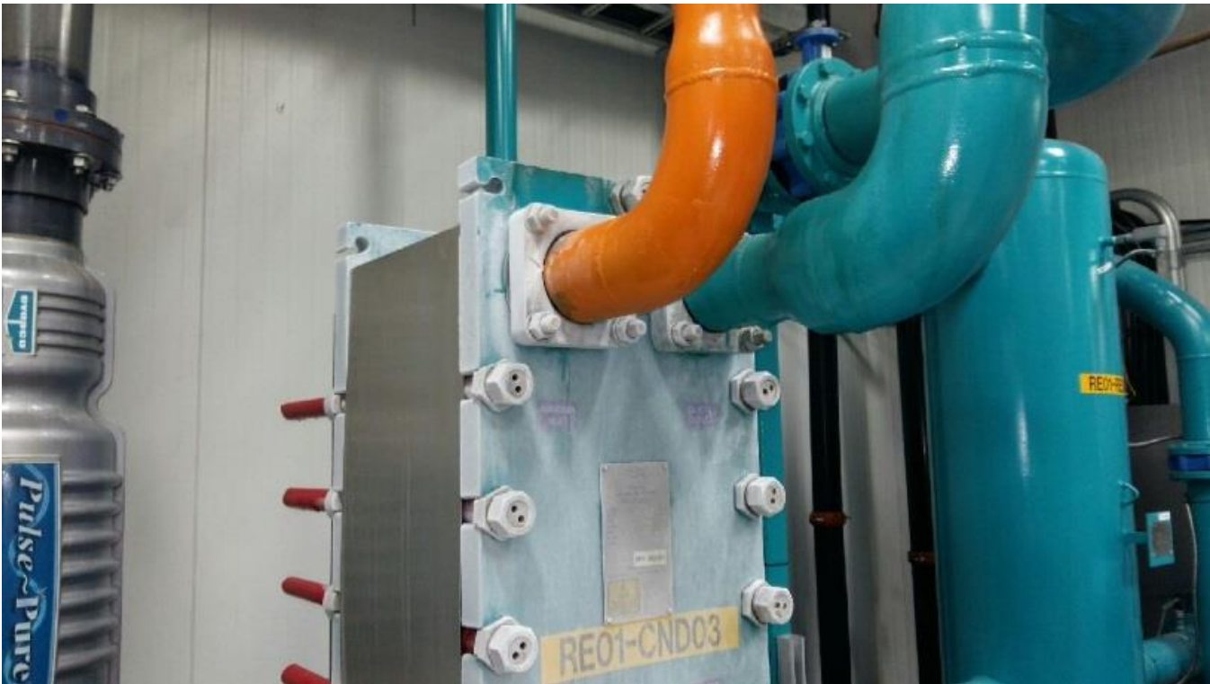
Image 2 Plate Heat Exchanger & NH3 Orange Pipe
