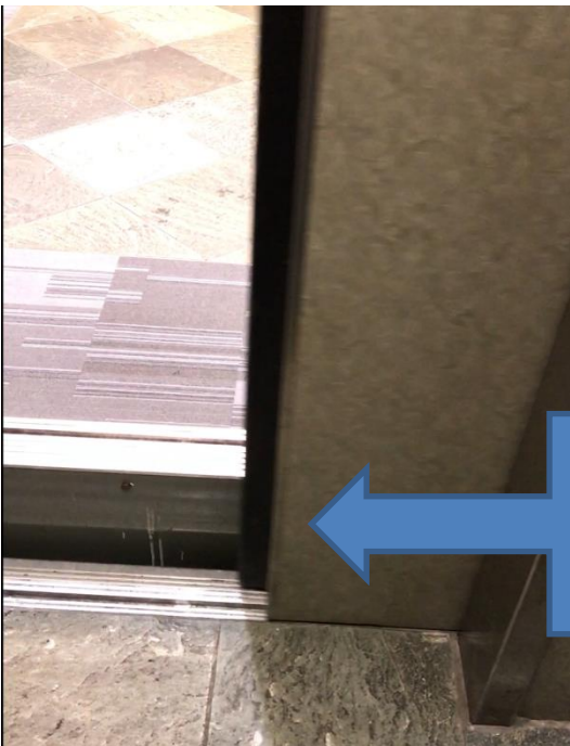
Picture 2 - showing the door opening wider and the elevator cab is still levelling into the landing,
