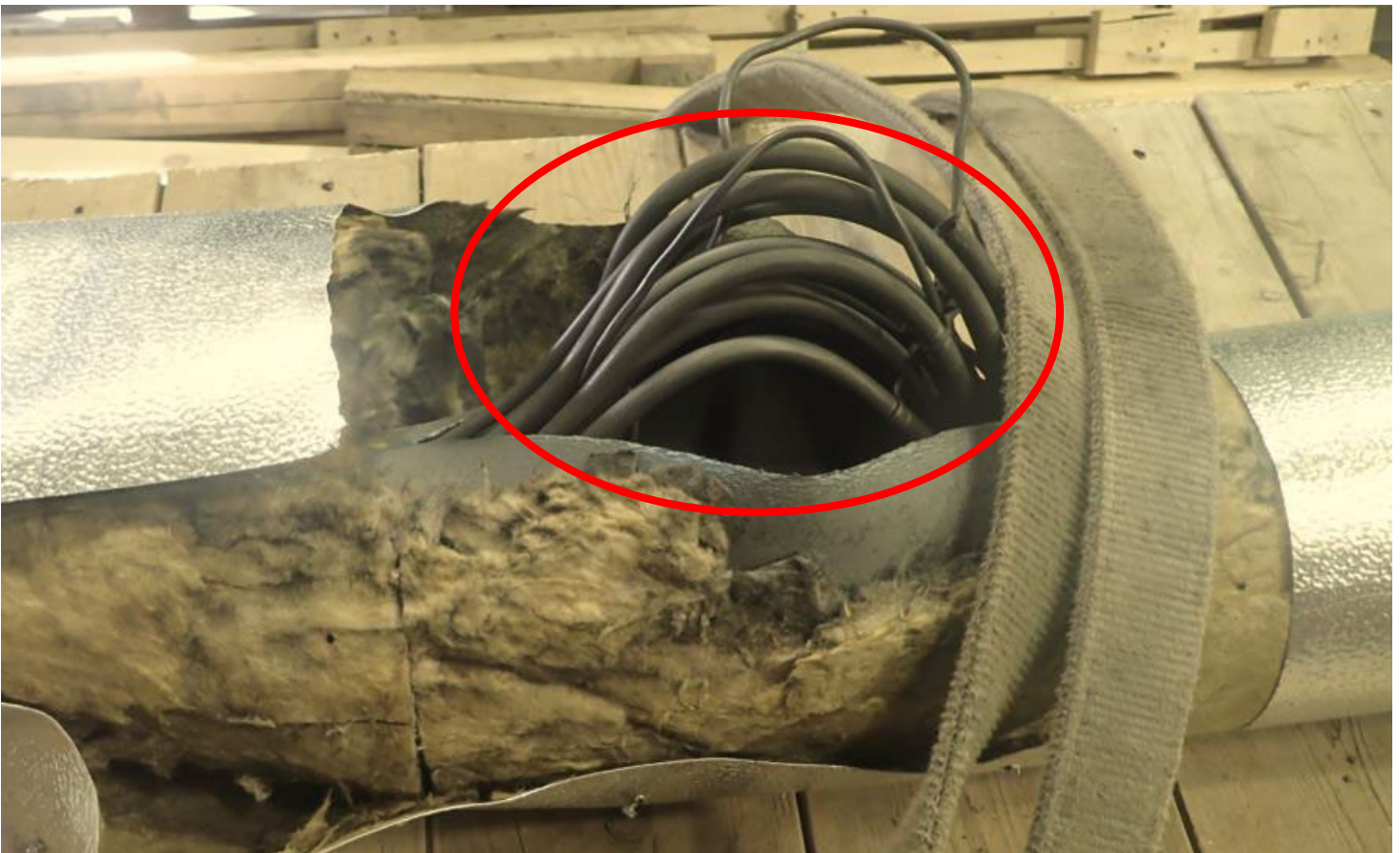
Photo 3: Heating coils displaced through rupture opening
