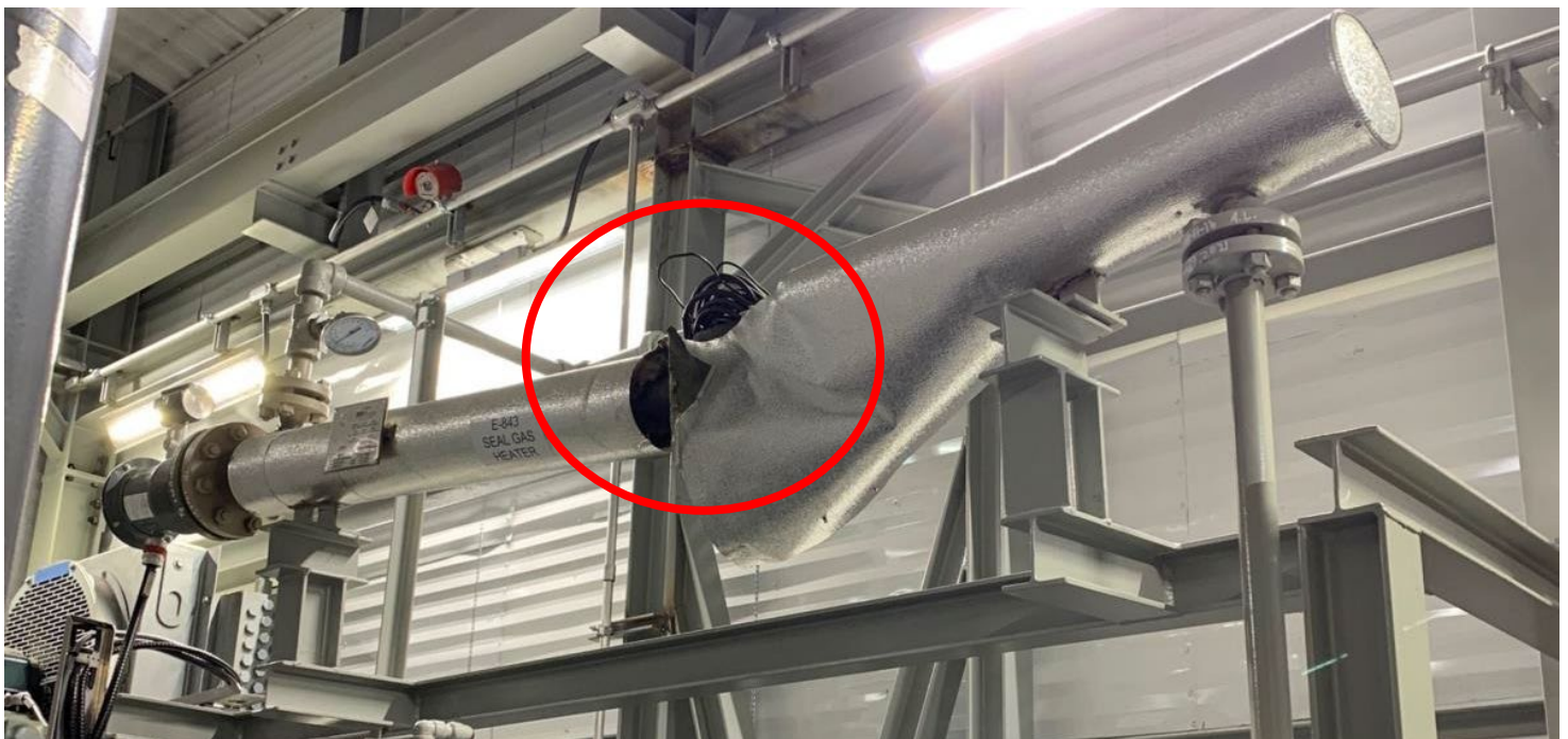
Photo 1: Overview of Heater
