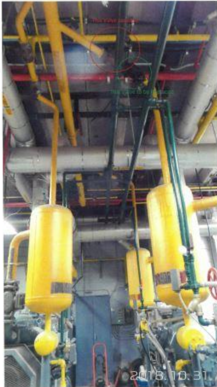
Image 3 - Discharge valve (Closed) and check valve (to be replaced)
