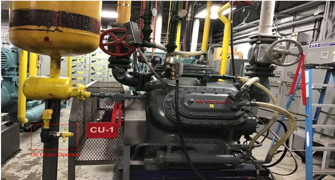
Image 1 - Oil drain valve opened
