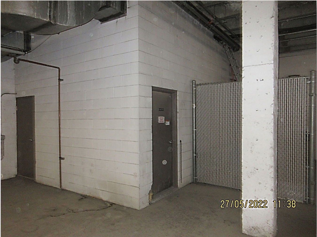
Photo 1 – Electrical room as seen from the parkade area.
