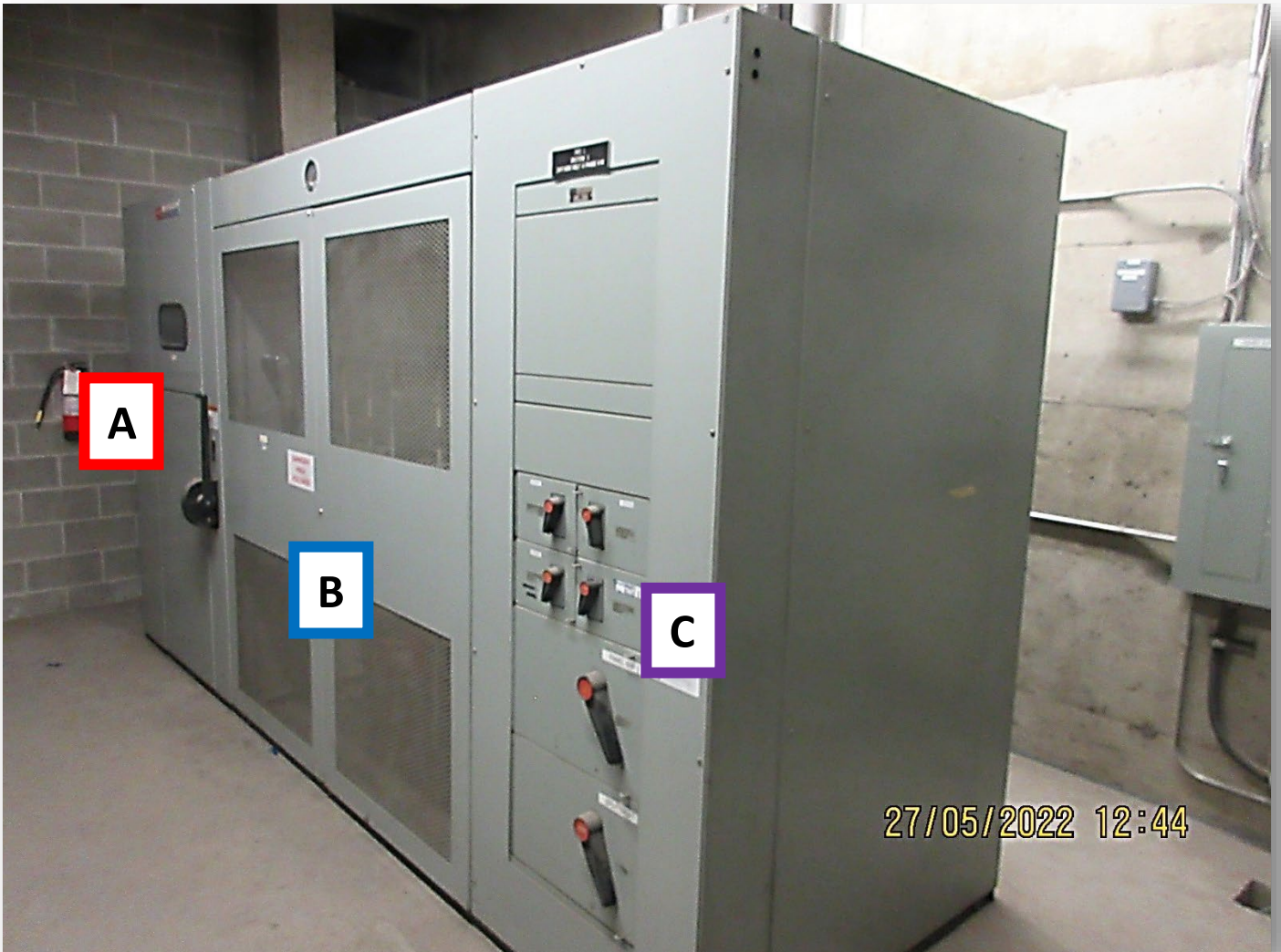
Photo 2 – Inside the electrical room/vault.
