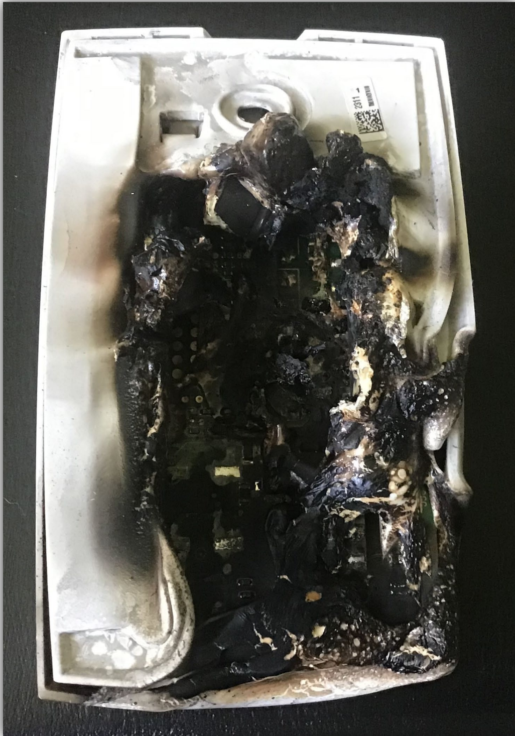
Image 3 - Damage to thermostat.
