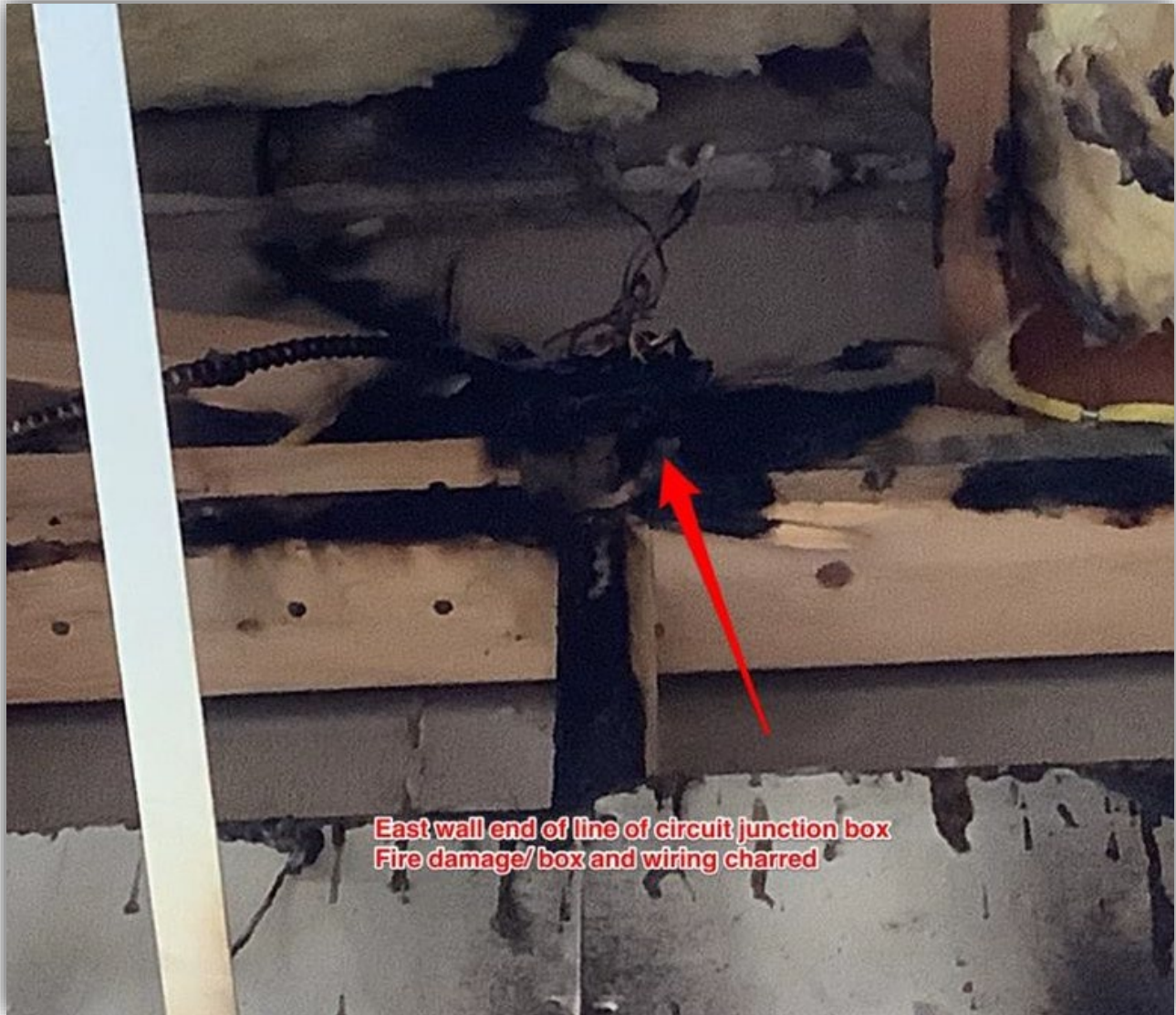
Image 4 – Damaged junction box.
