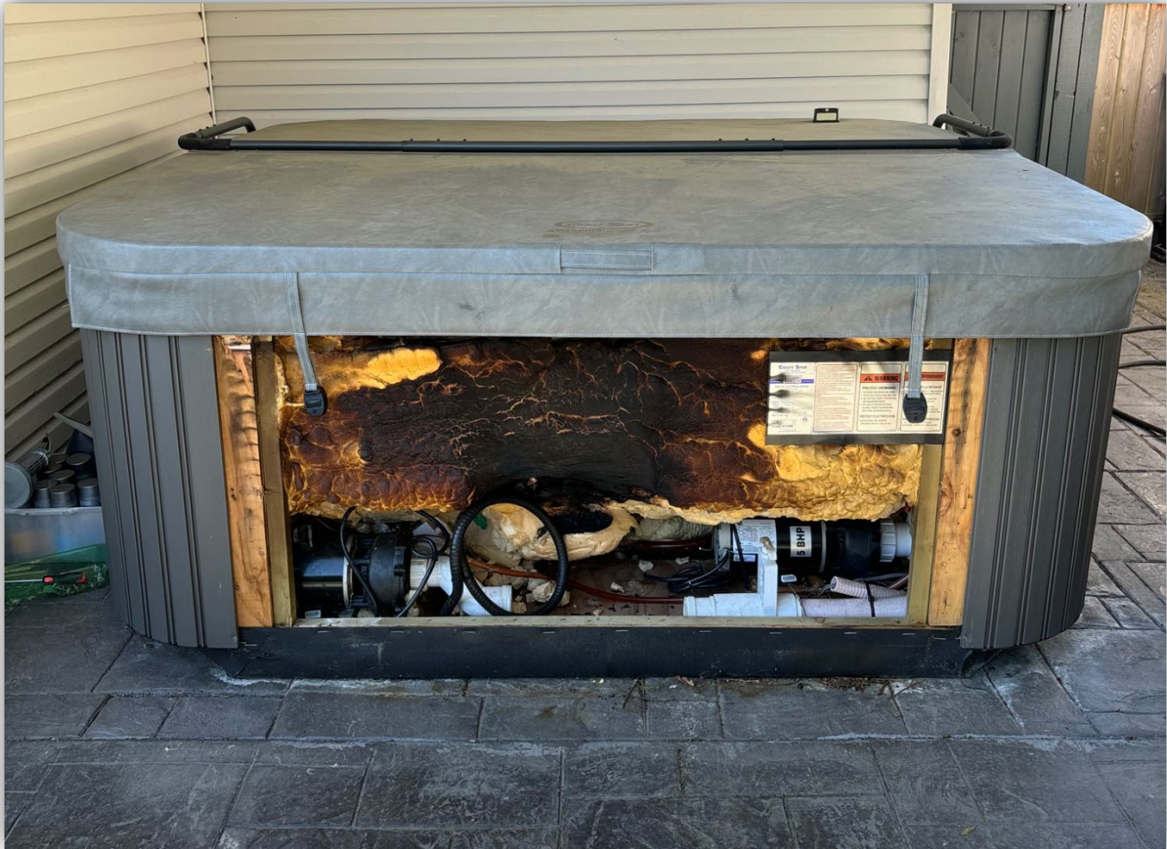
Image 1 – Damaged hot tub.
