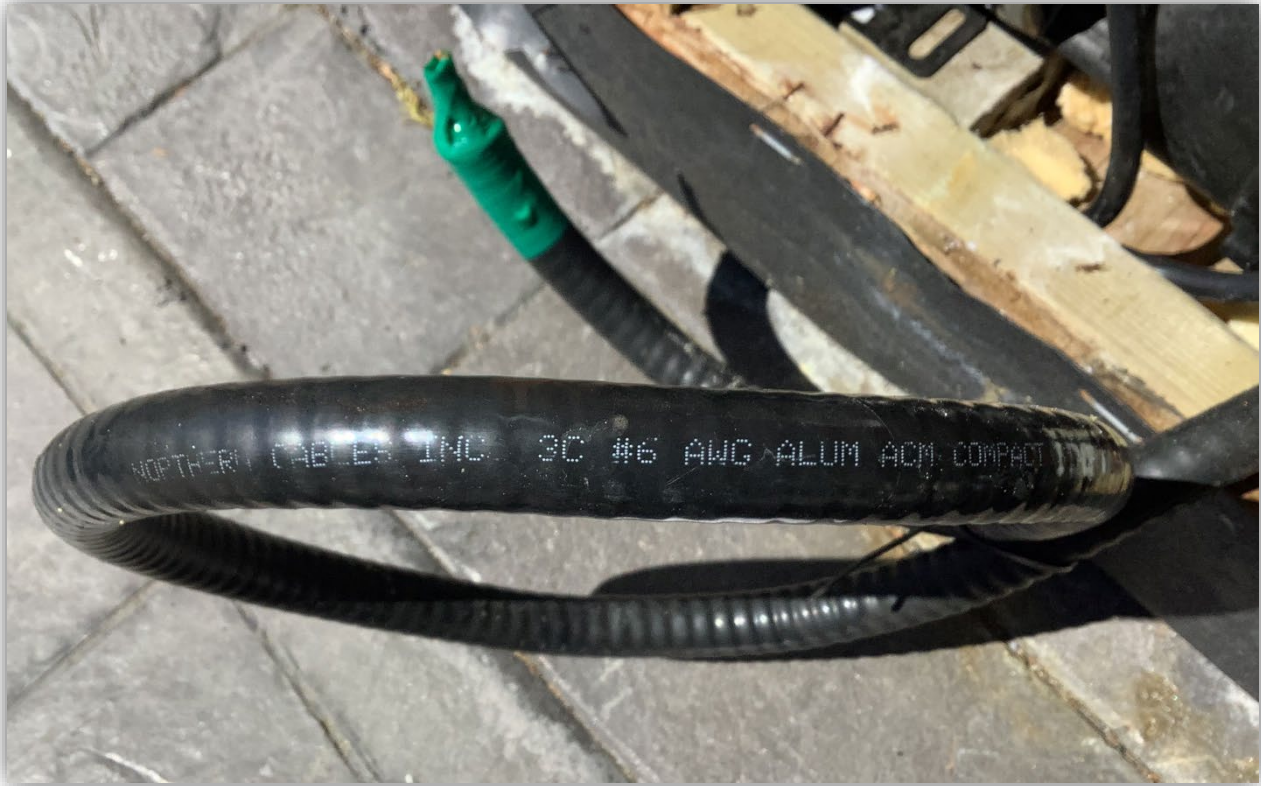
Image 4 – Aluminum conductor used to connect to the hot tub.
