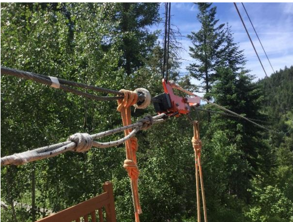
Brake System at Arrival Platform
