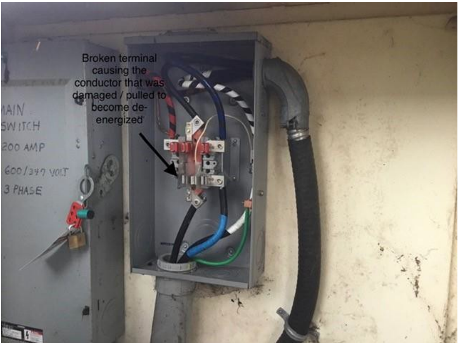
Image 2 - Location of power feeding the underground system that was damaged and the terminal that was broken off by force causing the conductor to be de-energized.
