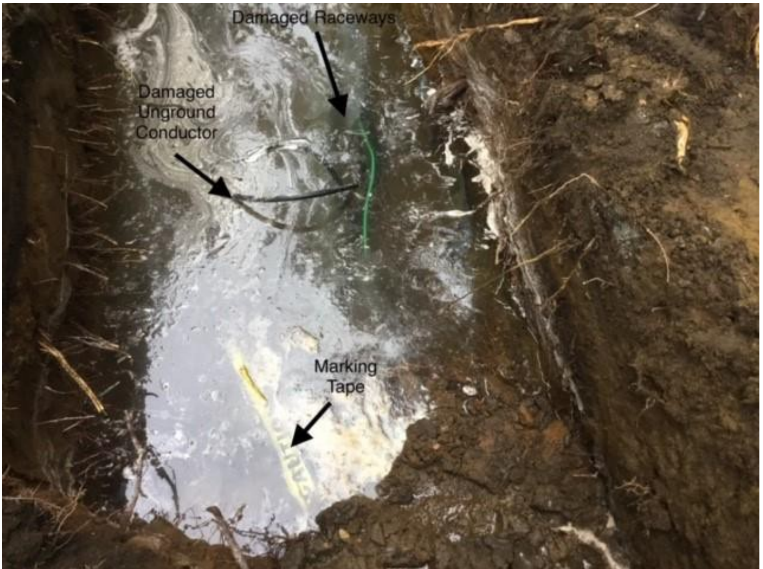
Image 1 - Location of damaged underground electrical system.
