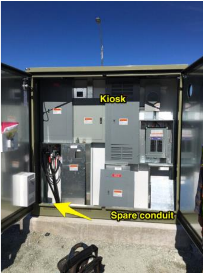
Photo 1: Electrical kiosk containing a spare conduit
