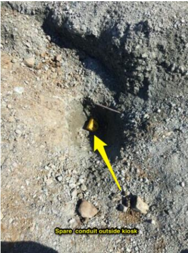
Photo 3: Other end of spare conduit leading to kiosk
