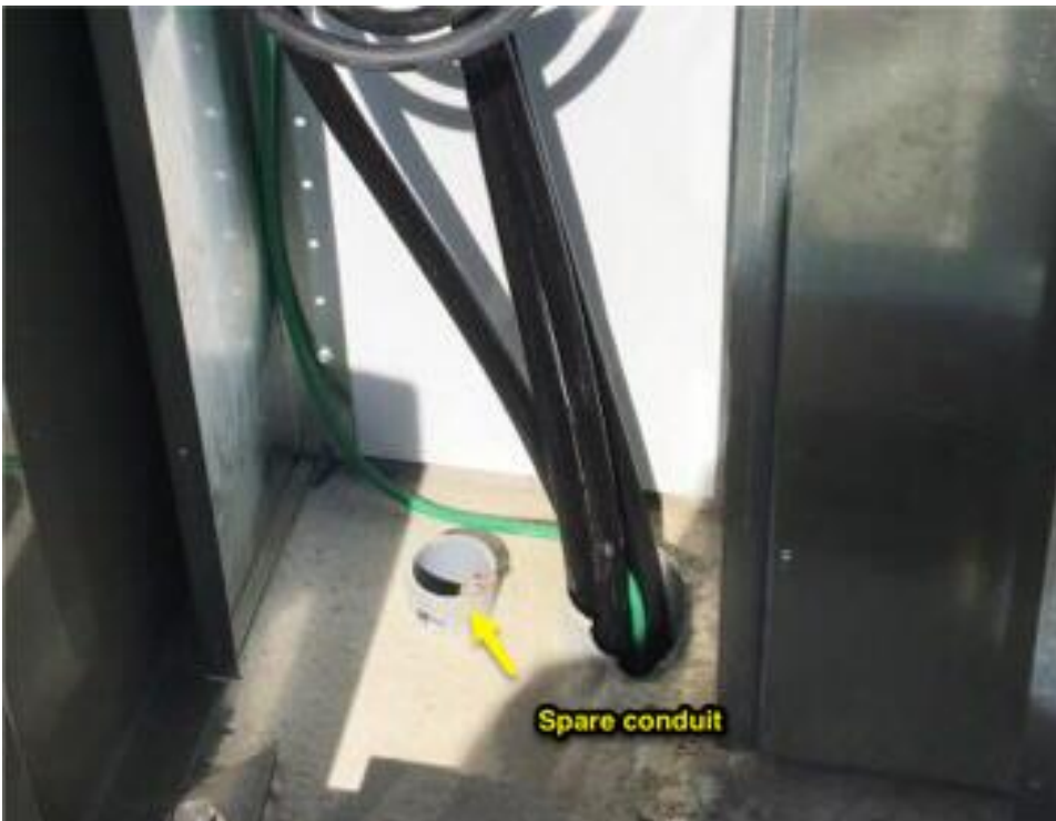
Photo 2: Spare conduit on floor of kiosk
