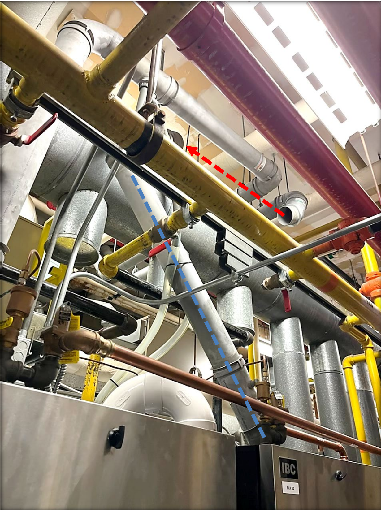
Image 3 – Boiler B2 venting system disengaged (red line) and knocked over (blue line).
