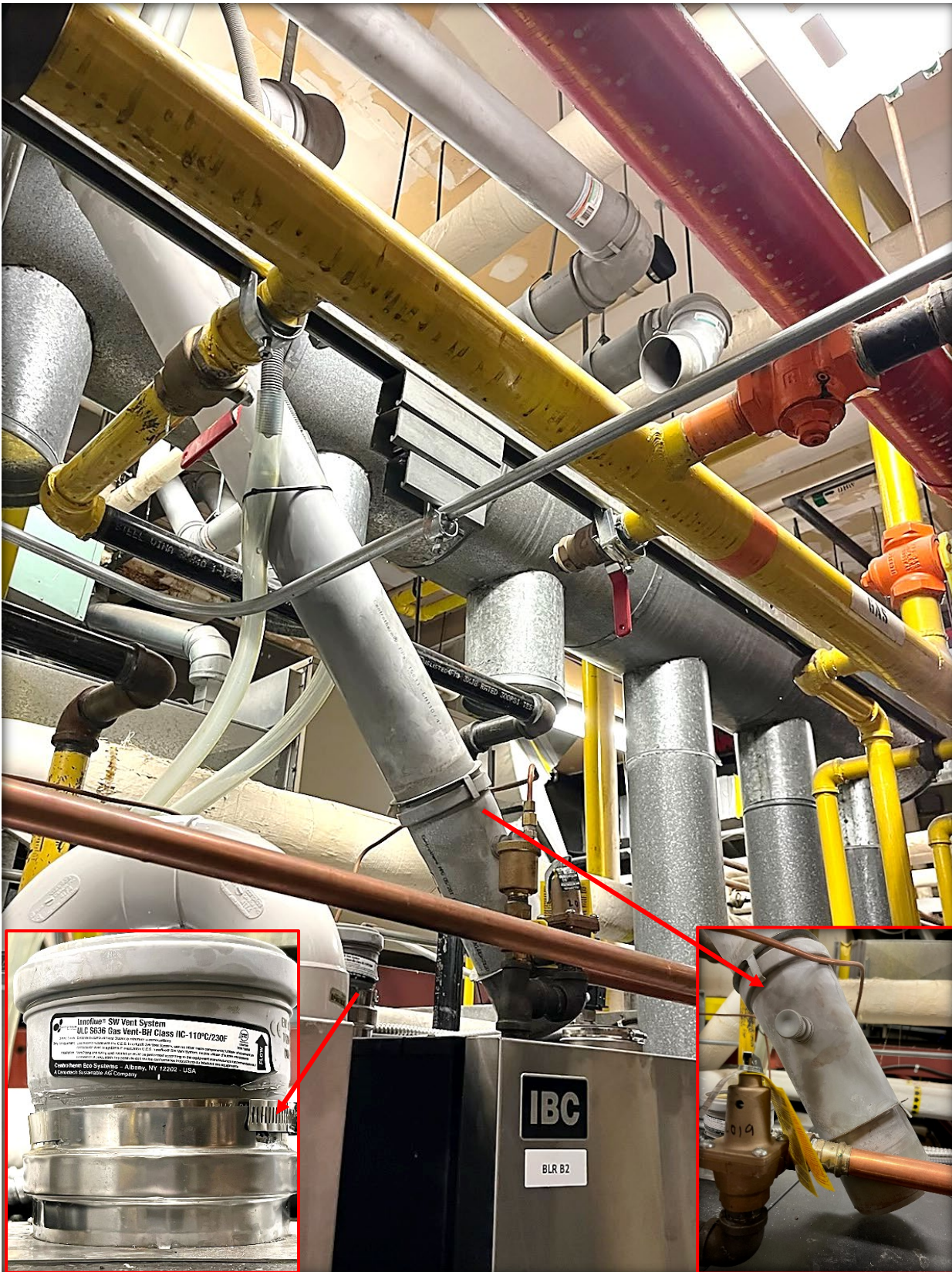
Image 2 – Boiler B2 after the incident with the venting system disengaged and knocked over.
