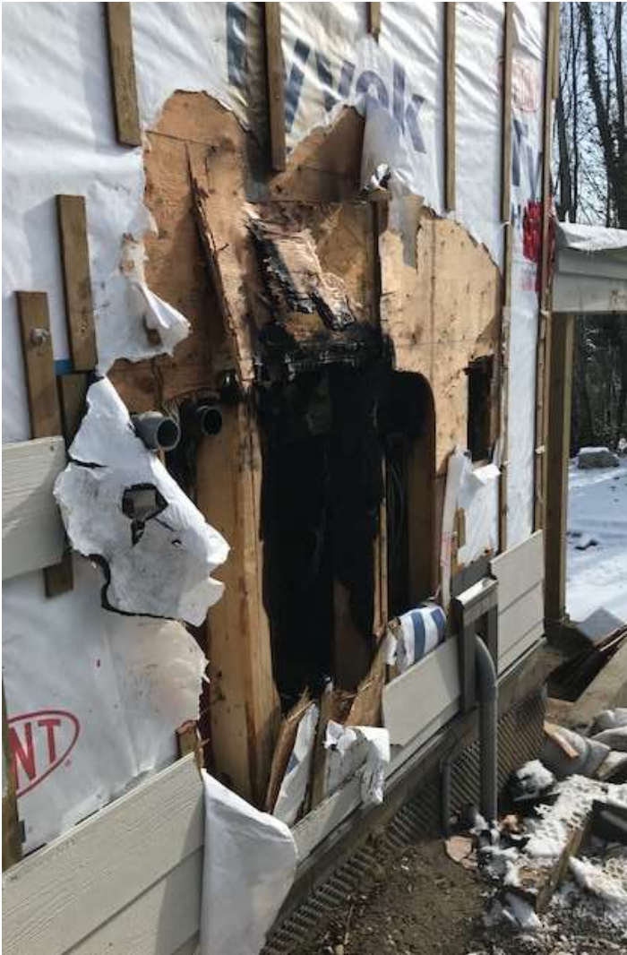
Resulting fire damage
