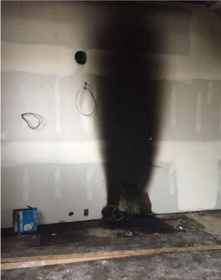
Location of junction at range box a lite gauge (under-sized) copper extension cord
