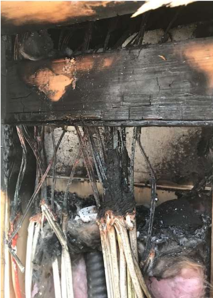
Resulting fire damage
