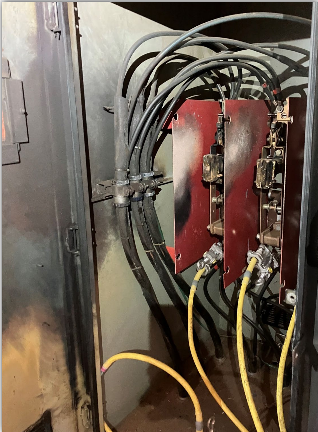
Photo 4 – Inside the local disconnect.
