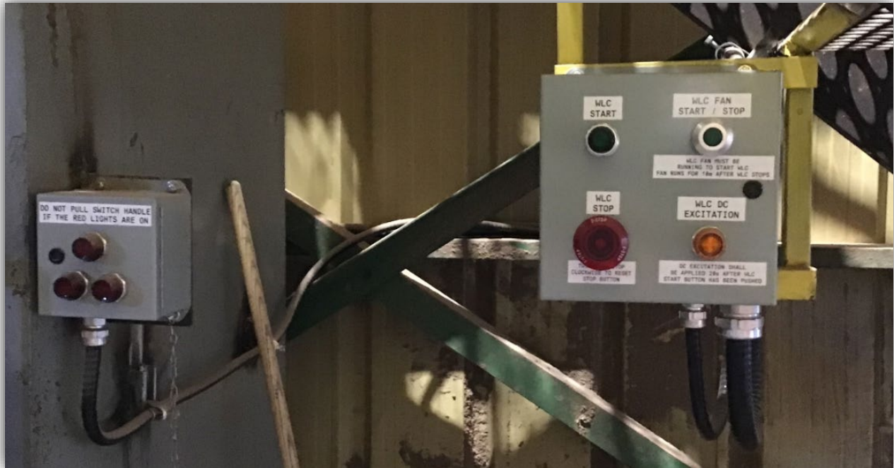
Photo 8 - New controls beside switch (post incident).
