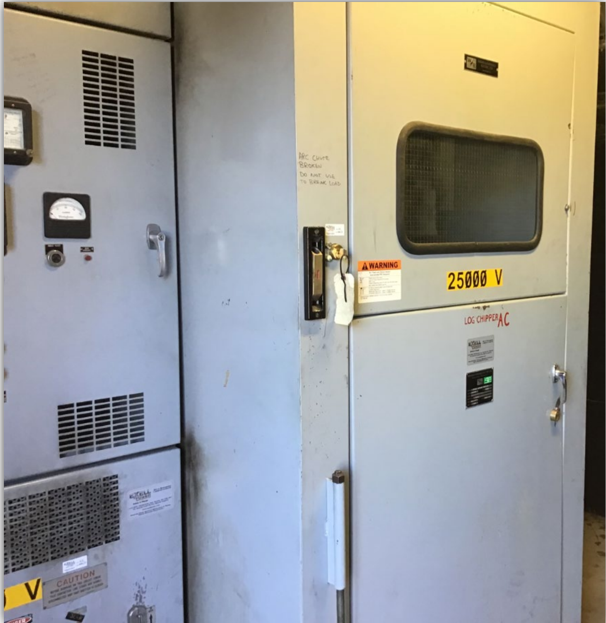
Photo 6 – High voltage equipment
