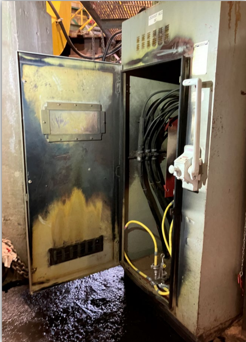
Photo 2 – Arc flash damage
