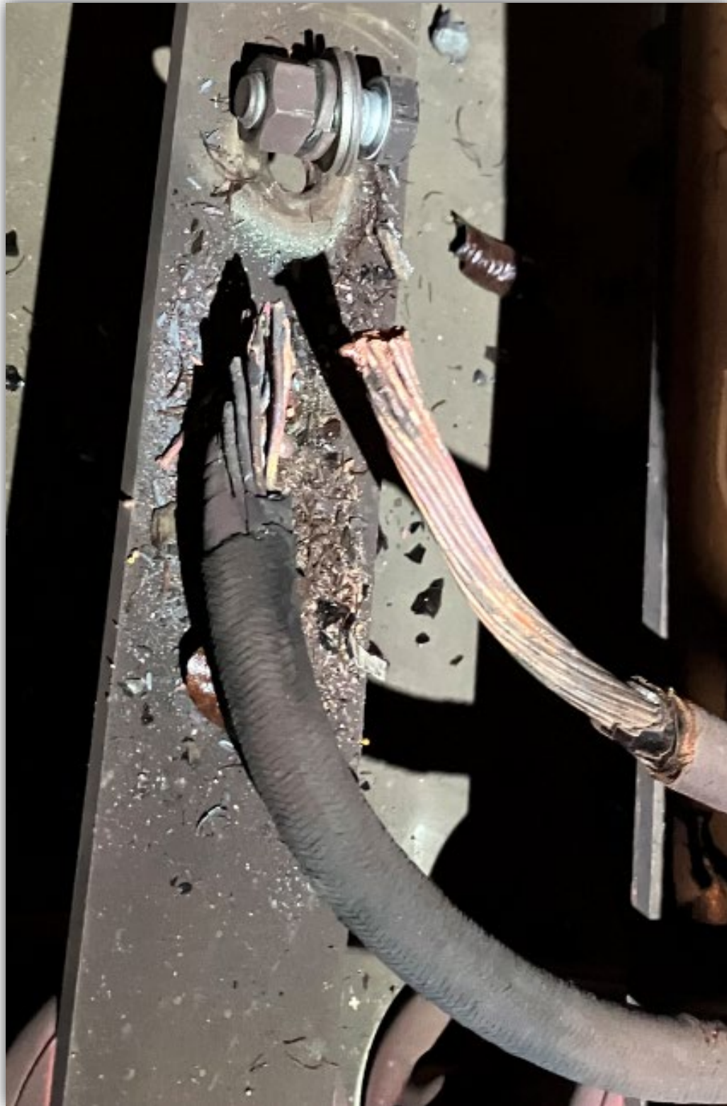
Photo 5 – High voltage feeder connections
