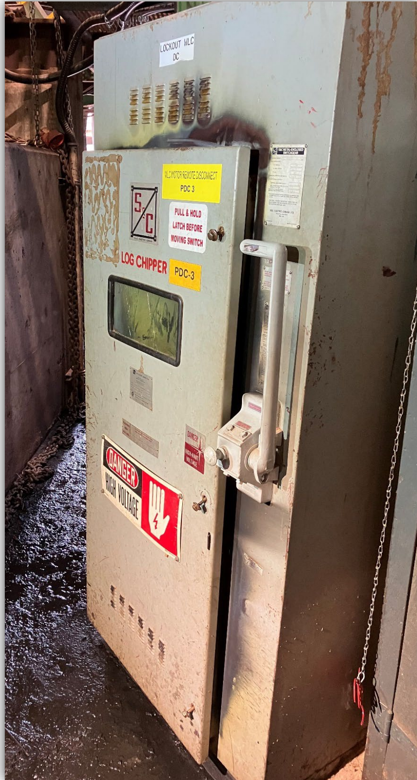
Photo 3 – Whole log chipper local disconnect.
