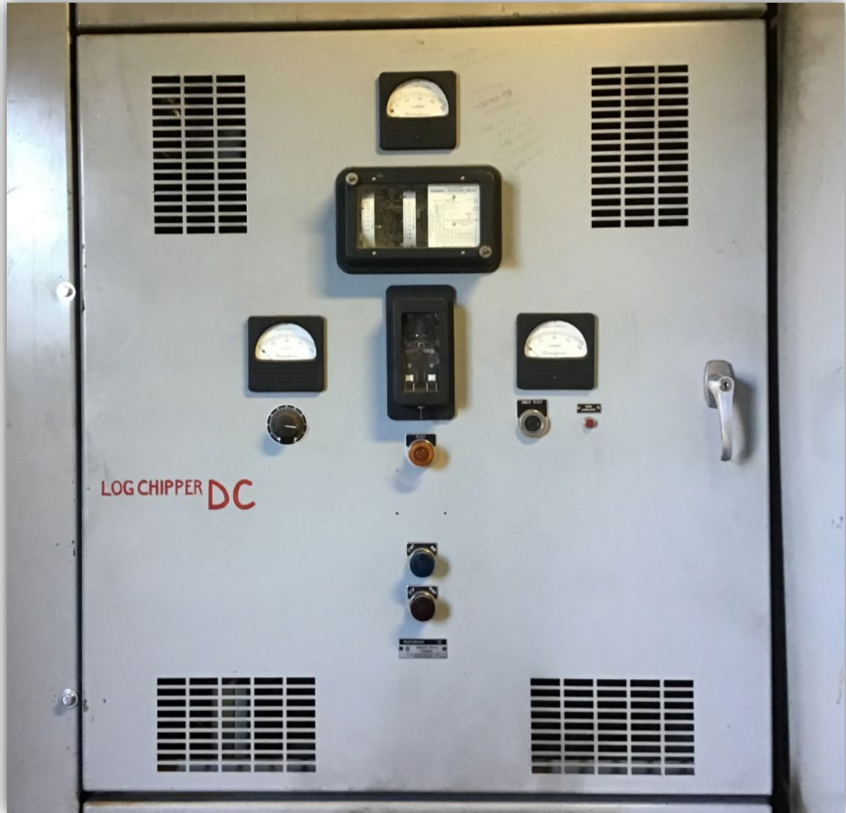
Photo 7 – Direct current controls in high voltage room
