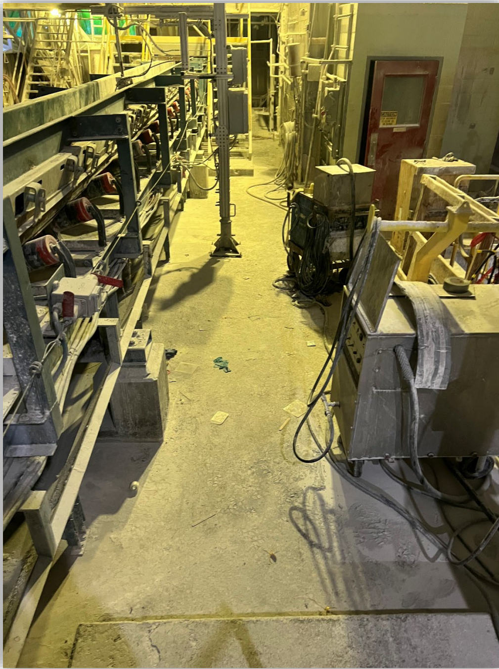
Image 1 – Area of work and equipment. Floor opening and overhead crane located on the right-hand side over the handrail.
