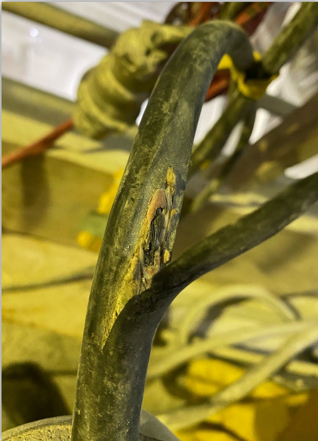
Image 8 - Close-up of cable damage and exposed conductor.
