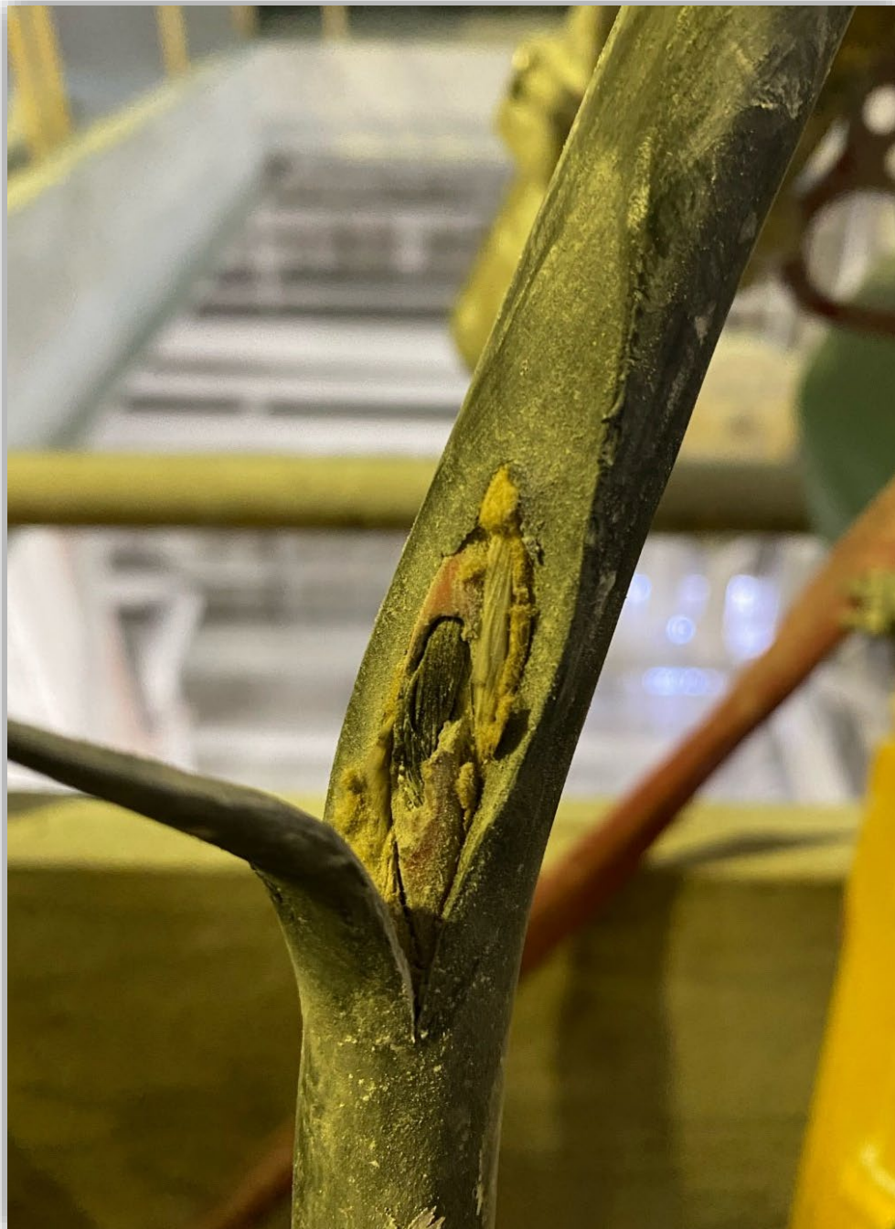
Image 7 - Close-up of cable damage and exposed conductor.
