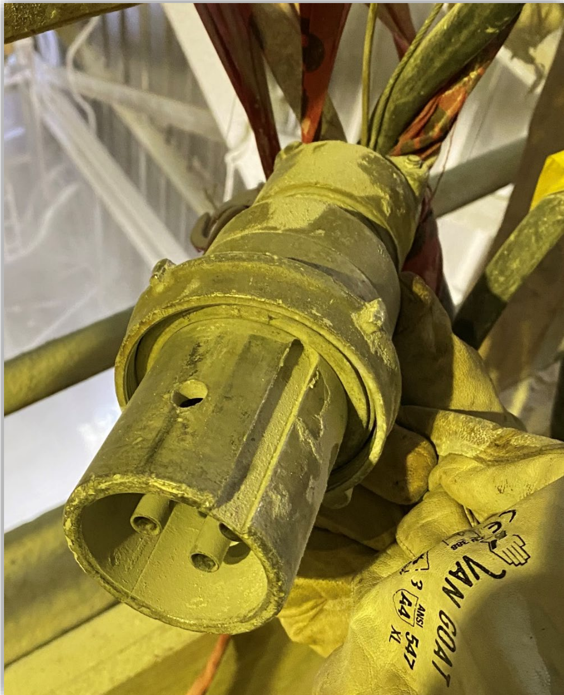
Image 5 – Plug end of the crane feeder cable disconnected from the receptacle after incident.
