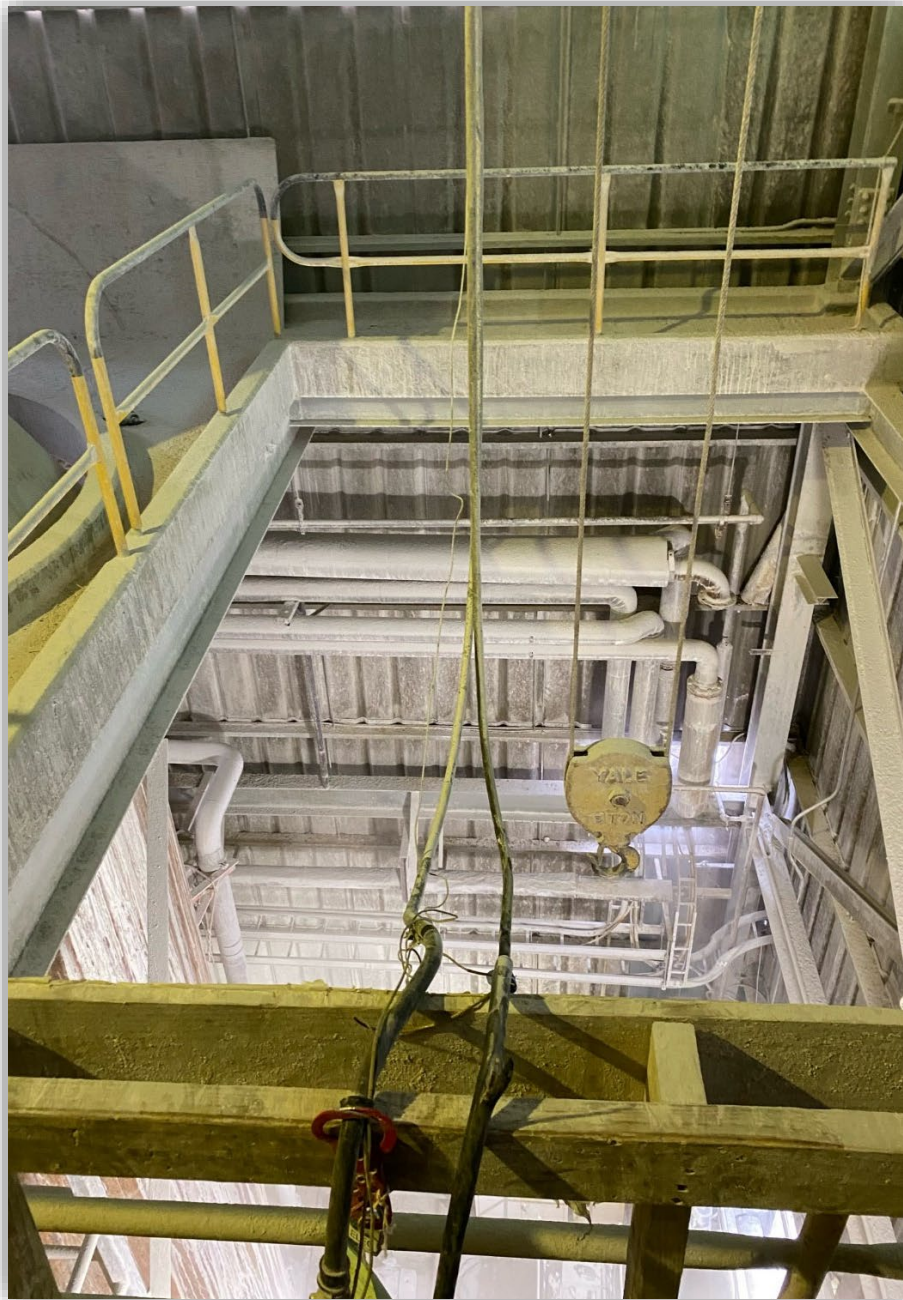
Image 2 – Crane lifting bay with damaged cable and control pendant in the approximate location and position when the incident occurred.
