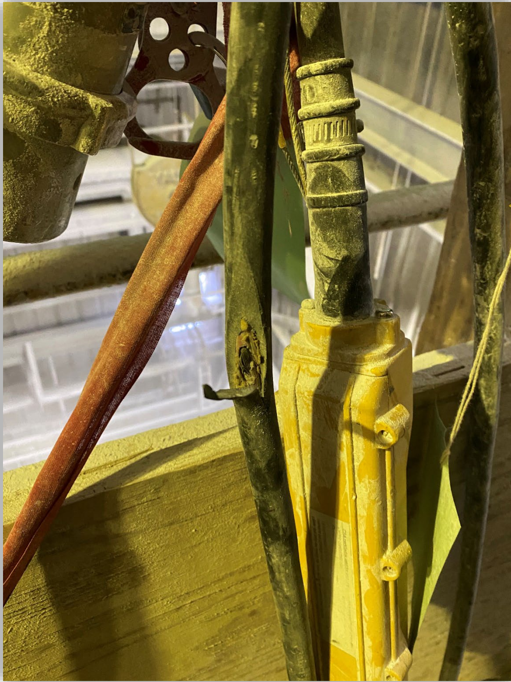
Image 6 – Crane operation pendant and damaged electrical cable on the handrail of the floor opening and overhead crane operation.
