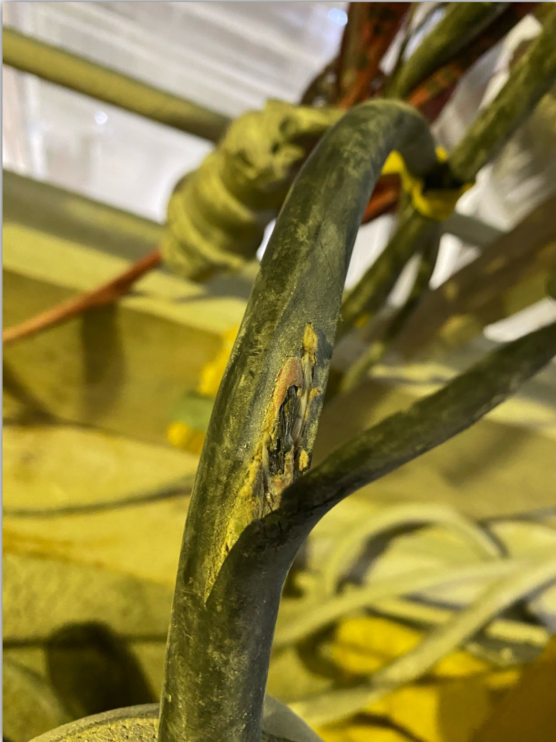
Image 3 - Close-up of cable damage and exposed conductor.
