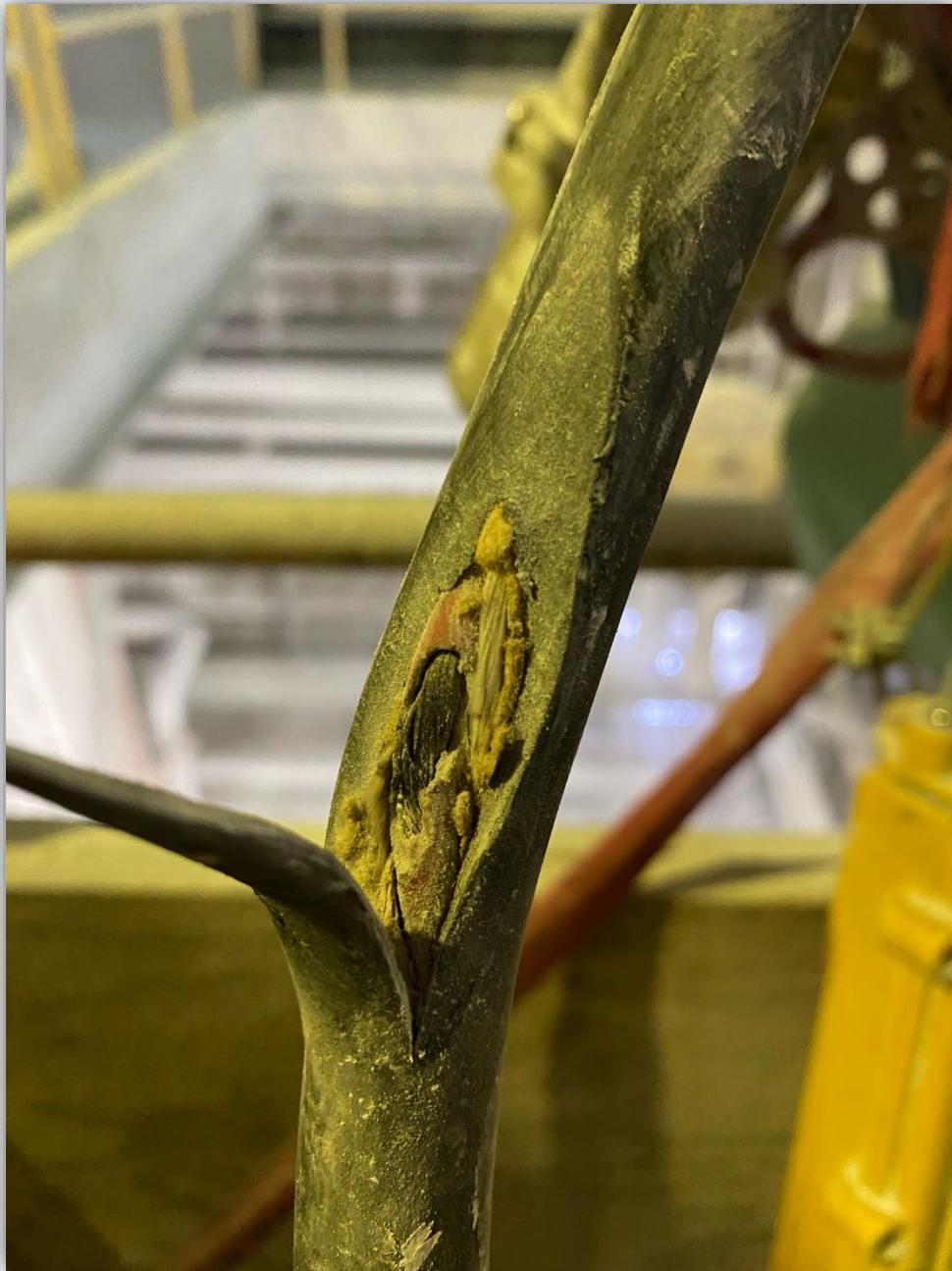
Image 2 - Close-up of cable damage and exposed conductor.
