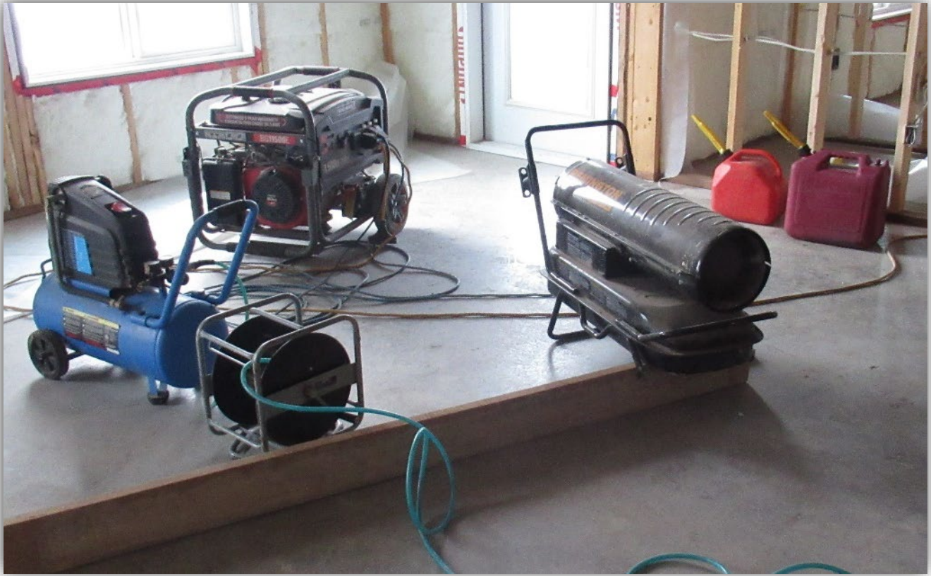
Image 2 – Gasoline generator (middle) found indoors powering a small air compressor (left) and a kerosine/diesel fueled space heater (right).
