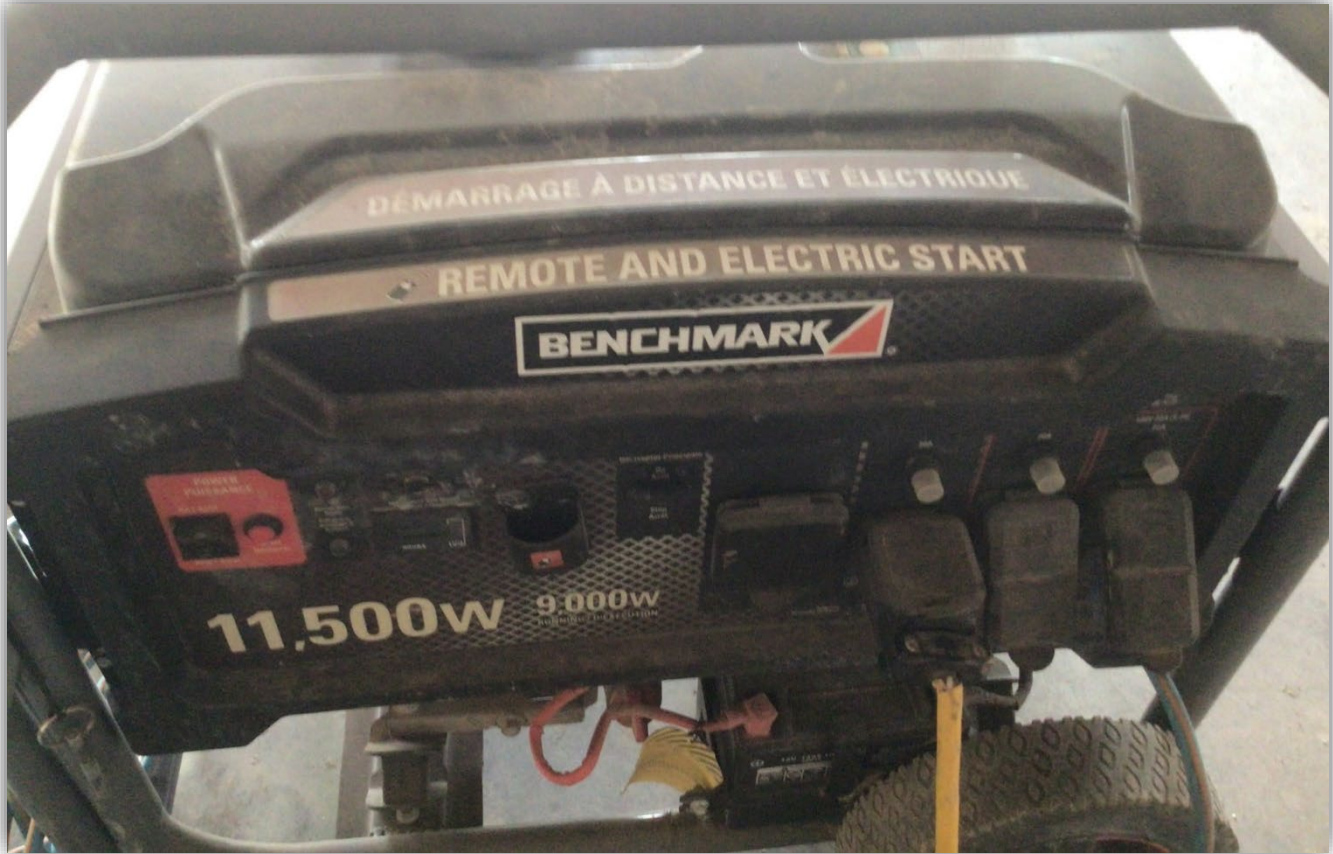
Image 3 – Front of generator.
