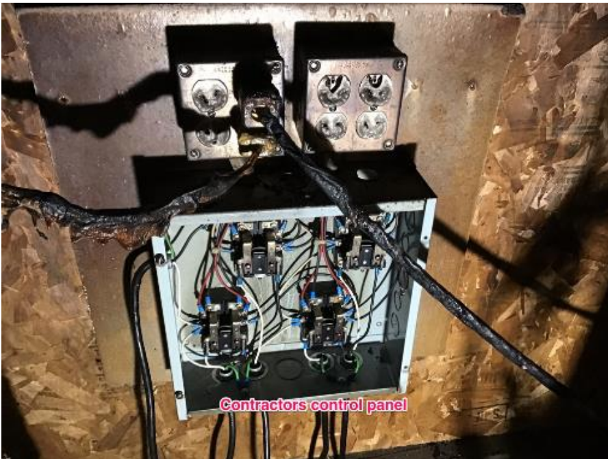
Photo 9: Extension cords heat damaged, wiring inside steel box are not damaged (photo provided by Fire/Rescue)
