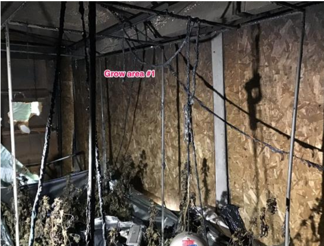
Photo 10: Fire damage in South grow area #1 (photo provided by Fire/Rescue)
