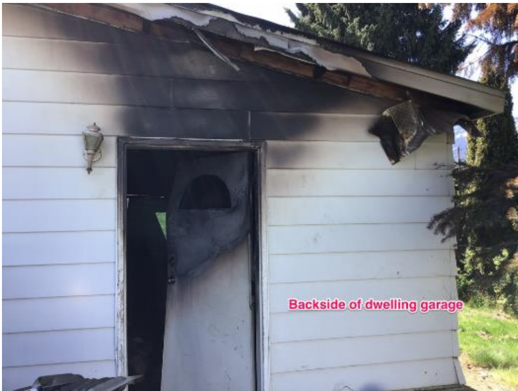
Photo 1: Burn marks and soot residue on door and outside wall due to fire within (photo by Fire/Rescue)
