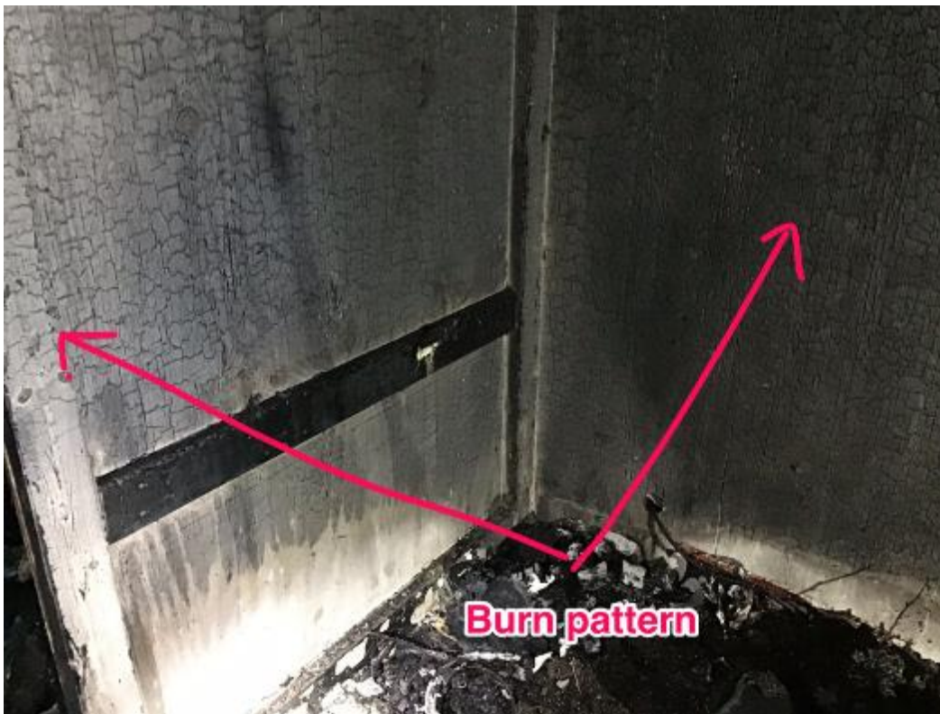
Photo 3: Burn patterns on the wall near the fire origin (photo provided by Fire/Rescue)
