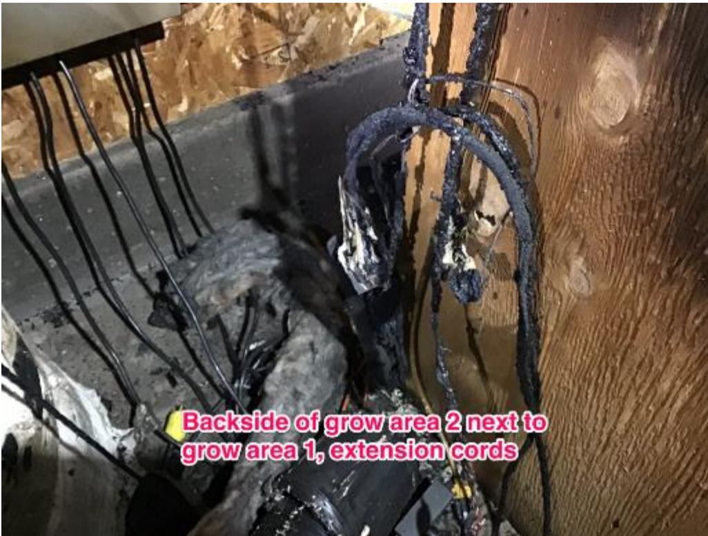
Photo 8: Extension cords used, significant heat damage (photo provided by Fire/Rescue)
