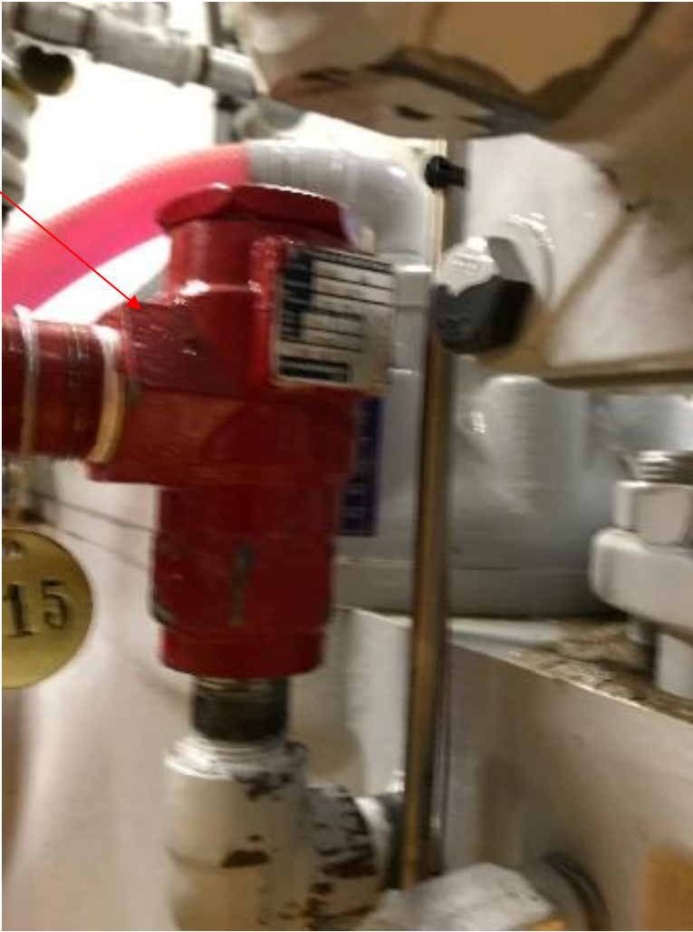
Side View of Normal Pipe Size \frac{3}{4} close nipple upstream of elbow.
