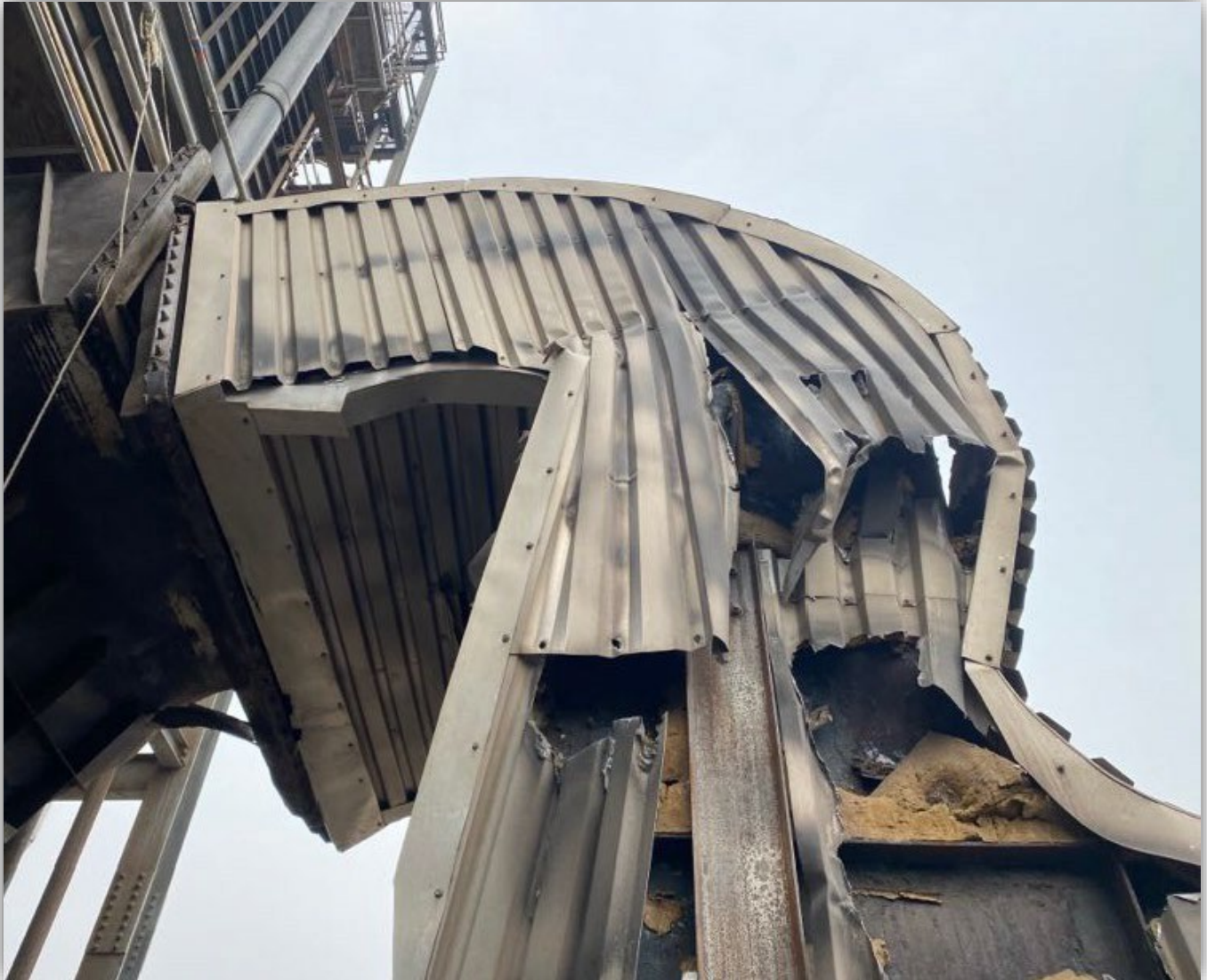
Image 7 – Damaged convection ducting.
