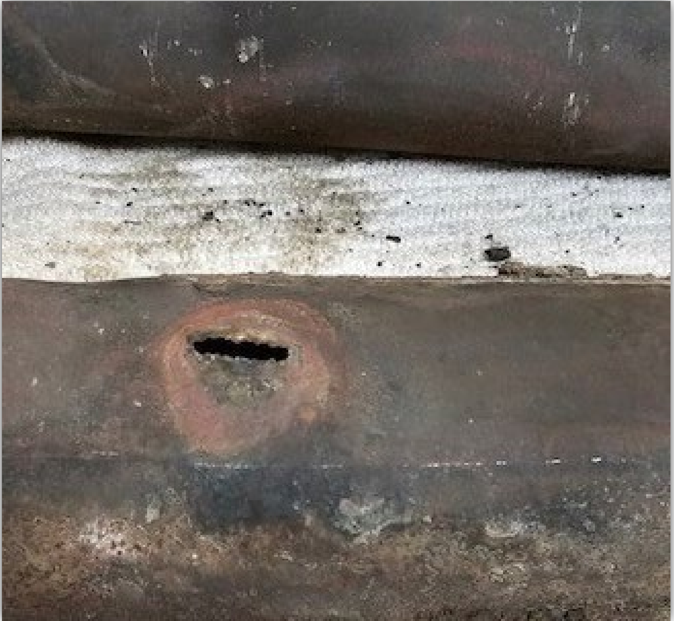
Image 5 - Face of failed tube.
