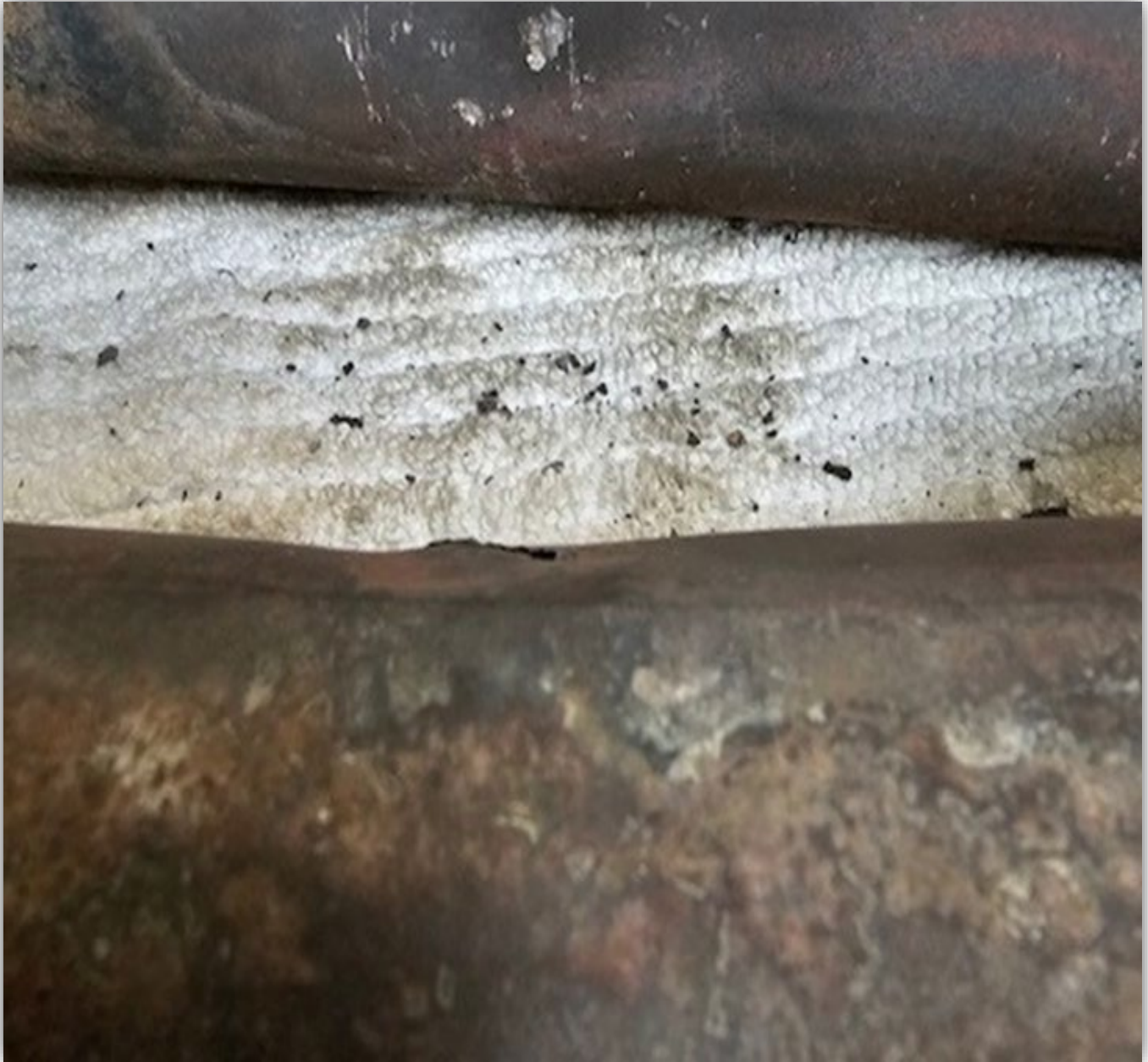
Image 6 – Side view of failed tube.
