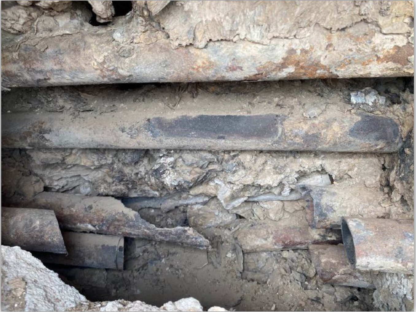
Image 4 - Location of tube failure.
