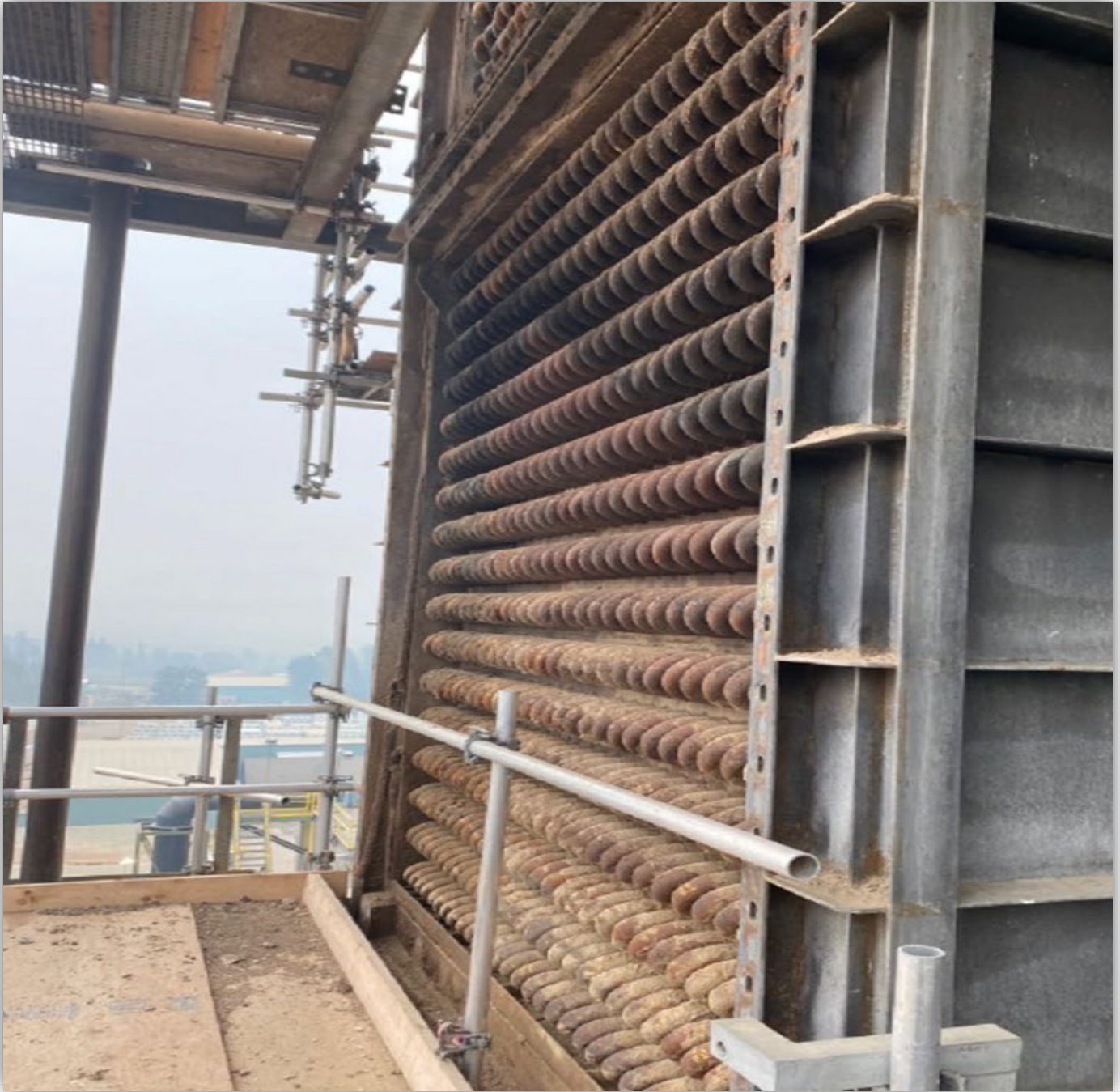
Image 3 – East side of failed S-tube heat exchanger.
