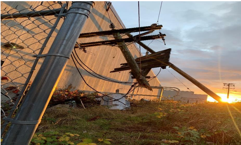
(Photo #1) High voltage transformer platform collapsed
