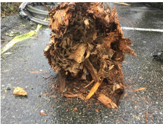
(Photo #2) West pole dry rotted out at base where subject to years of wet soil.
