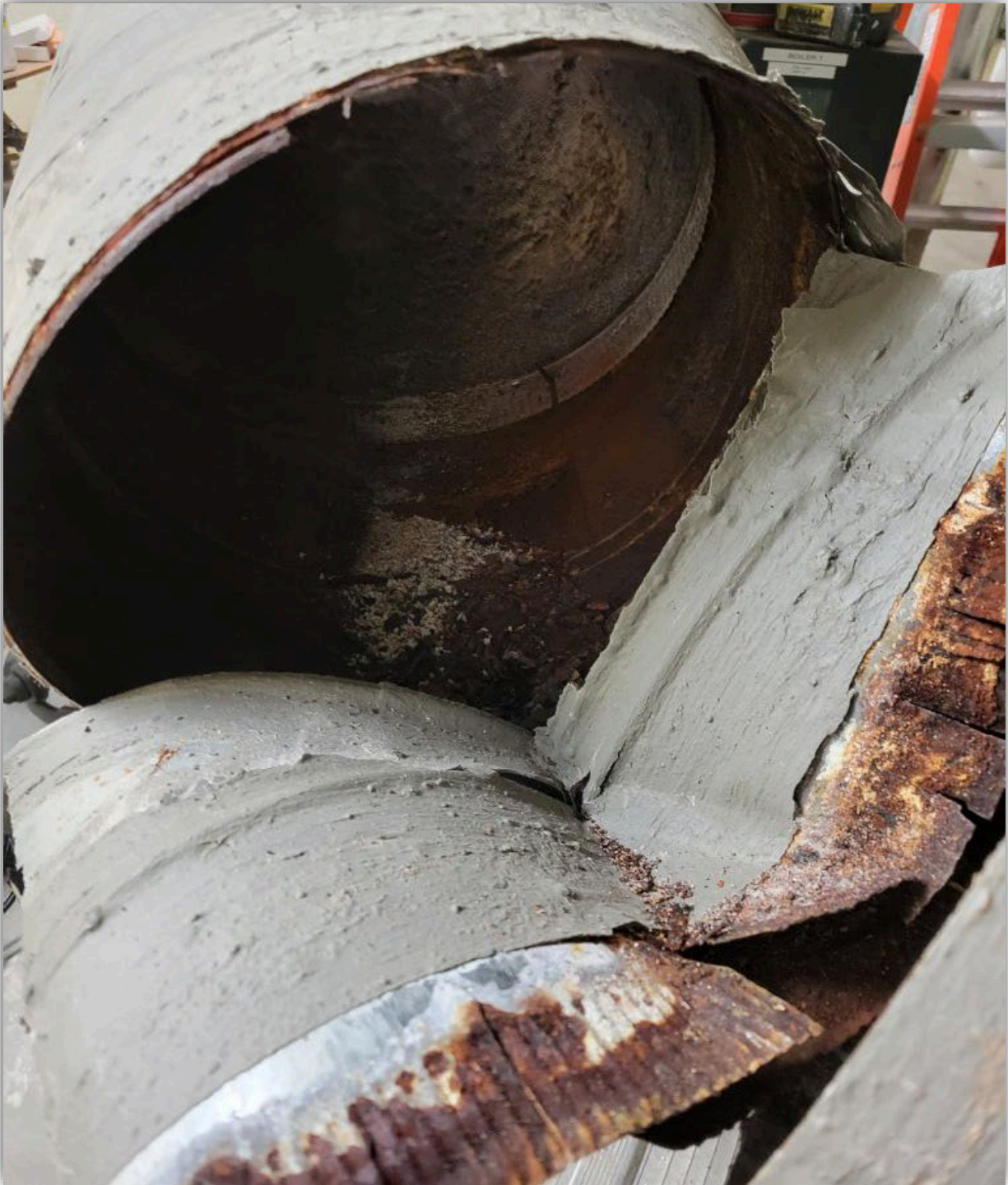
Photo 4 – Venting common header with corrosion damage, photo taken after removal.
