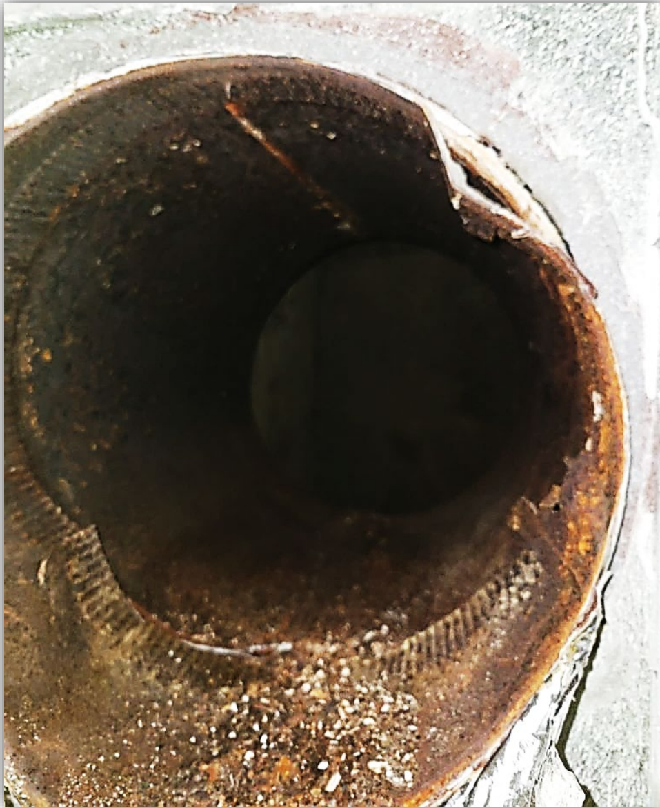
Photo 3 - Vent common header interior going into chimney with no pipe going upwards, concrete cinder blocks are visible.
