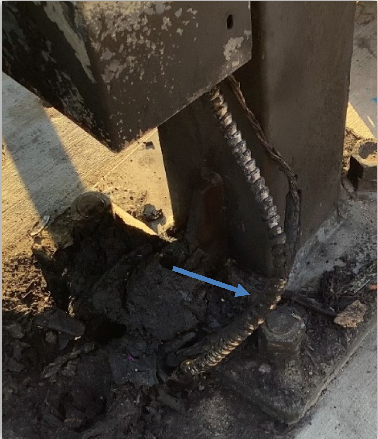
Image 4 - Cable fail point inside bus shelter.
