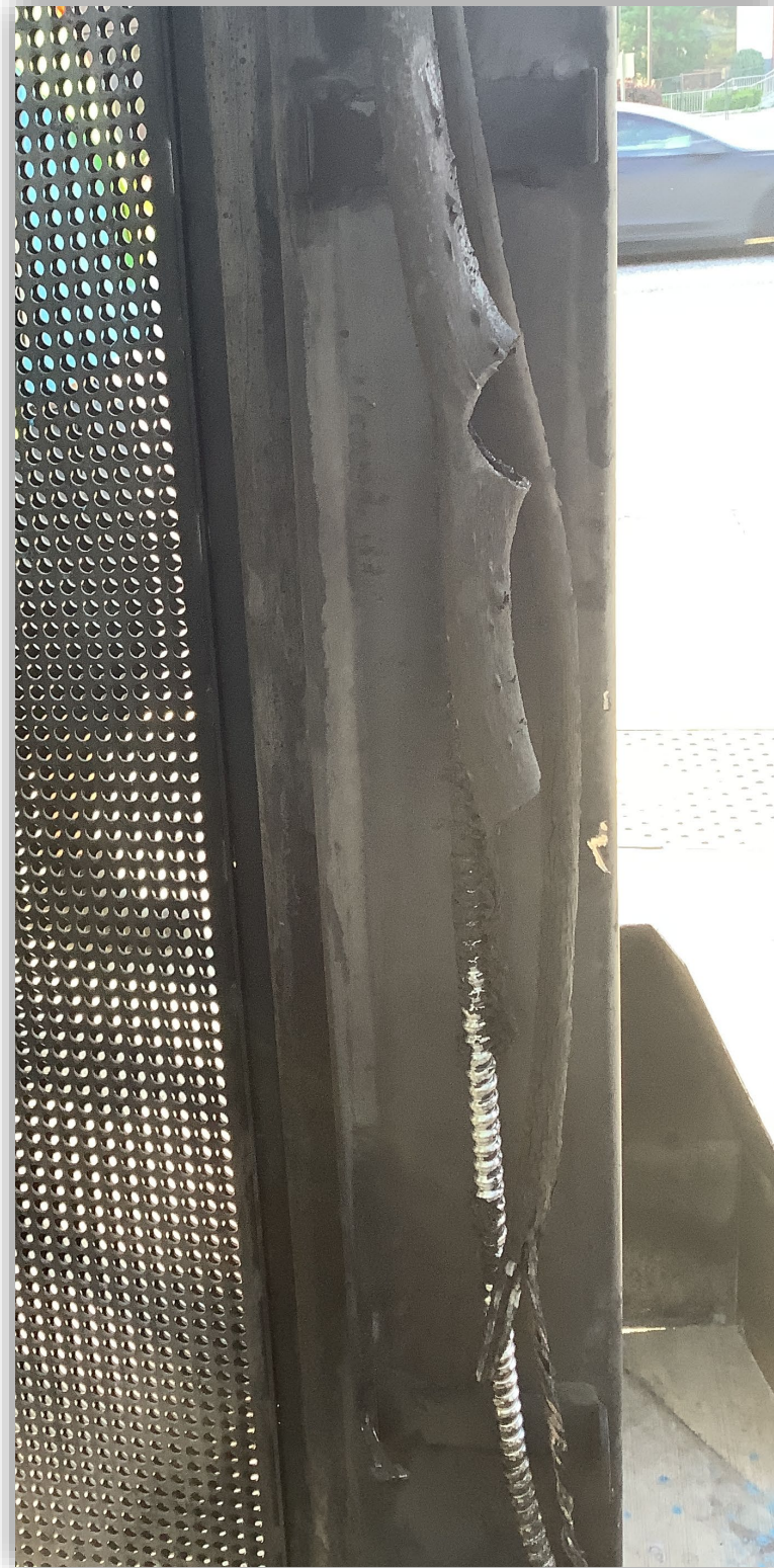
Image 5 - Overview bus shelter; damaged to armoured cable and sheath.
