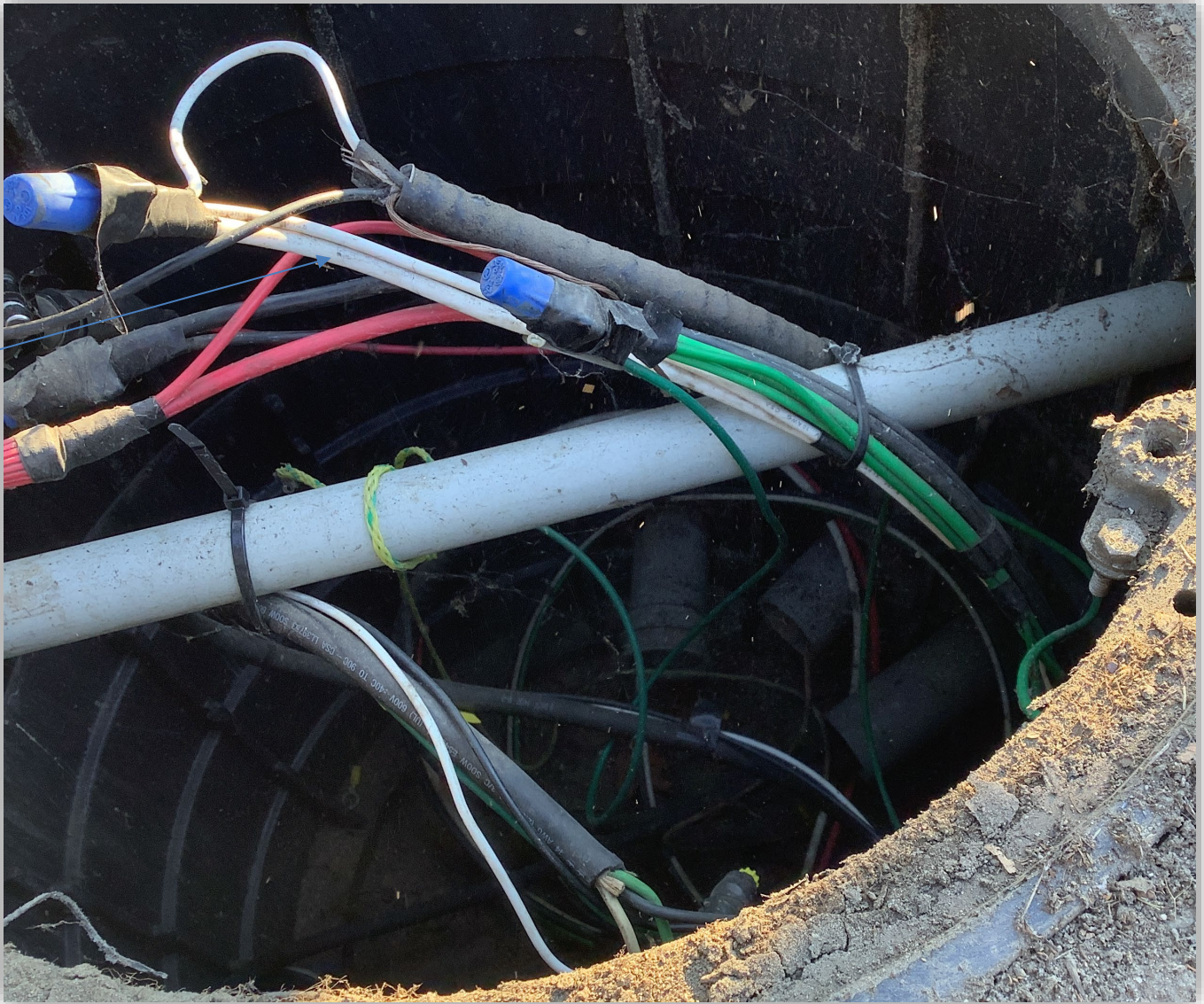
Image 3 - City lighting vault; source voltage connected to flex cable.
