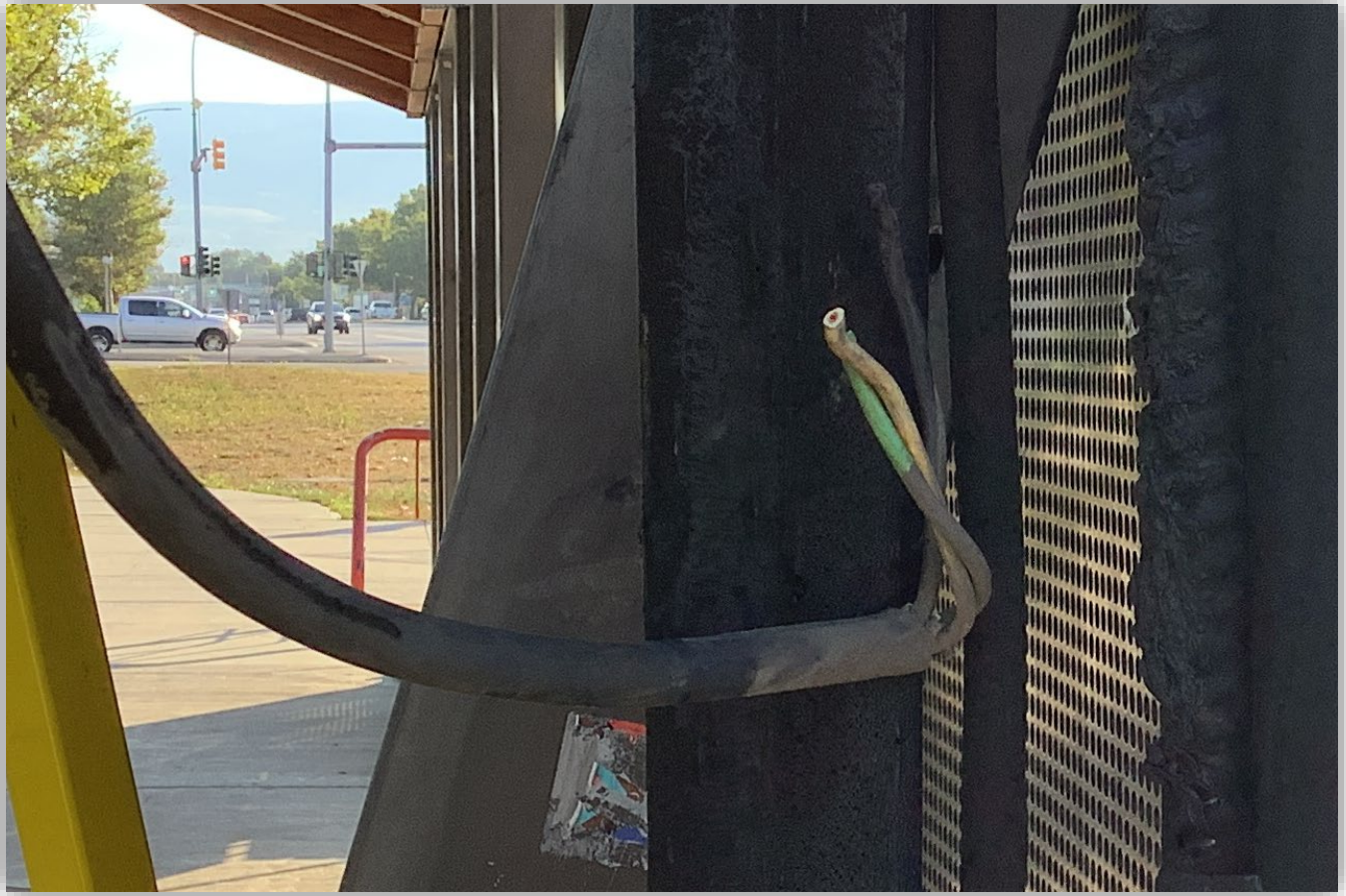
Image 2 - Cable taped off; sign disconnected-Energized from vault (see image 3 -source).
