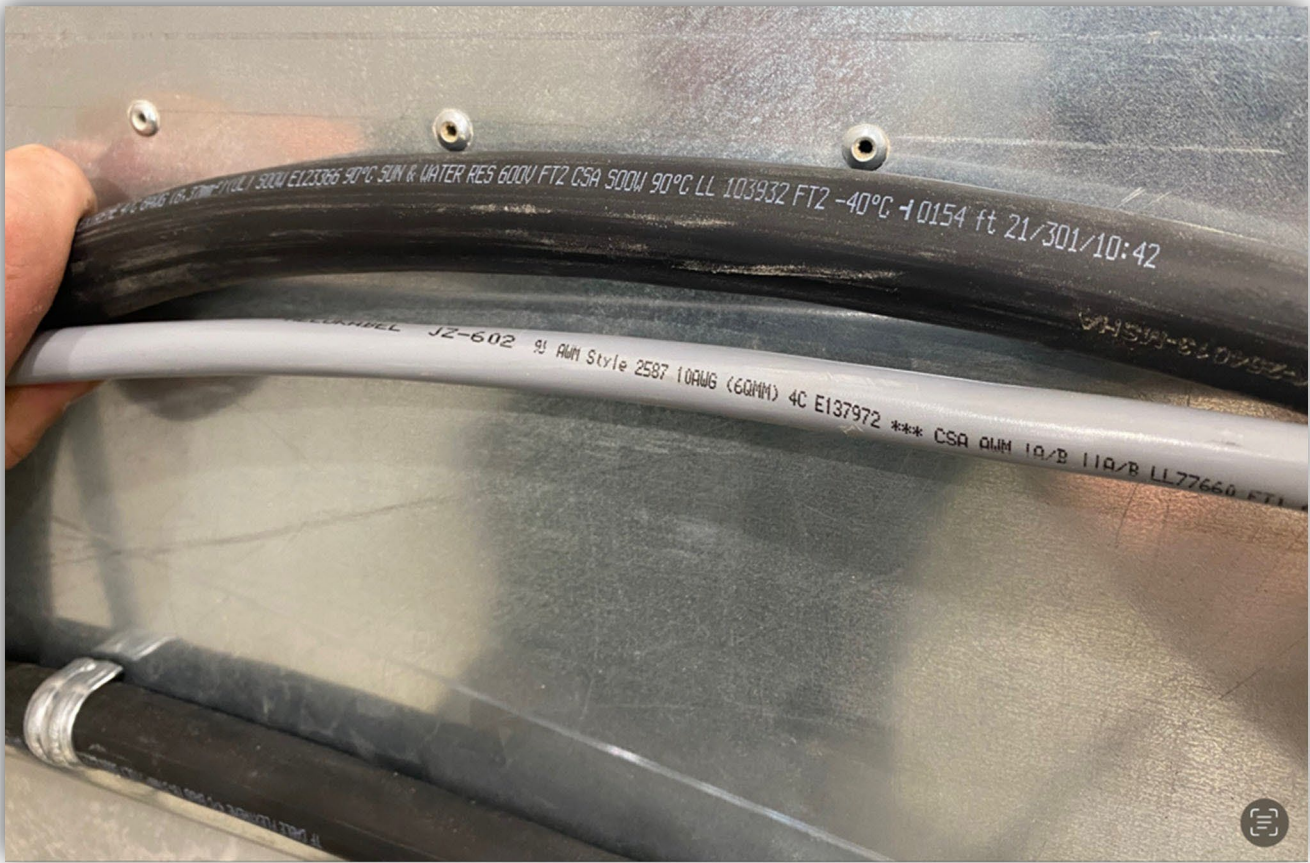
Image 8 – Flexible cables used for connection of the dust collector. The lower cable was a #10 awg type AWM cable that came with the dust collector from the manufacturer. The upper cable was a #8 awg type SOOW flexible cord that was installed on site by an electrical contractor for connection of the dust collector.
