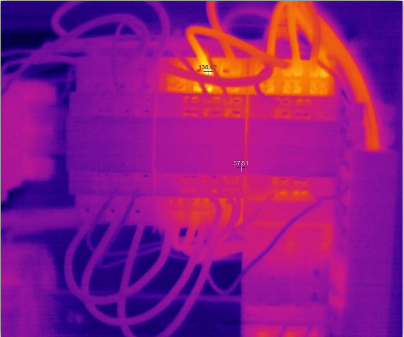
Image 3 - Infrared photograph showing 136 degrees Celsius temperatures measured at the motor conductor terminations at the control contactors within another identical machine at the site.
