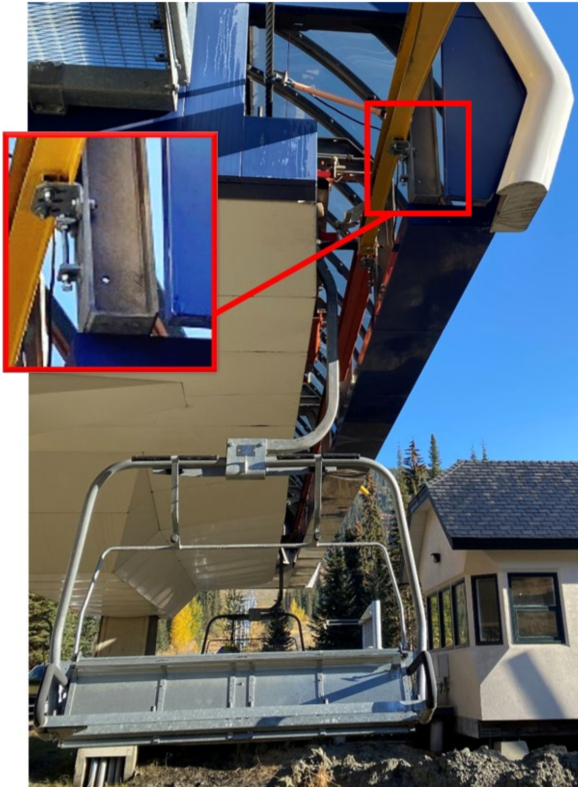
Photo 1 – A typical passenger carrier in the lower station of the lift. [RED] Area the work carrier handrail contacted the station structure when it was reversed into the station.
