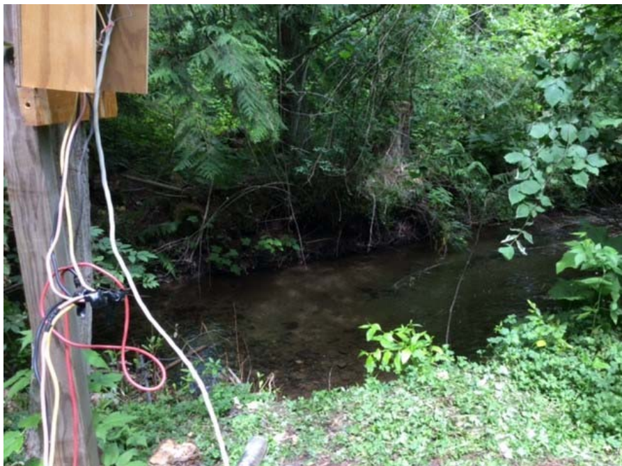
Creek Pump location
