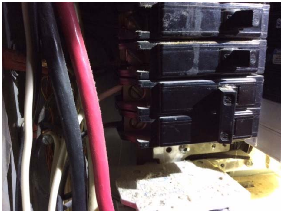
Pump 2P 30 amp residence Overcurrent Device
