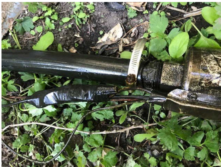
As found splice to motor
