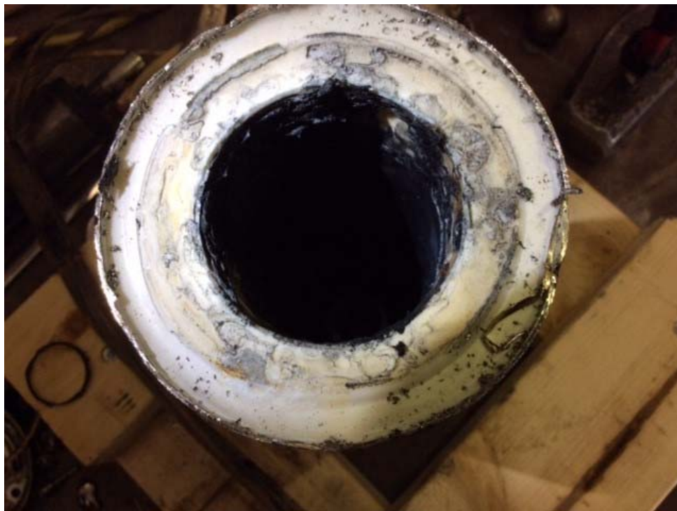
Cut end of stator- damaged noted from rotor jammed at upper right. Windings visible
