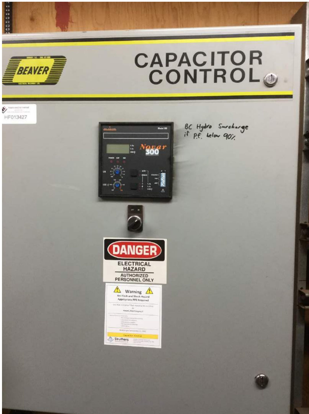
Automatic capacitor control cabinet
