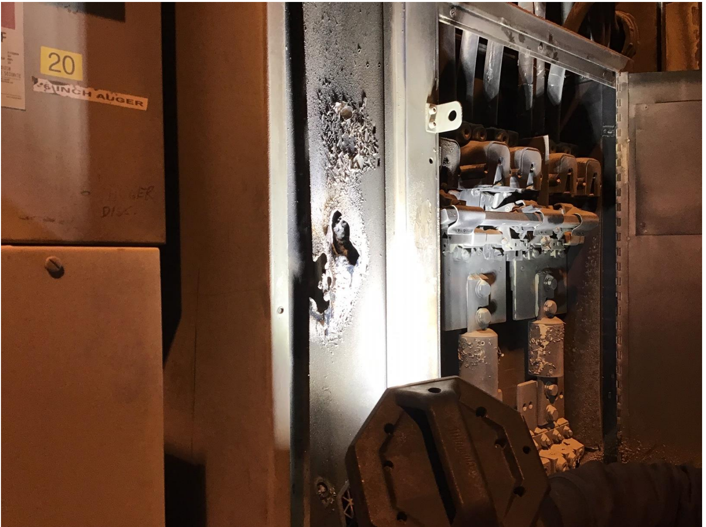
External damage, enclosure perforation
