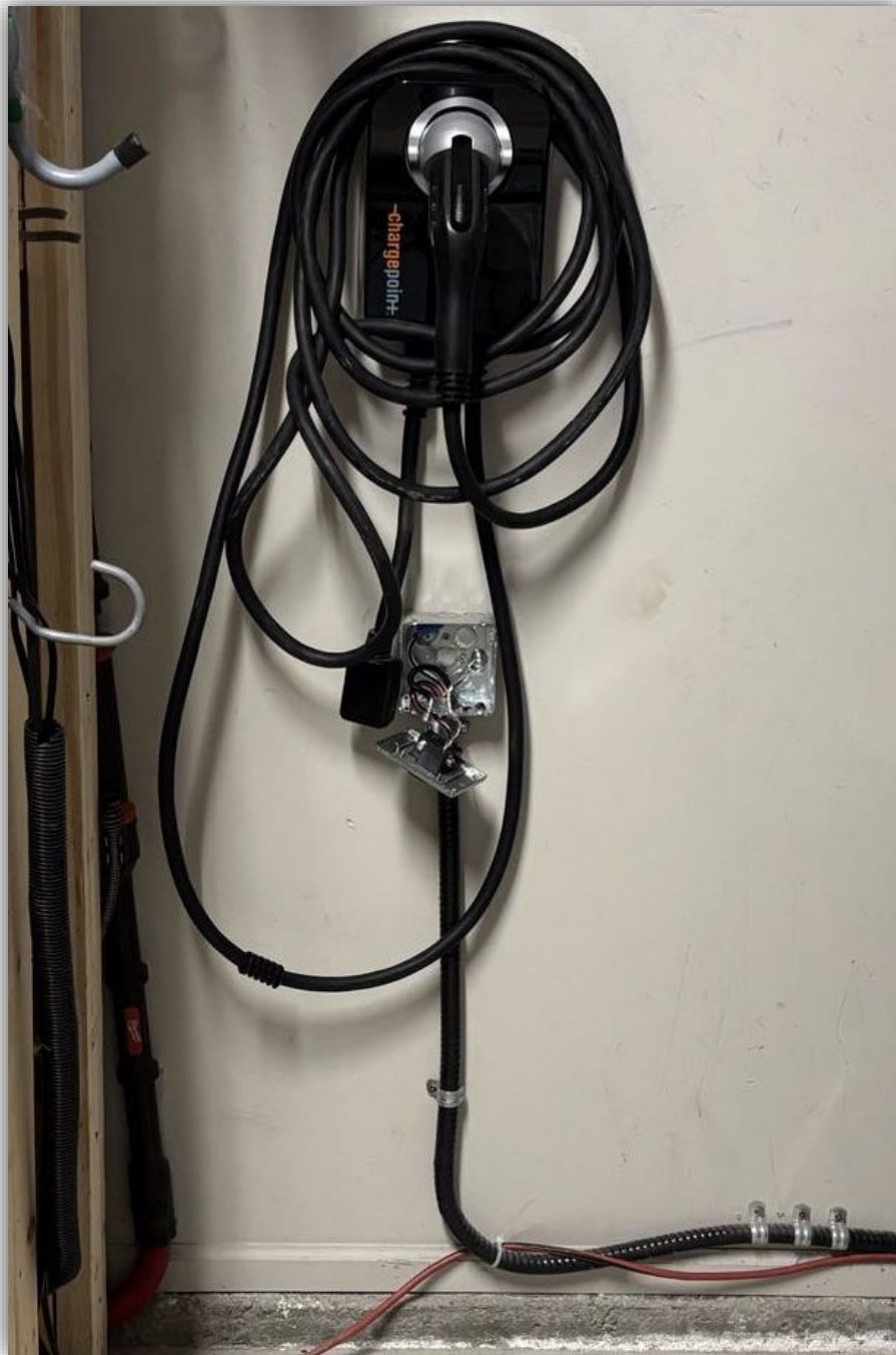
Image 2 – EV ChargePoint charger and plug by receptacle box.
