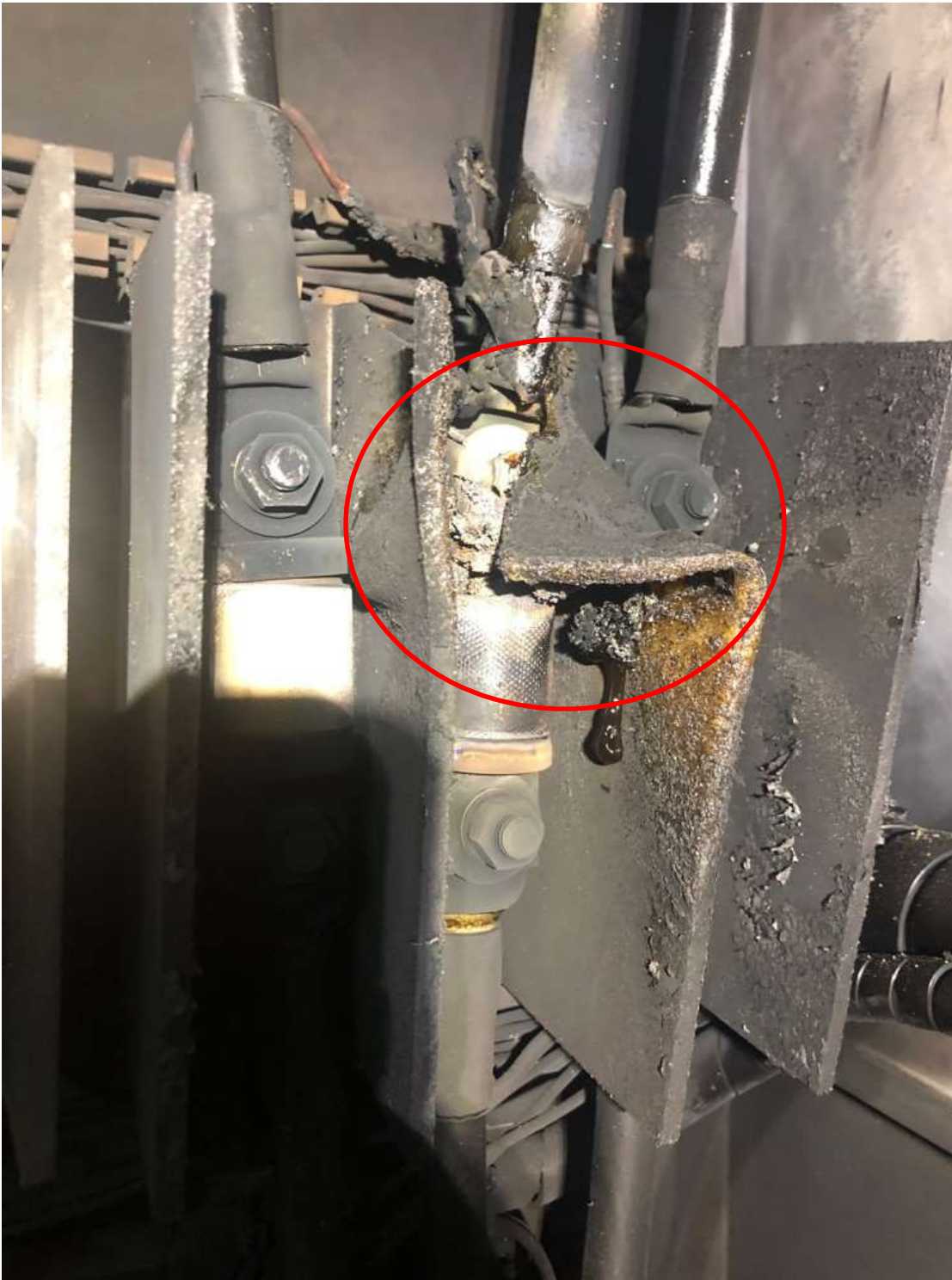
Melted plexiglass divider and termination.
