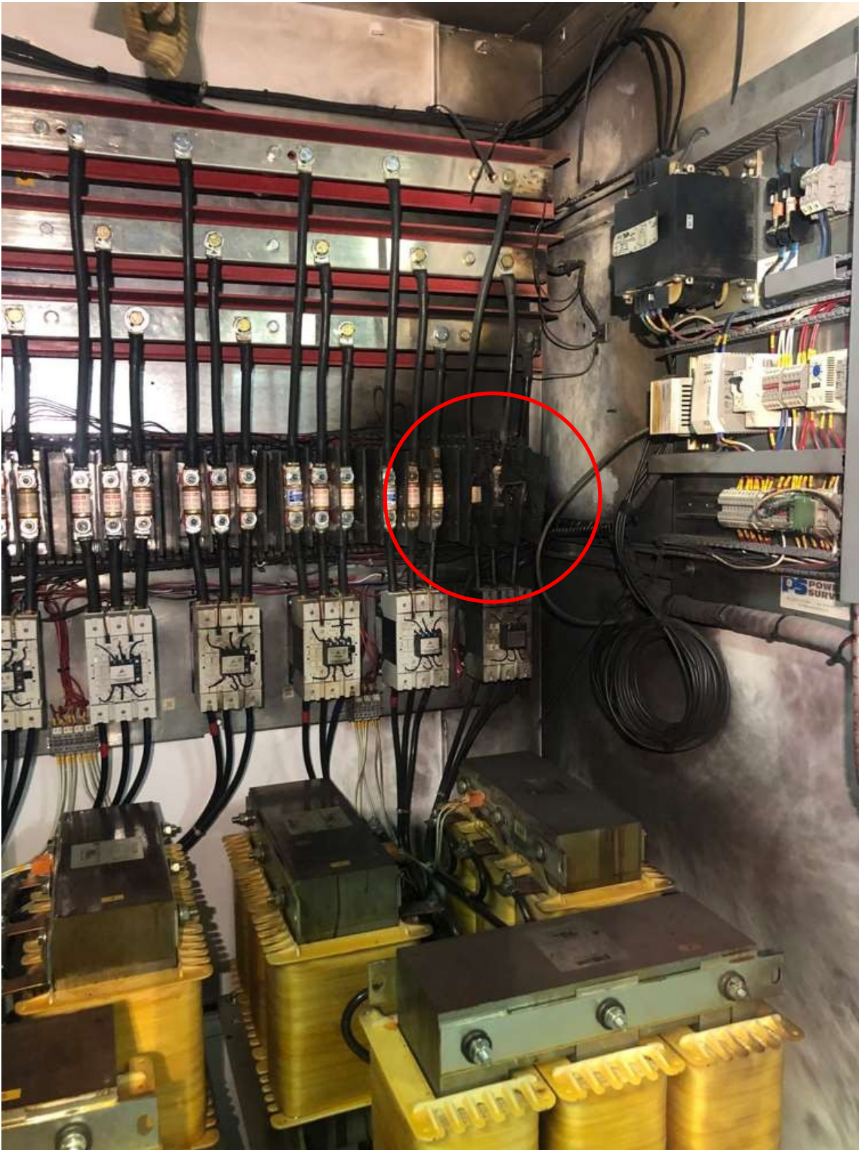
Interior view of damaged capacitor bank.
