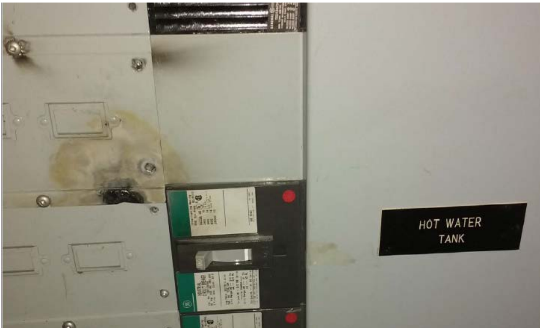
Burn mark on exterior from screwdriver making contact with energized electrical parts and grounded panel-board enclosure
