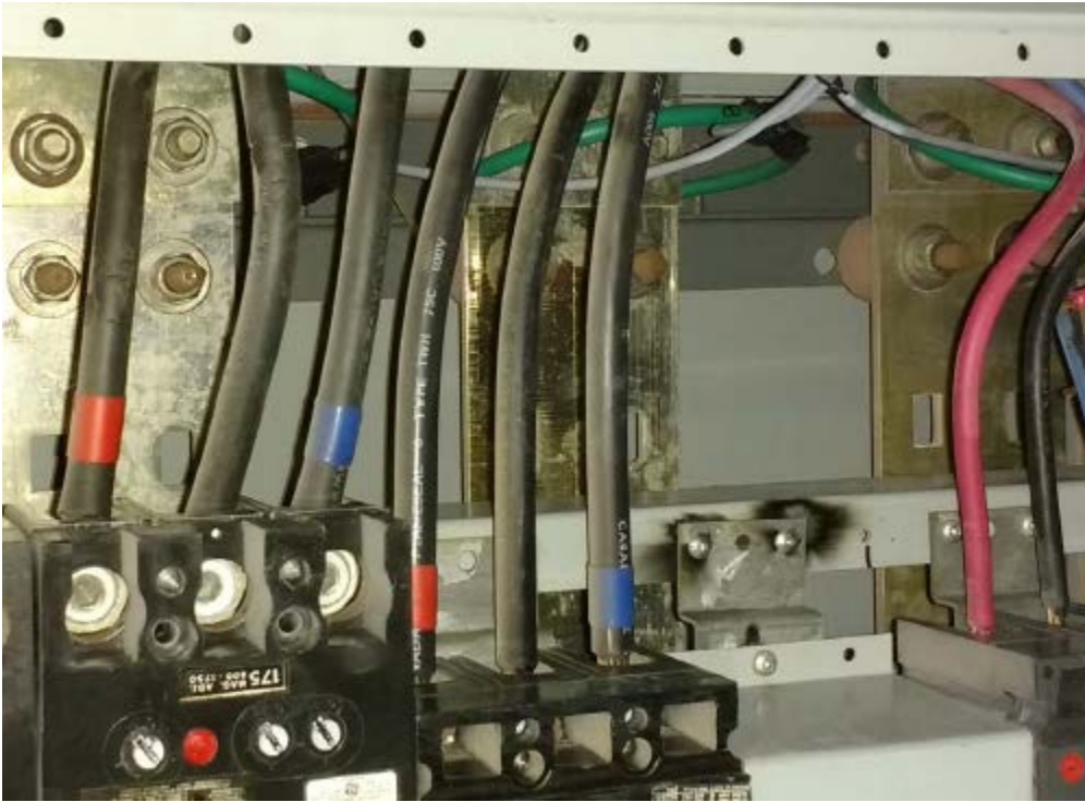
Burn mark on interior of panel-board enclosure
