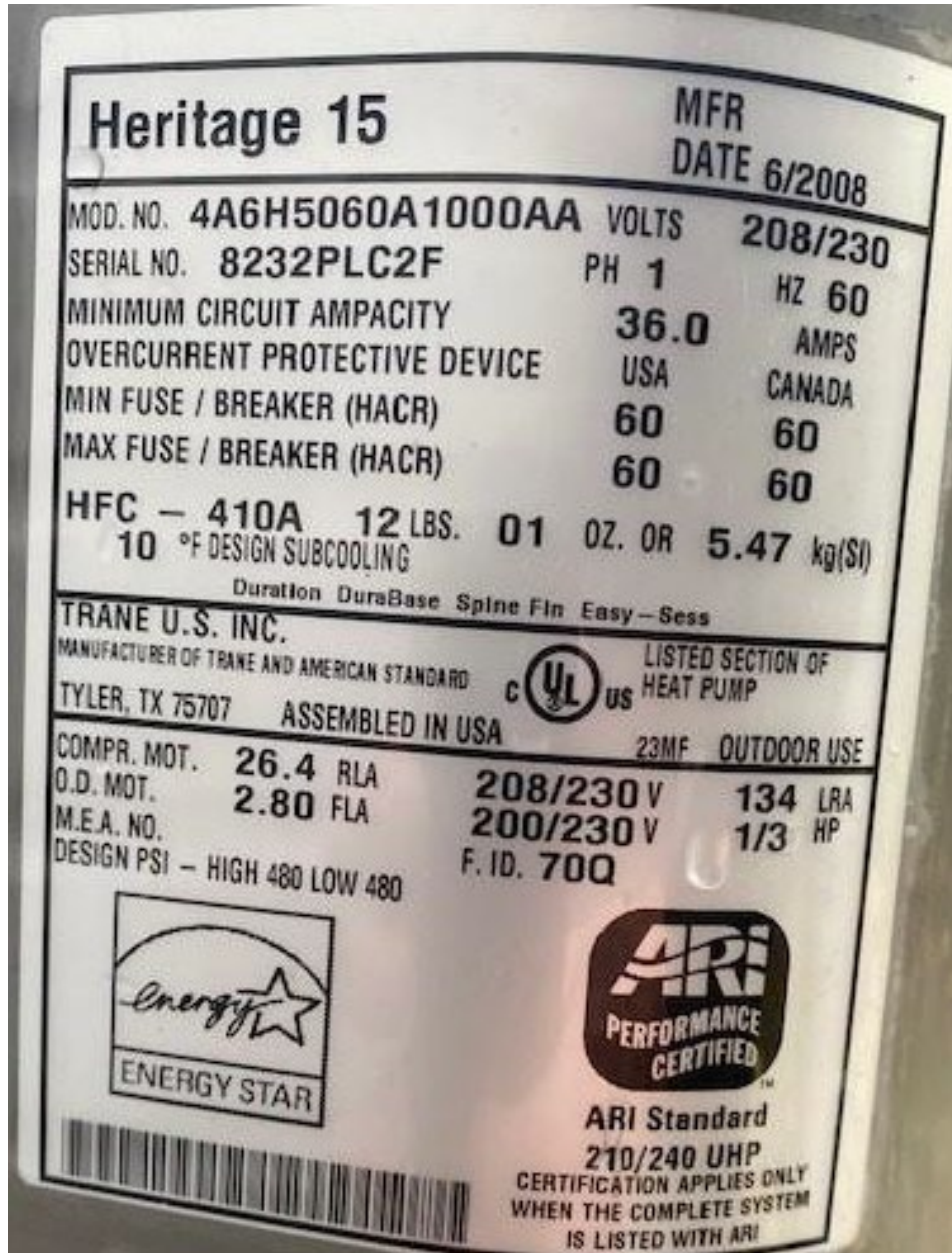
Photo 4 - Heat pump nameplate with breaker size requirement and minimum circuit ampacity
