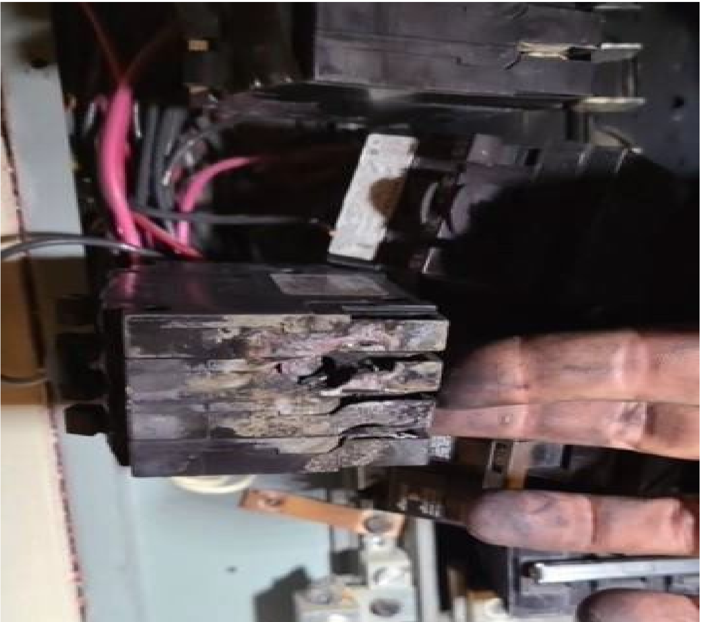
Photo 3 - Quad 2 pole 40-Amp heat pump breaker
