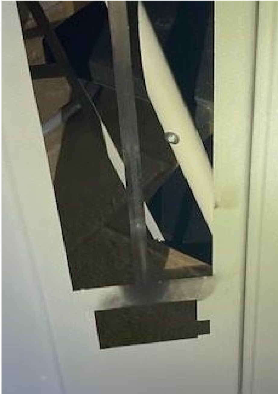
Photo 2 - Back side of cover from distribution panel with smoke damage
