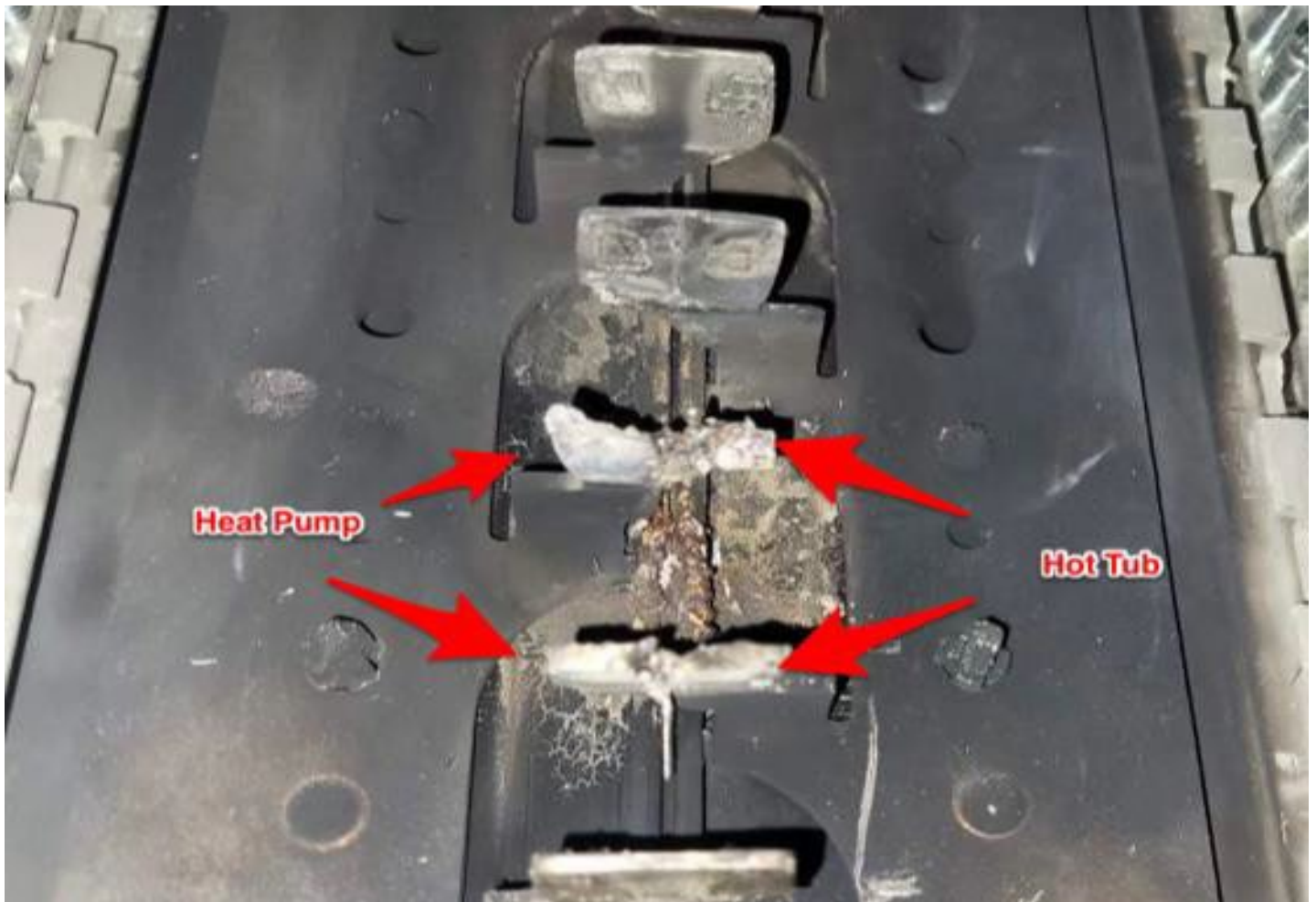
Photo 5 - Location of Heat pump and Hot tub breakers on main buss
