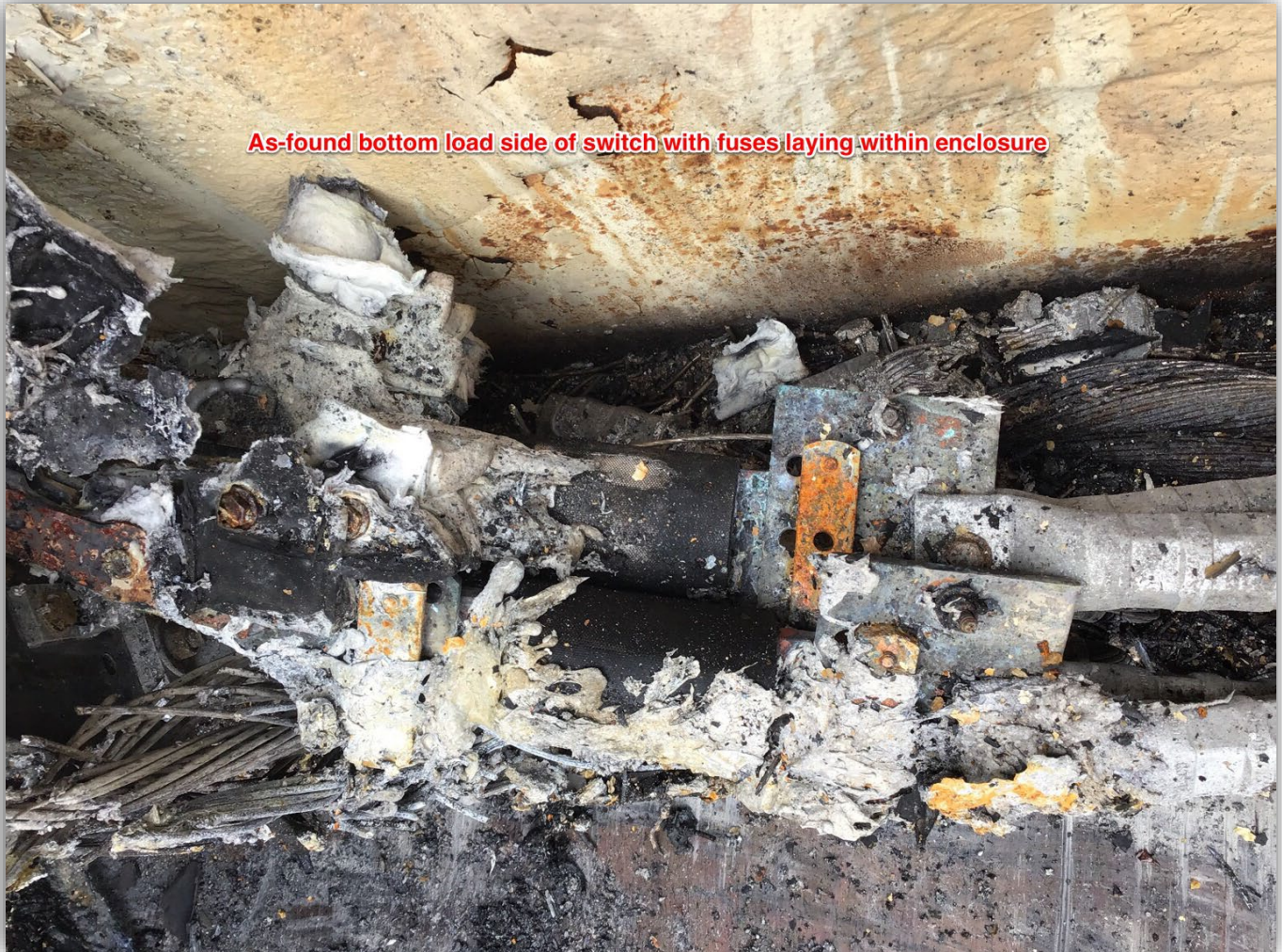
Image 7 – As-found view of fuses laying in bottom of 800amp main fused disconnect switch.
