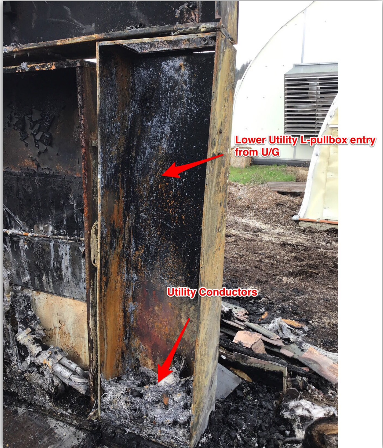
Image 11 – Utility 'L' Pull-box vertical section. This section provides cable mounting blocks for utility to support incoming underground conductors from utility pad mount transformer.
