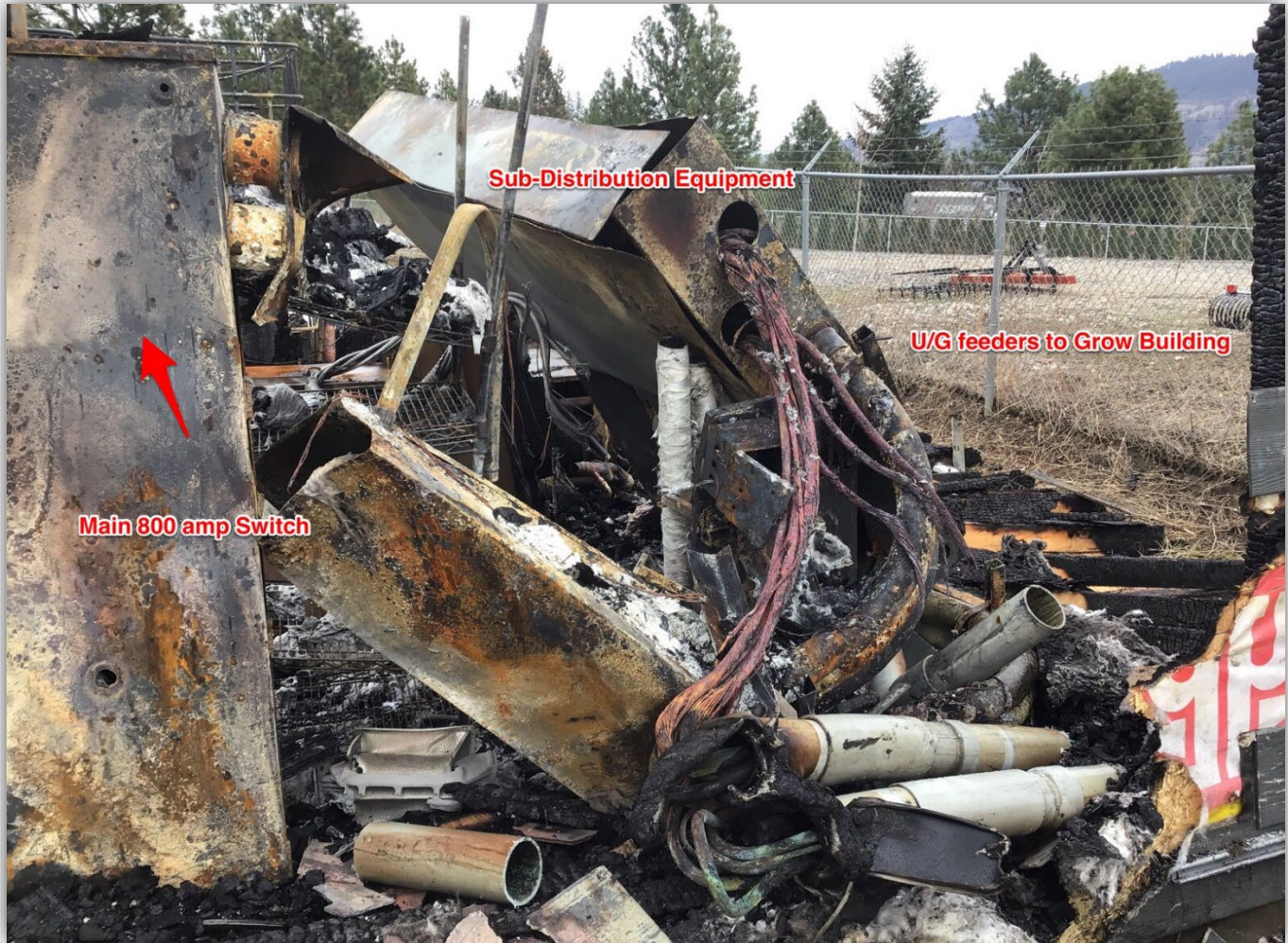
Image 14 – View from outside of the electrical room building on the westside, showing the damage to the sub-distribution equipment, the existing splitter and feeder conductors. Main 800amp fused disconnect switch viewed on left, and utility CT cabinet at lower mid area fell during fire.
