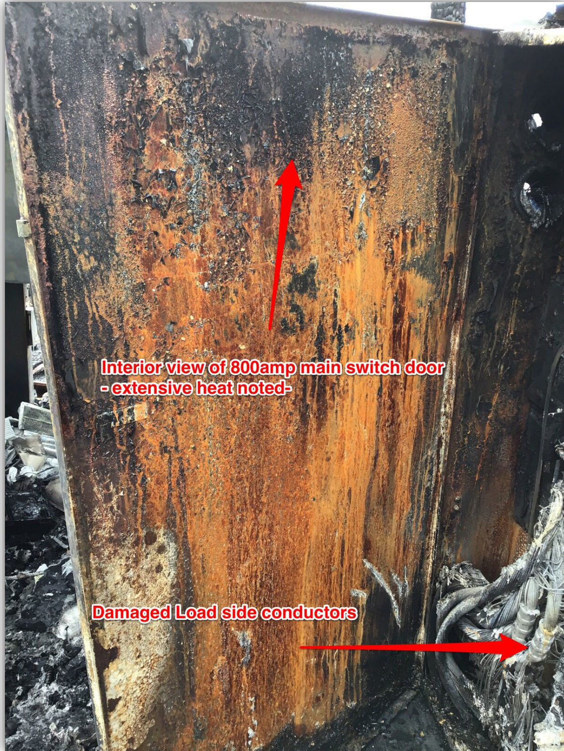
Image 6 – Interior view of 800amp main fused disconnect door providing evidence of arc-faulting occurring within main switch.
