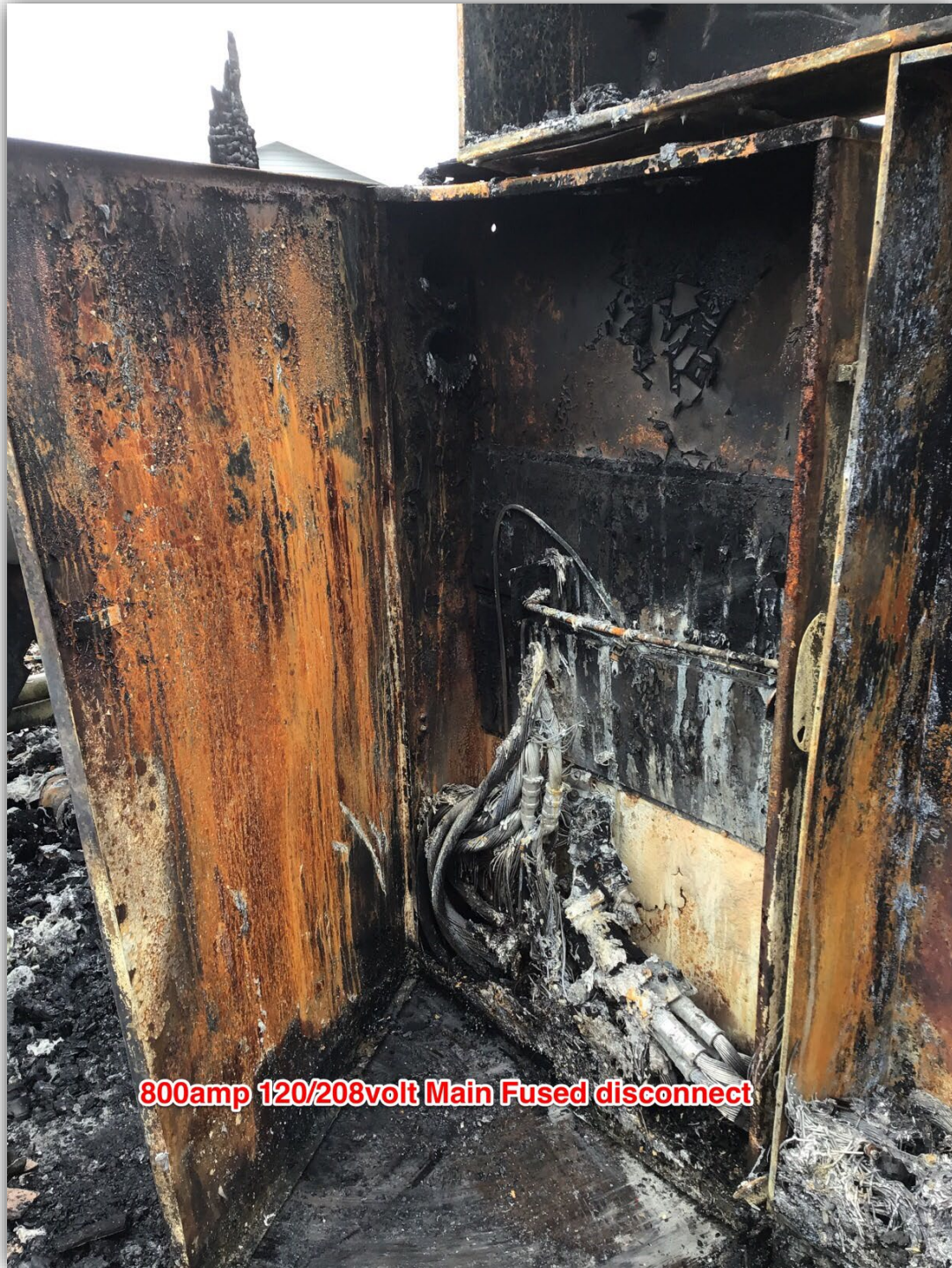
Image 4 – Interior of the 800amp fused disconnect switch, with the load side fusing laying in bottom with lugs still attached, all line side operating hardware mechanisms, and all conductors are destroyed.
