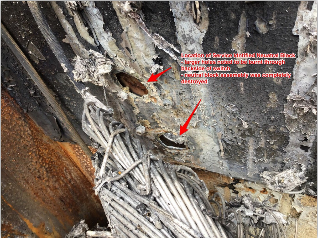
Image 9 – Interior view of main 800amp fused disconnect switch and the location where neutral block would be installed. Excessive heat noted with melting of metal enclosure noted.
