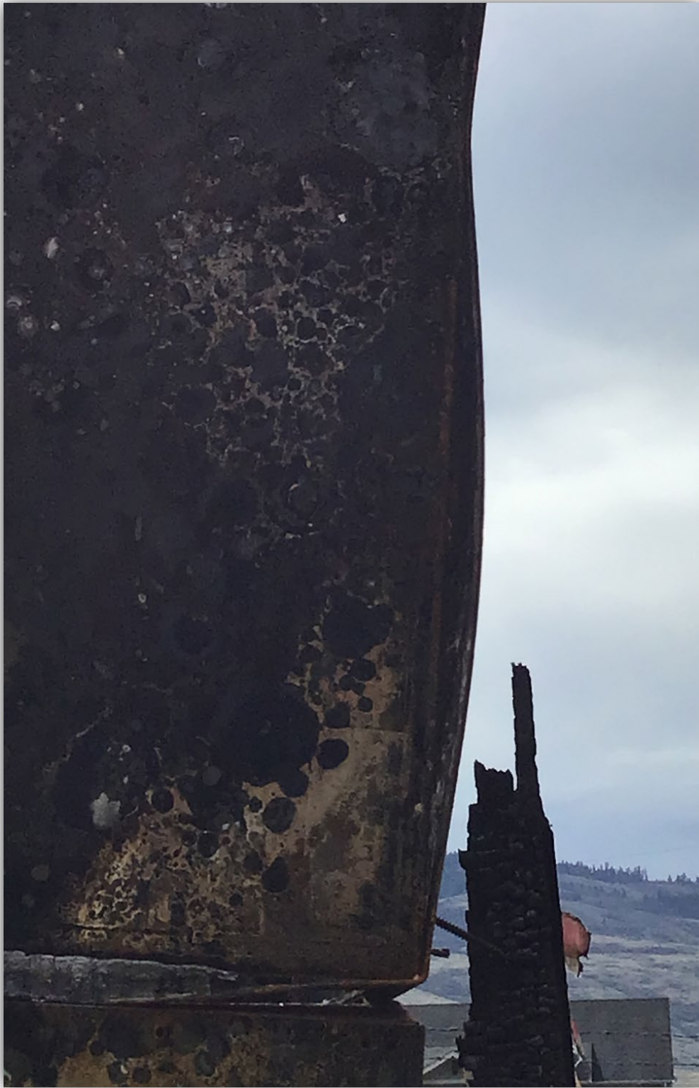
Image 12 – Backside edge view of upper utility pull-box showing signs of deformation from interior fault allowing excessive arcing to release from cabinet. Intense heat within utility L-pull box deformed joints, creating openings for heat/sparks/flames to escape to combustible walls.
