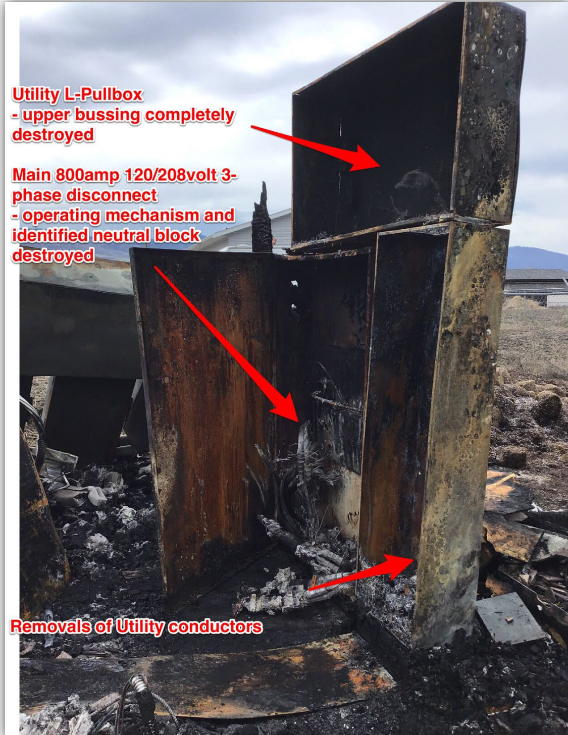
Image 3 – Main Service entrance equipment:
