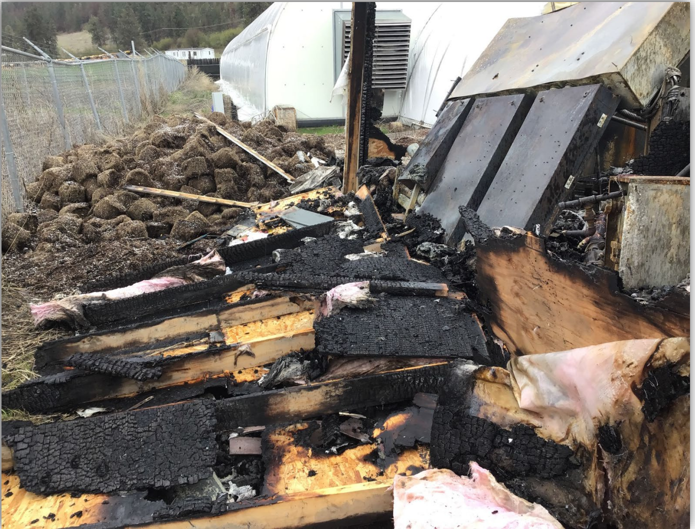
Image 15 – South backside exterior wall of electrical room that sub-distribution was secured to laying on ground with studs and sheathing showing fire damage with areas not burnt.
