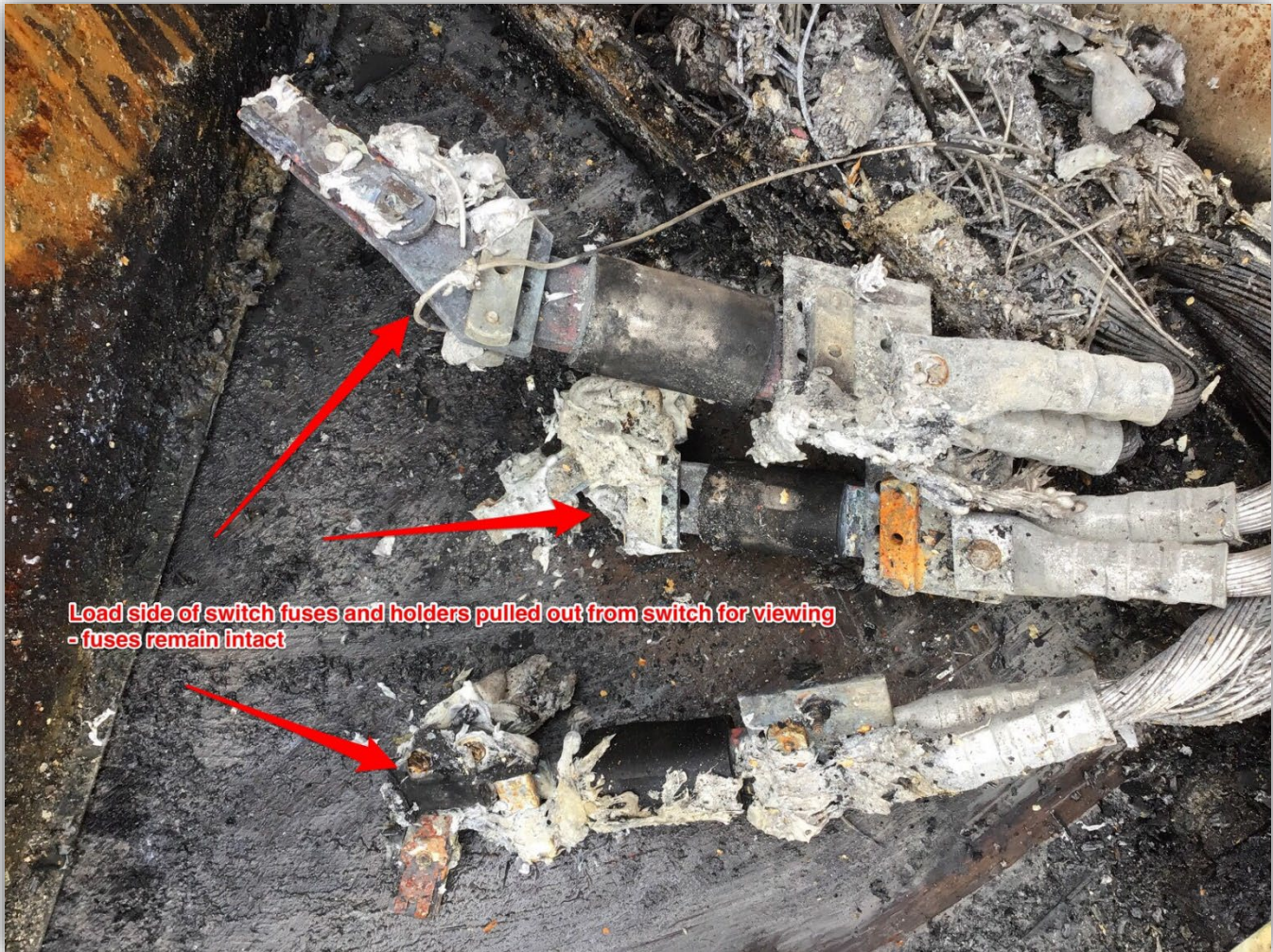
Image 8 – Main 800amp fuses pulled out from disconnect for viewing noting damaged load side fuses/connections remain with partial pieces of switching hardware connect to line side.
