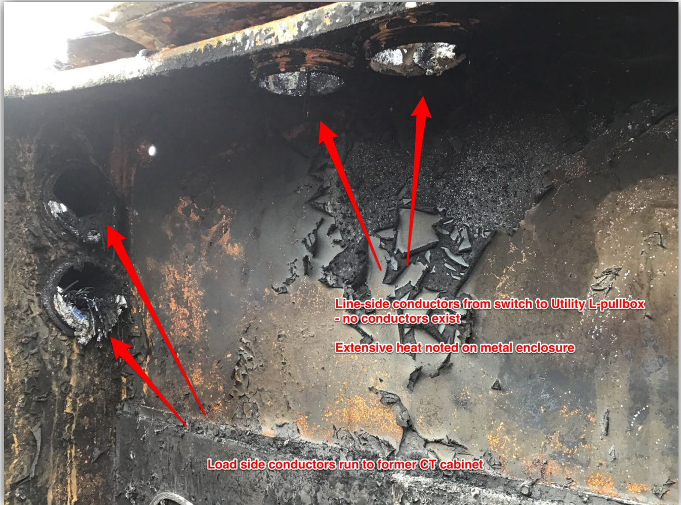
Image 5 – Main Upper interior view of 800amp main fused disconnect switch, all conductors are destroyed, evidence of excessive interior arc-faulting occurrence.
