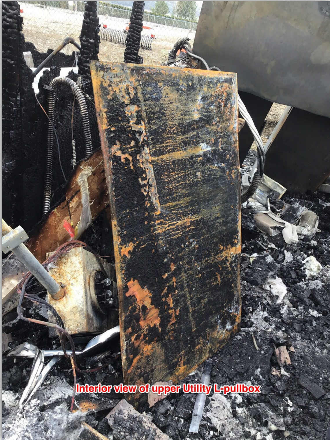
Image 13 – View of interior of upper utility pull box showing excessive interior electrical faulting.
