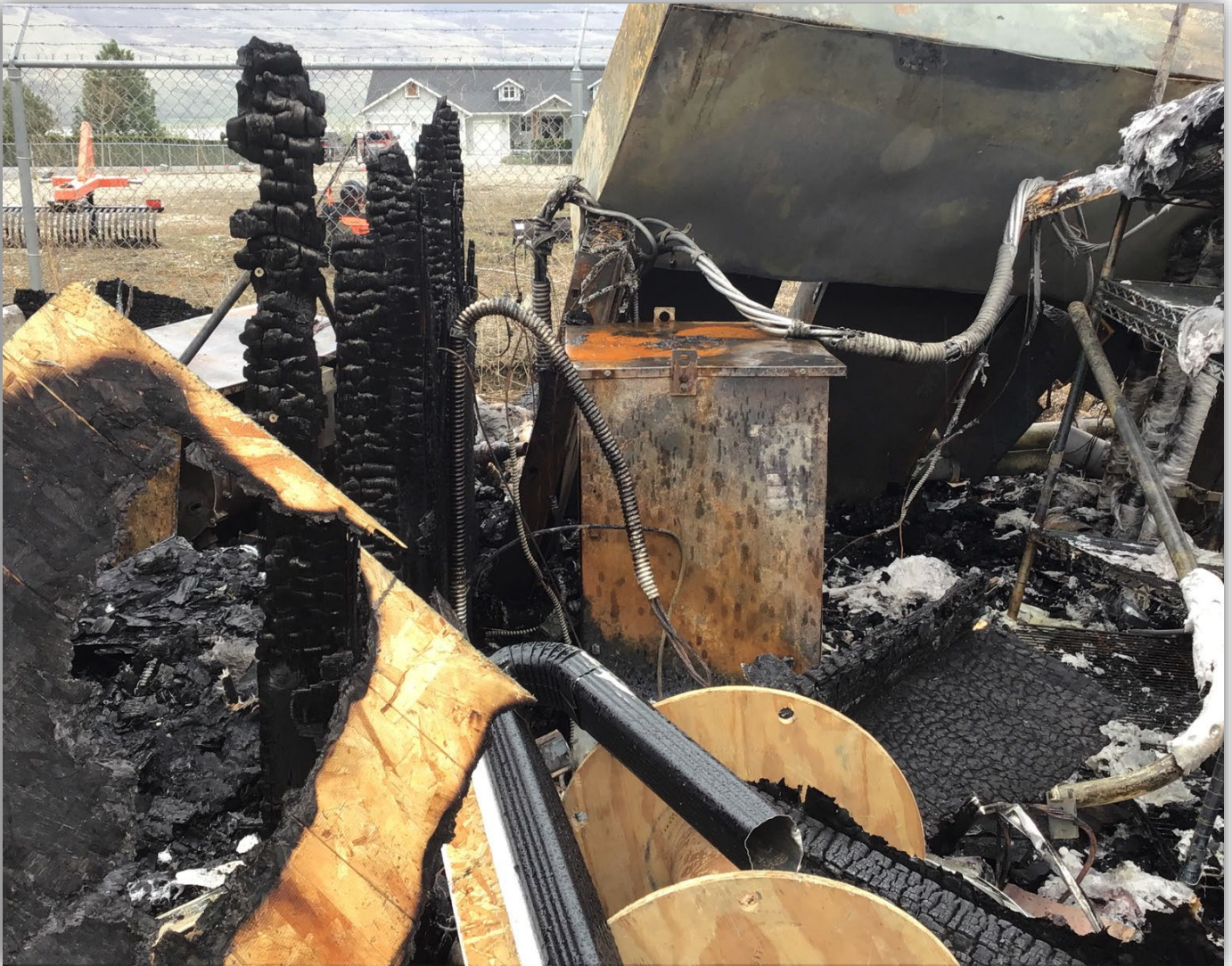
Image 16 – Internal view of electrical room looking south note burnt studs to left standing which was the separation wall between electrical and mechanical areas of the structure.
