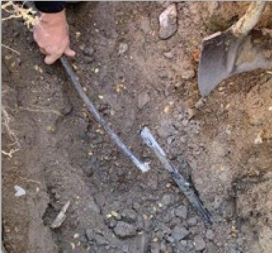
Image 3 – Location where cable was once joined.
