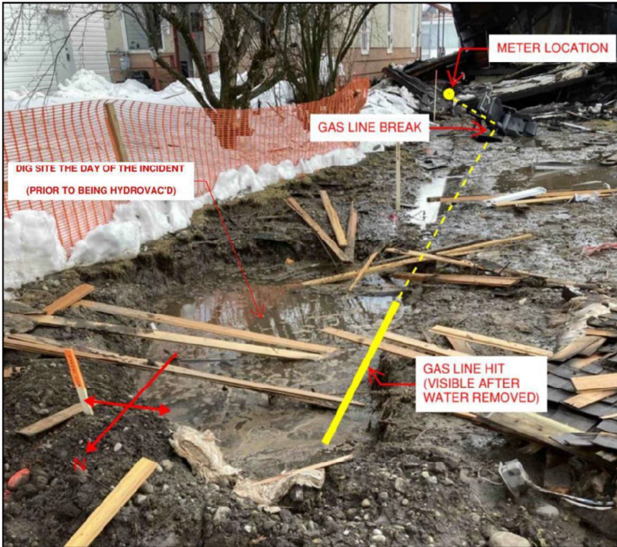
Figure 5 - Dig / Excavation Area after the NG Explosion (prior to Hydrovac)
