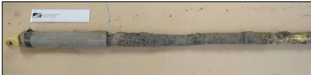
Figure 16 - 3/4" steel to 1/2" PE Transition Fitting from the Subject Property
