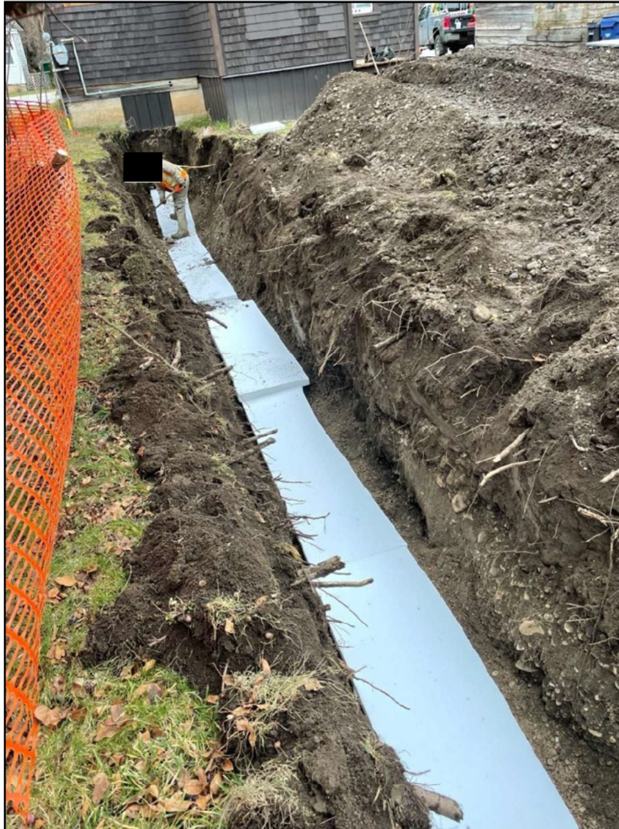
Figure 2 - New Water Service and Sanitary Line Trench (assume ~5.0 ft deep) prior to the NG Explosion
