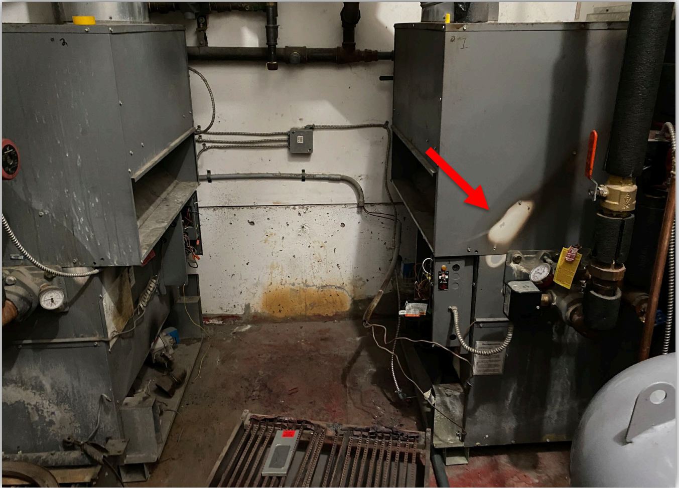
Image 1 - Scene when Safety Officer arrived on site. Arrow indicates hot spot found on side of boiler.
