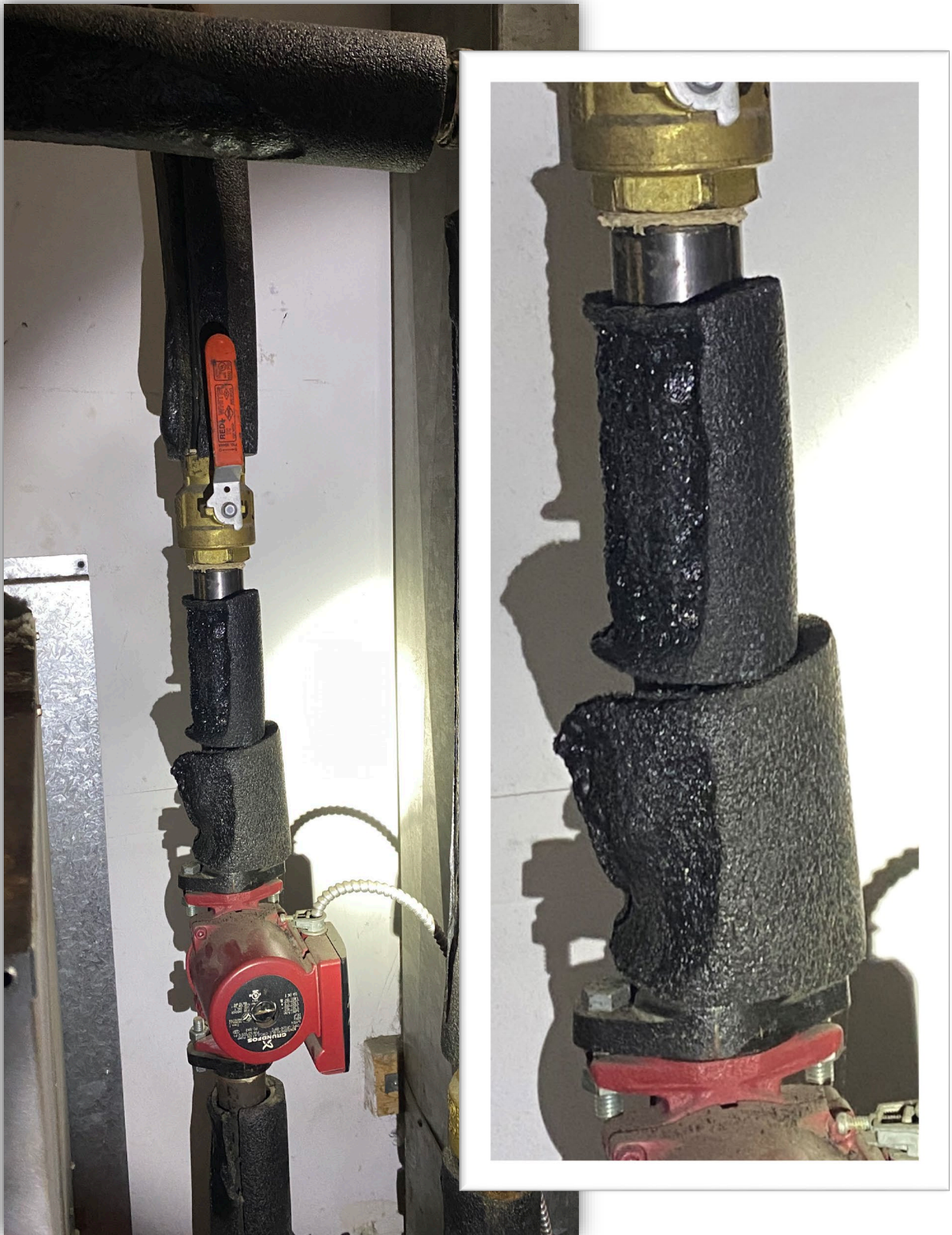
Image 14 - Boiler piping insulation, melted from heat radiated by hot spots on boiler sheet metal.
