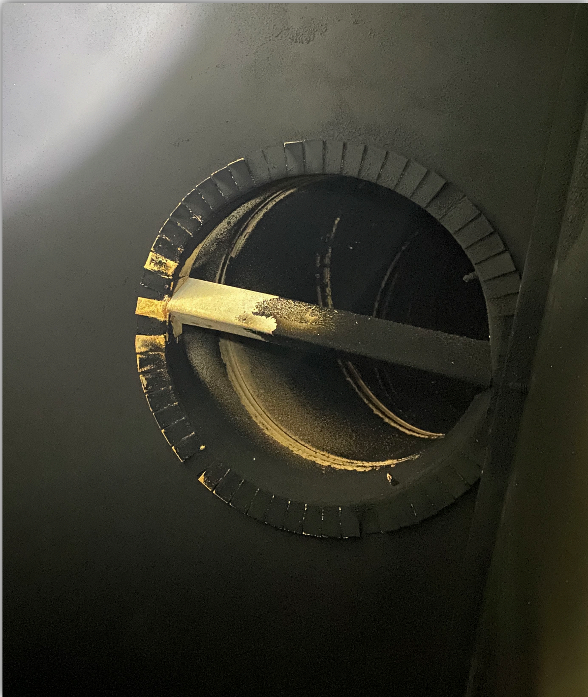
Image 12 - Boiler breeching where vent connects to the boiler showing signs of heavy sooting due to poor combustion.
