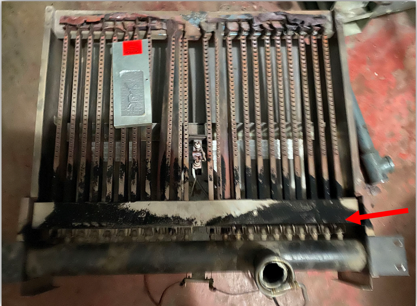
Image 8 - Boiler burner tray showing sooting from poor combustion. Arrow indicates burner orifice where flames exiting the boiler are believed to have come from.
