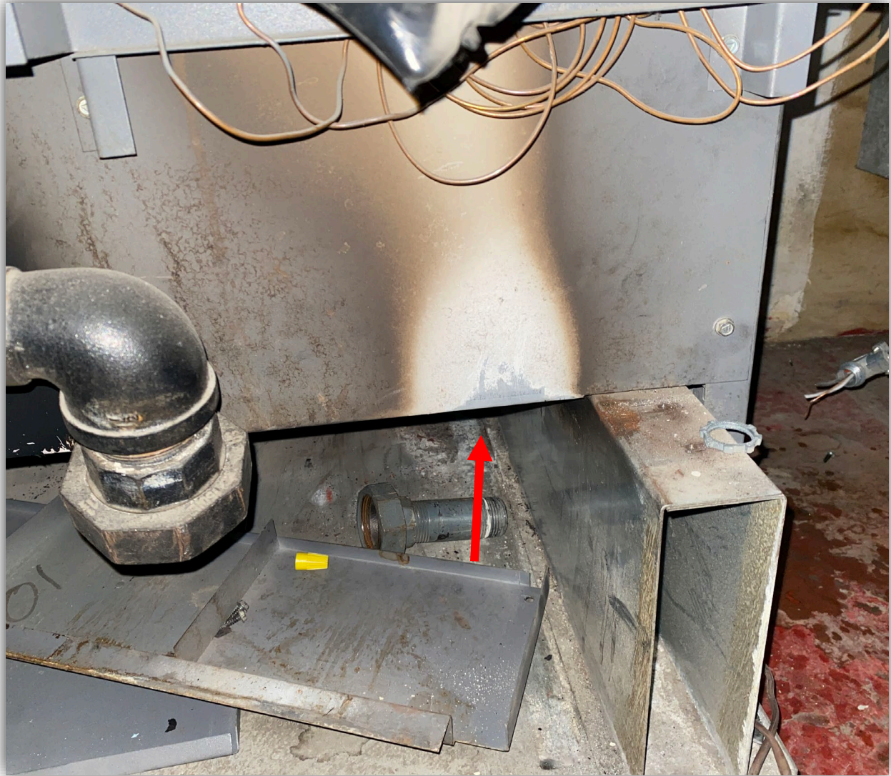
Image 5 - Boiler combustion chamber showing burn path where flames were found exiting the boiler.
