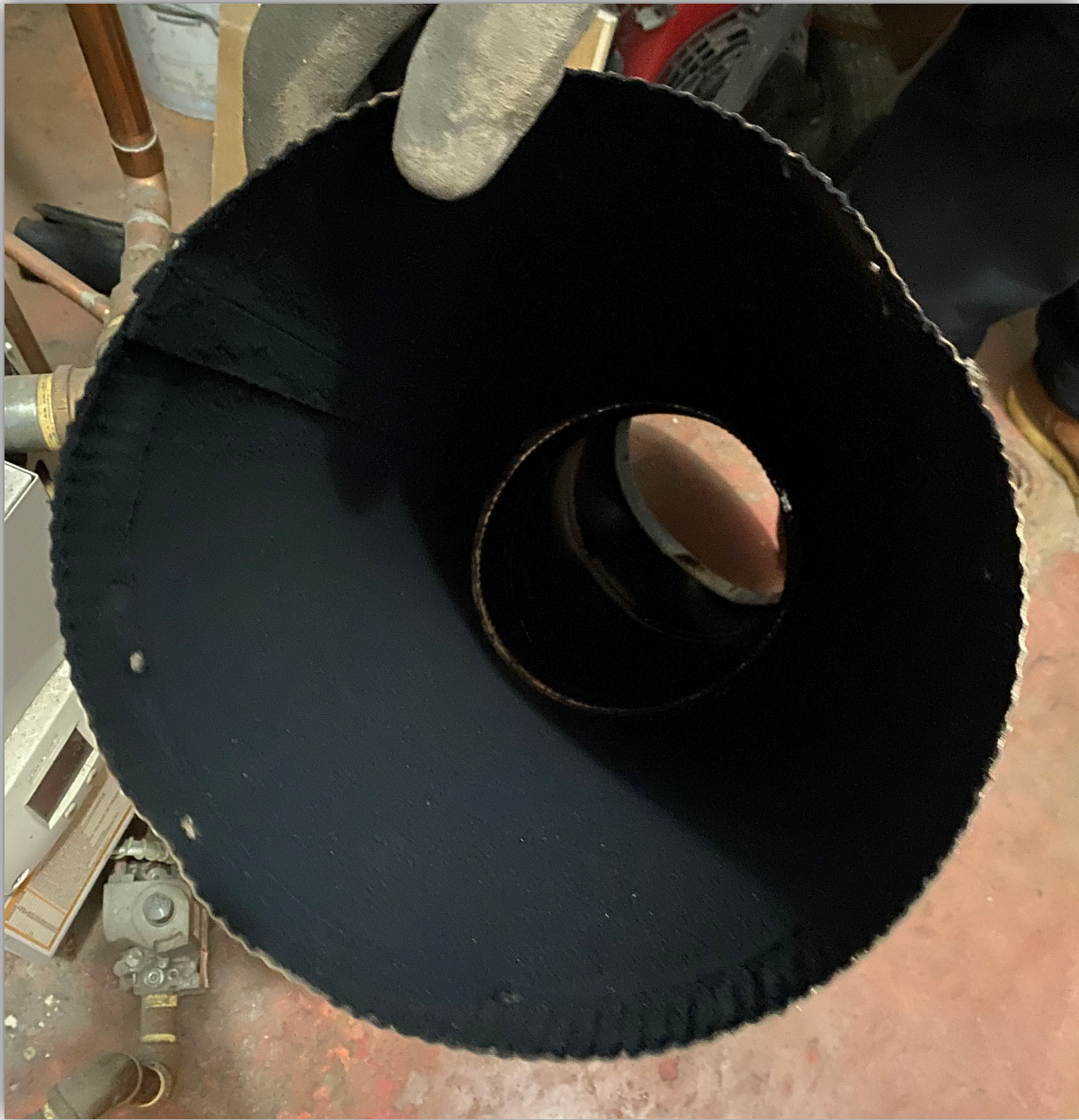
Image 13 - Interior of boiler venting showing heavy sooting due to poor combustion.
