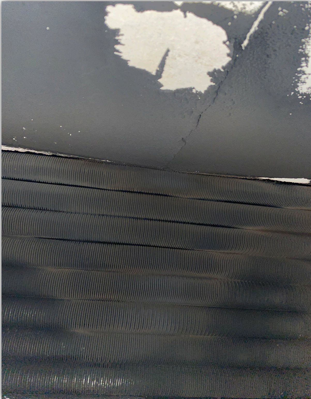
Image 10 - Underside of heat exchanger showing visible sooting and plugging.
