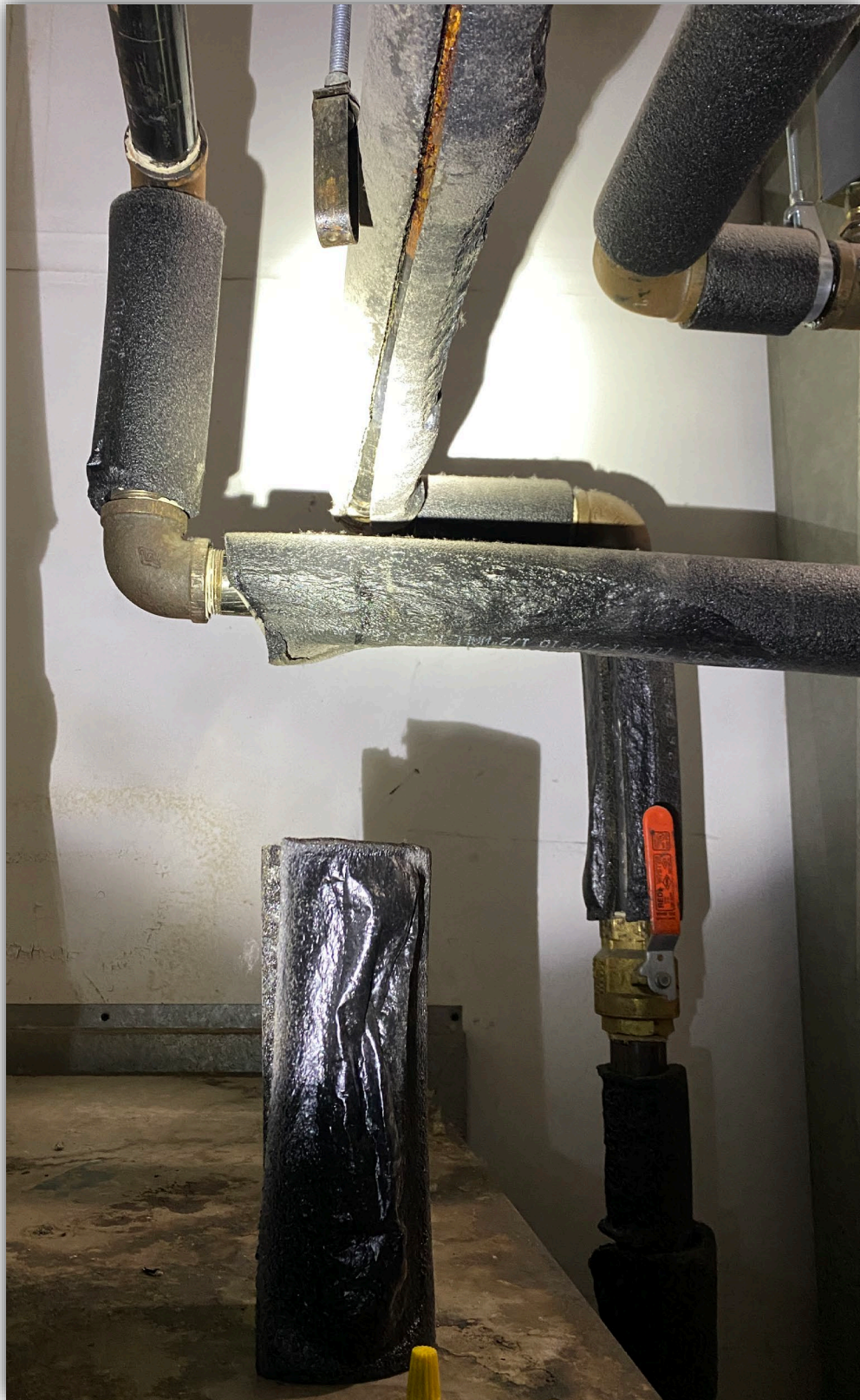
Image 15 - Boiler piping insulation melted by heat radiated from hot spots on boiler sheet metal.
