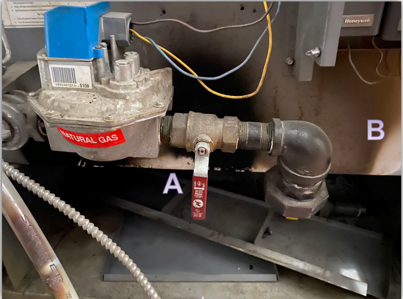
Image 4 - Boiler gas valve and combustion chamber at time of investigation. [A] Area where flame rollout was occurring. [B] Area where flames were seen exiting boiler.
