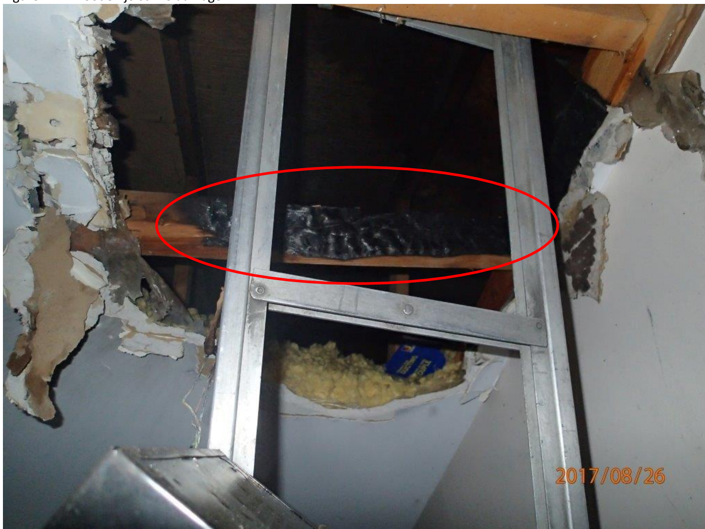
Figure #2 – Wooden joist fire damage
