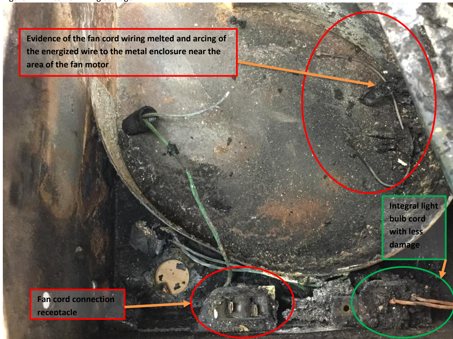
Figure #1 – Internal wiring damage
