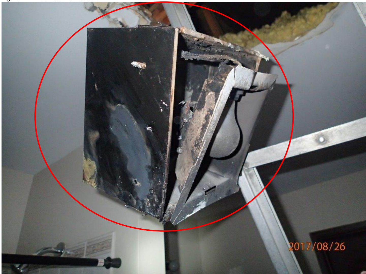
Figure #1 – Bathroom exhaust fan
