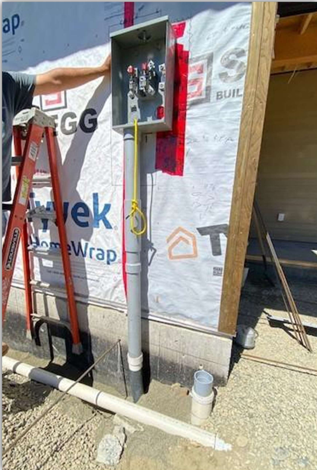
Image - Location where the hammer drill contacted the consumer service cable in the foundation wall. (Rebar was inserted into the hole left of the 3" PVC for ease of viewing).
