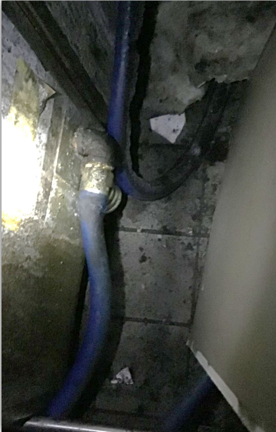
Image 2 - Cable restraint located on rear of fryer bank.
